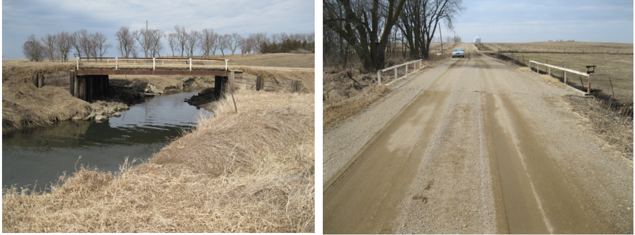
Figure B-58. Steel-Timber Bridge 8: South elevation view (left) and west end view (right)
