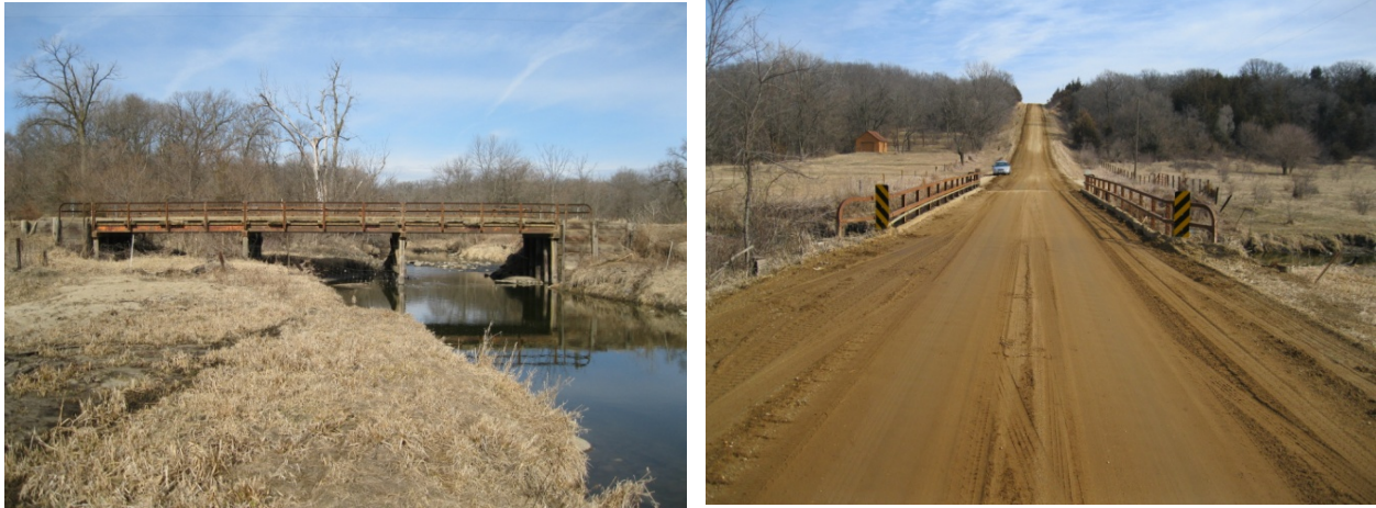
Figure B-81. Steel-Timber Bridge 11: South elevation view (left) and east end view (right)
