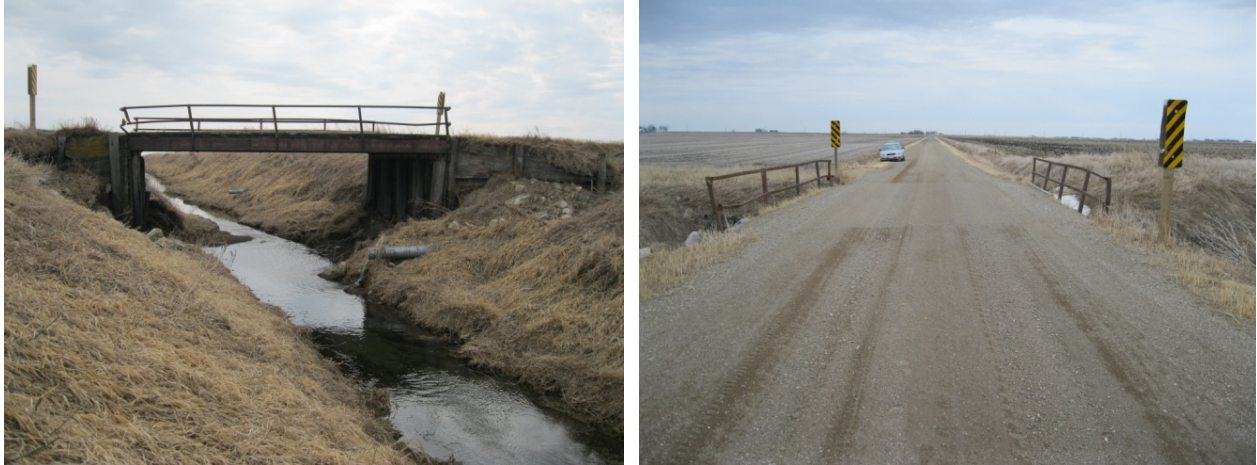
Figure B-65. Steel-Timber Bridge 9: North elevation view (left) and east end view (right)
