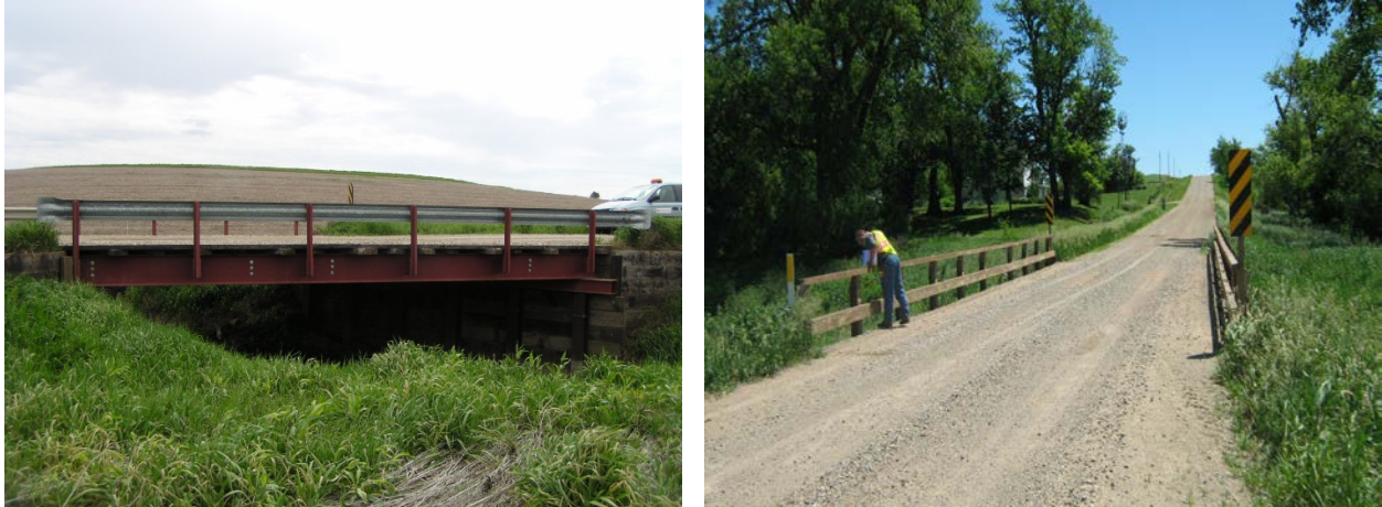
Figure B-42. Steel-Timber Bridge 6: North elevation view (left) and east end view (right)
