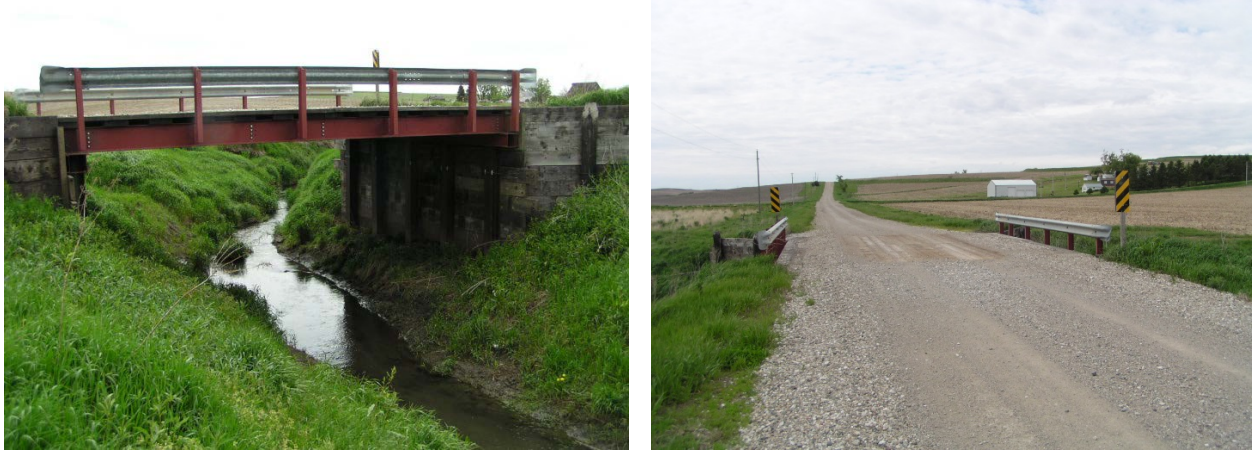
Figure B-2. Steel-Timber Bridge 1: West elevation view (left) and north end view (right)
