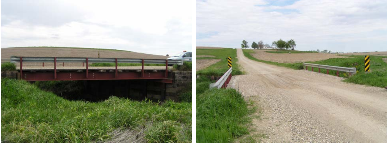
Figure B-10. Steel-Timber Bridge 2: South elevation view (left) and west end view (right)
