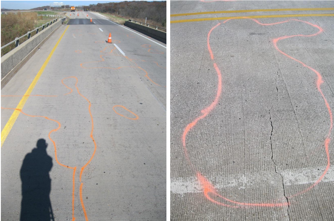
Figure 3.4. Photographic documentation of delamination
