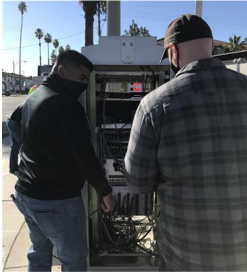
(a) At Traffic Controller Cabinet
