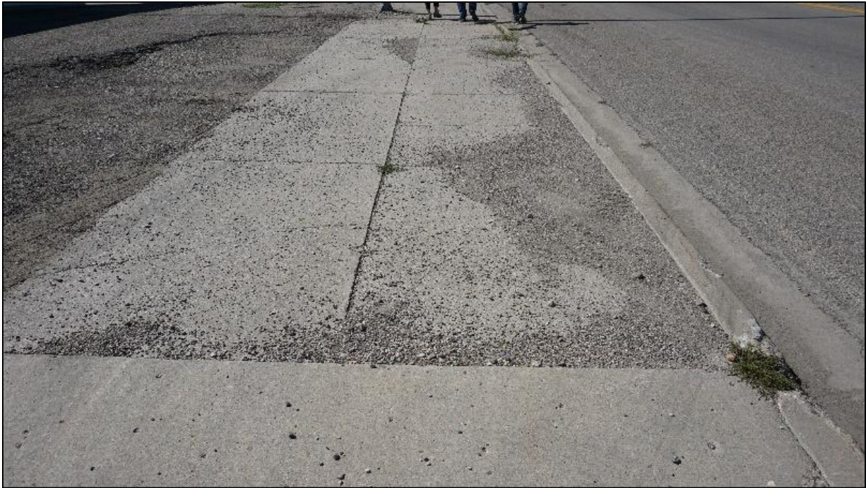
Figure 19. Debris and weeds on the sidewalk
