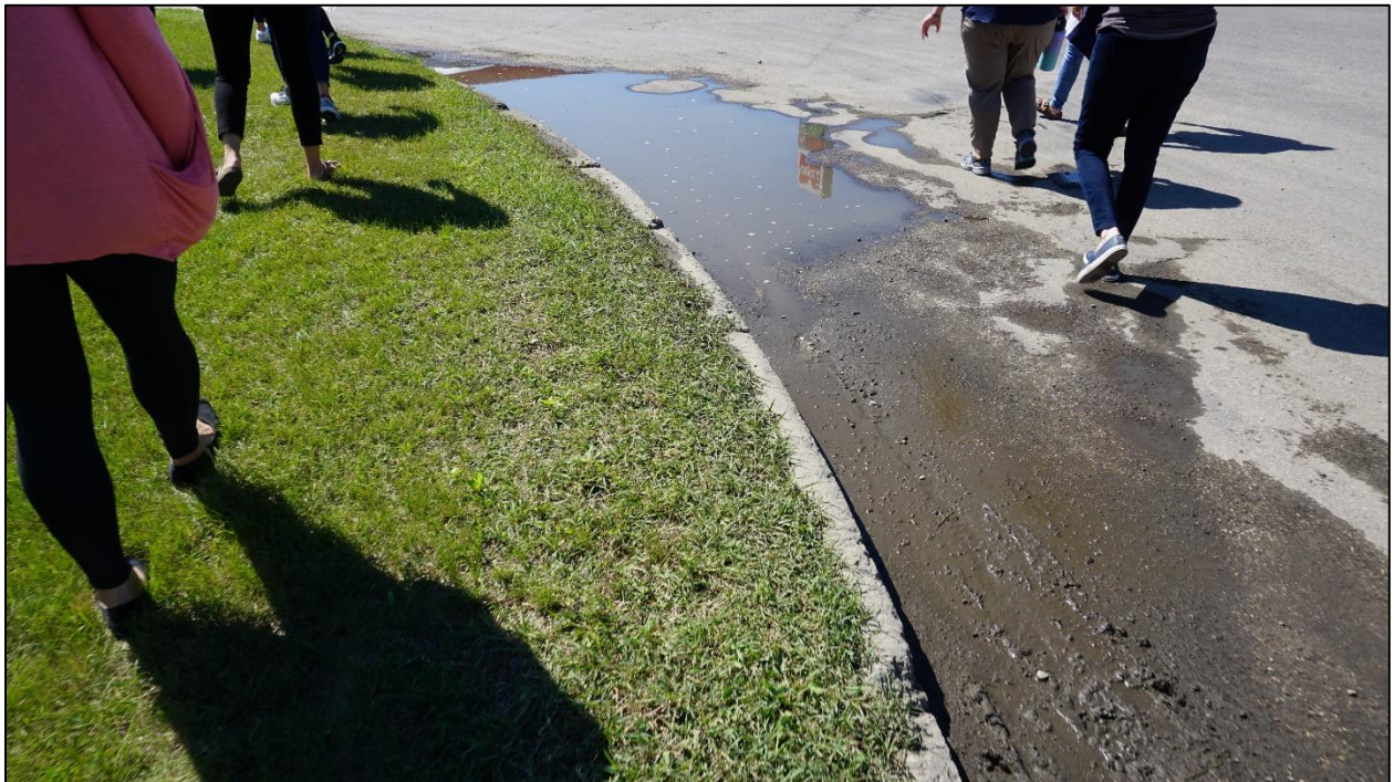
Figure 13. Puddled water at the southeast quadrant of the intersection of ND Highway 1 & ND Highway 5
