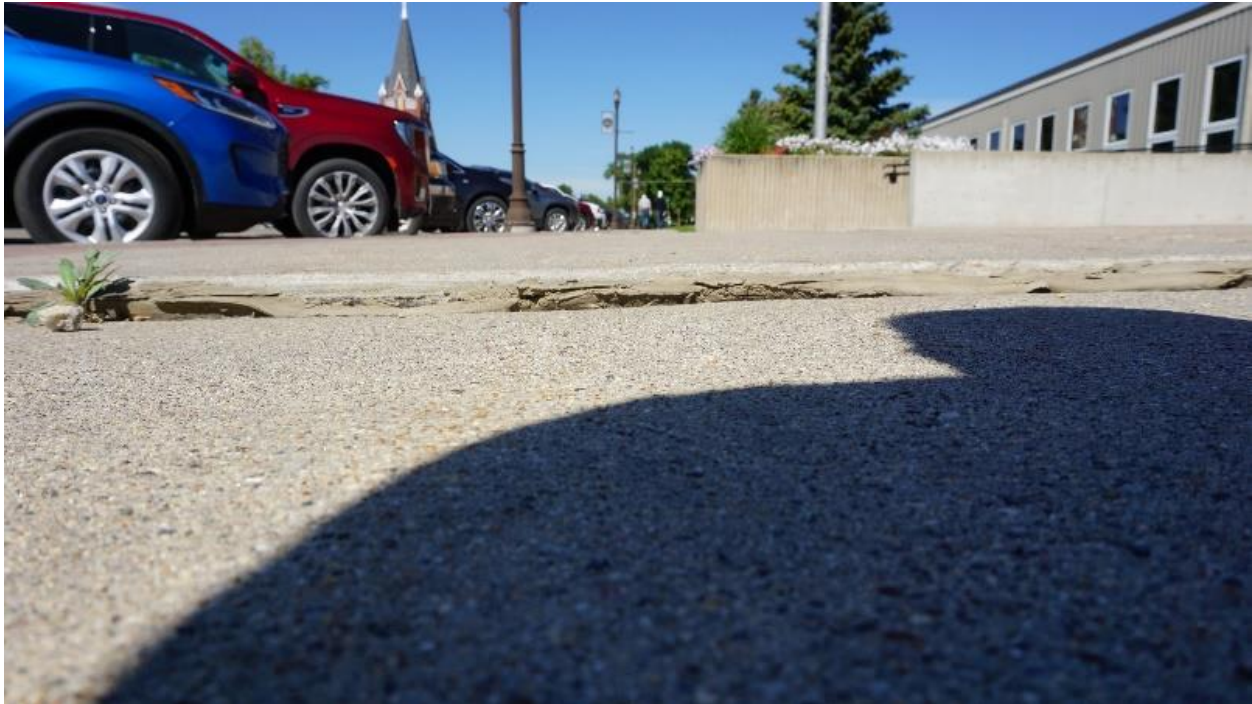
Figure 20. Sidewalk displacement along Third Street
