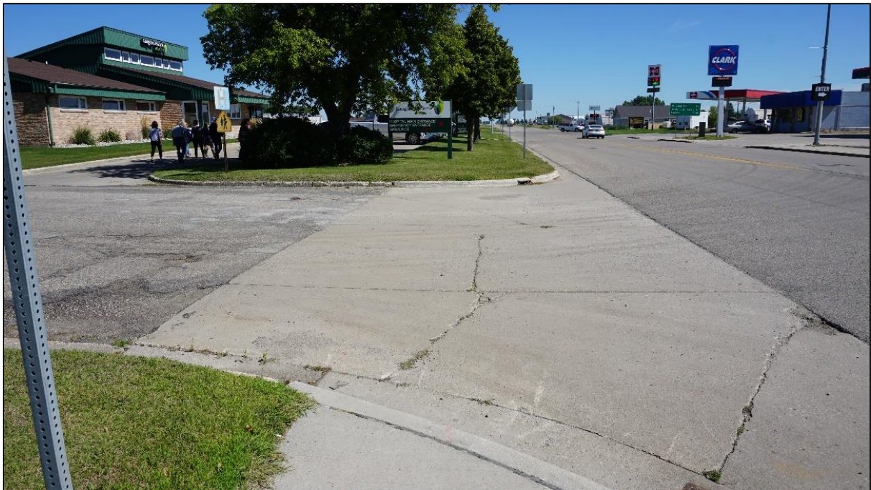
Figure 5. Missing ramps, crosswalk and sidewalk along ND Highway 5
