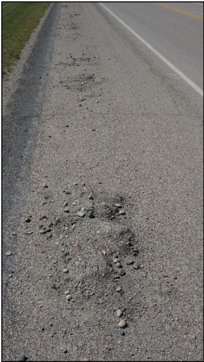
Figure 11. Debris and mud along the south side shoulder of ND Highway 5
