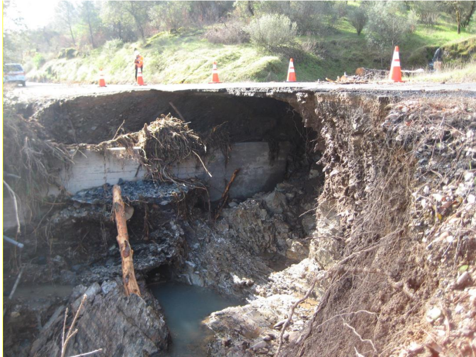
FIGURE 26: DAMAGE ON SR 49 IN TUOLUMNE COUNTY, MARCH 2018
