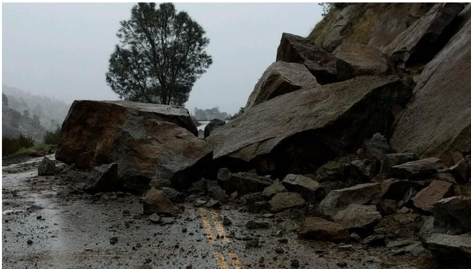
FIGURE 20: SR 178 FLOODING AND ROCK SLIDES, 2018
