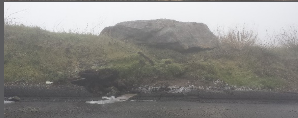
STATE ROUTE 18 | 2017 | ROCKFALL BARRIER STOPS FALLING ROCKS AND DEBRIS
