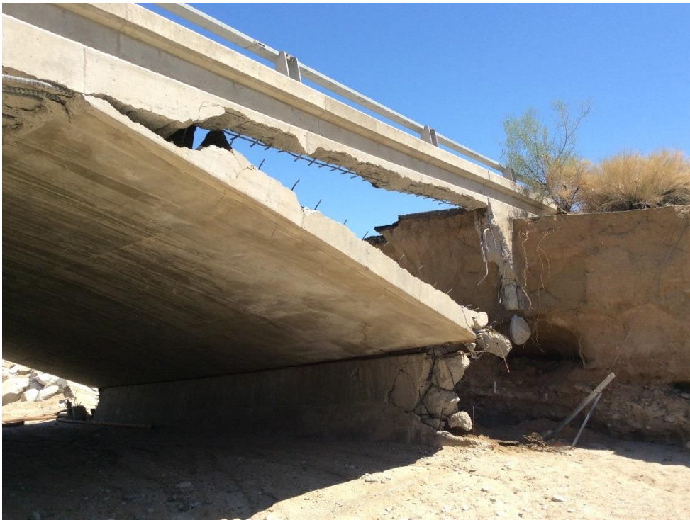
FIGURE 20: TEX WASH BRIDGE ABUTMENT AND DECK COLLAPSE
