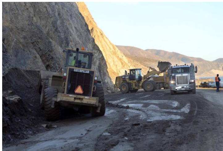
FIGURE 2: CALTRANS STAFF CLEAR DEBRIS FROM POINT MUGU SLIDE IN 2015
