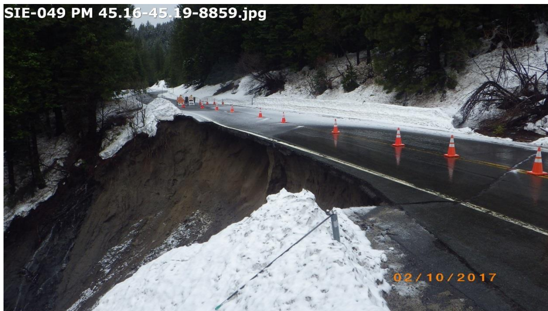
FIGURE 2-3: ROUTE 49 SLIP OUT IN SIERRA COUNTY
