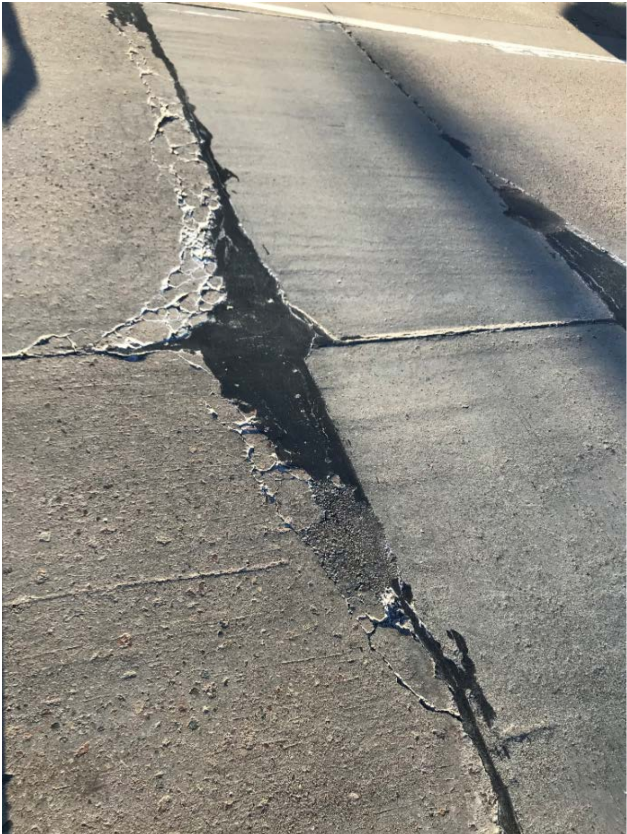
Figure D-8. D Cracking and full-depth repairs in existing concrete pavement (Site #8, State Road 66, Stevens Point).
