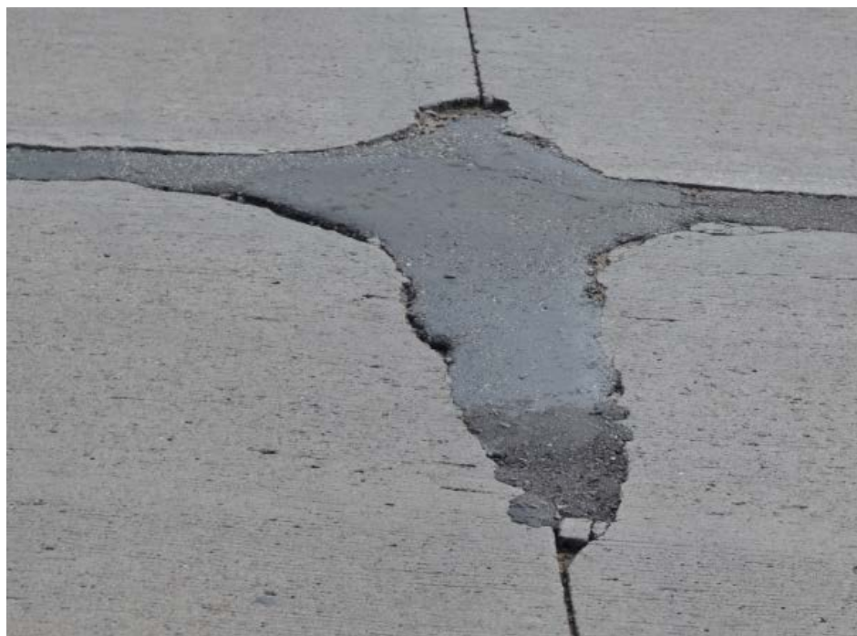
Figure F-13. PDR to address joint deterioration (Site #23, W. Kemp St., Rhinelander).
