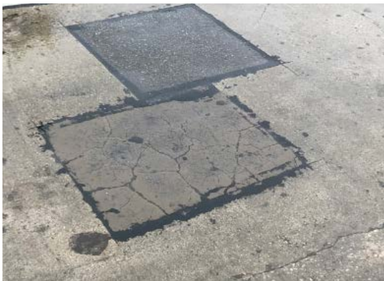
Figure 3-21. Surface map cracking pattern observed on some RM-4 PDRs on Site #16.
