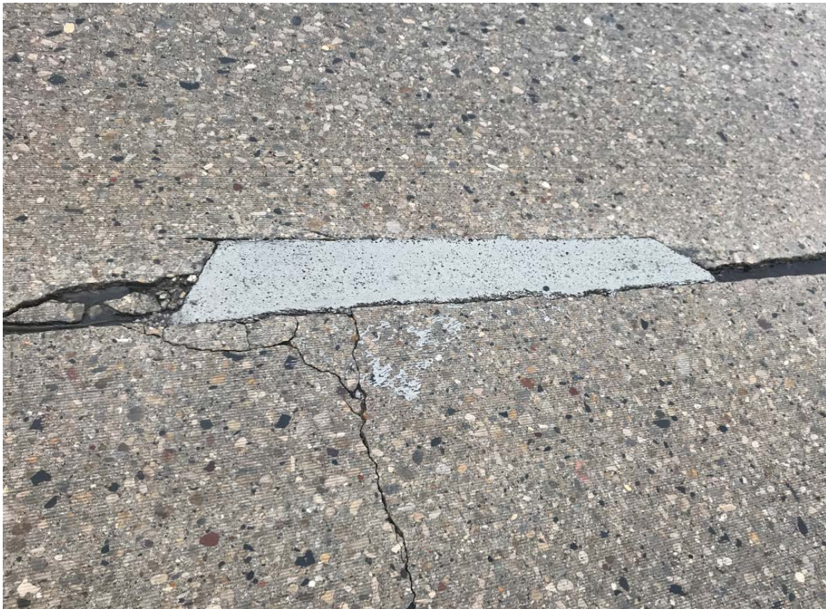
Figure E-16. Concrete pavement deteriorating around the PDR (Site #12, US 41, Marinette).
