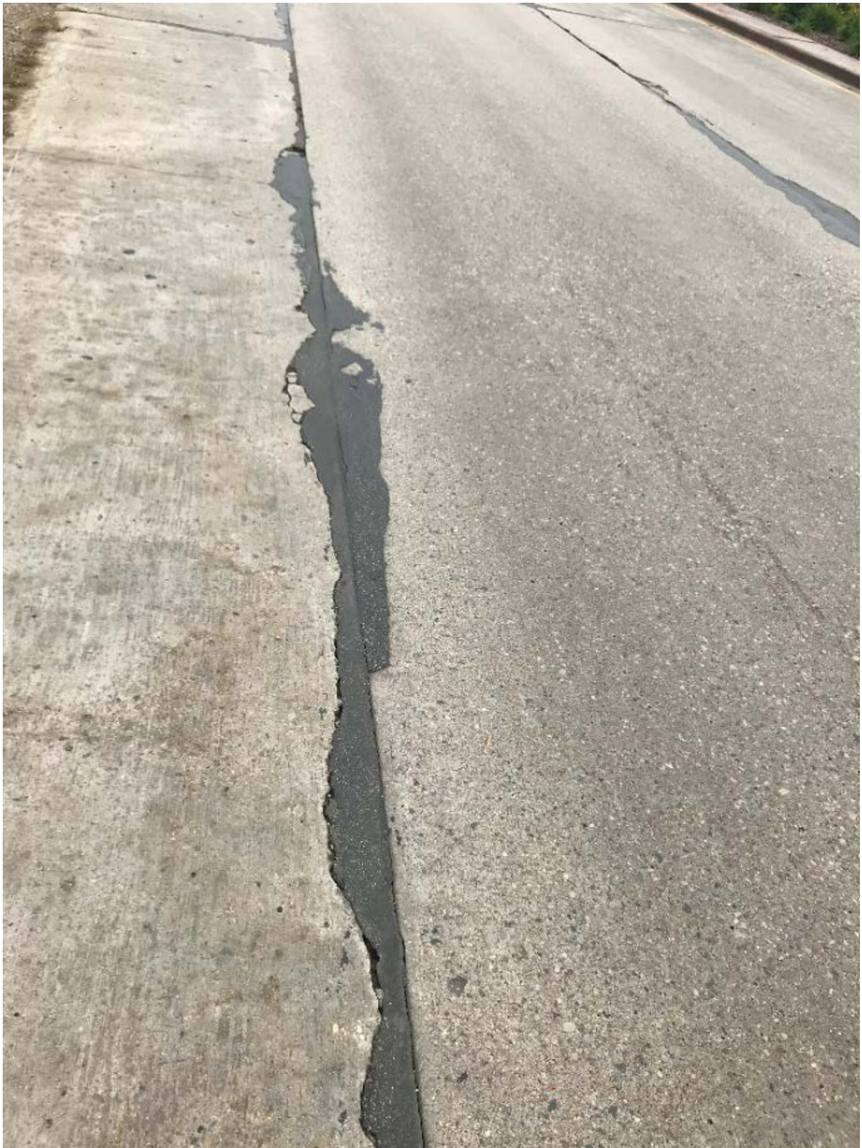
Figure D-3. PDRs to address spalling along lane-shoulder joint (Site #6, Plover Rd., Plover).
