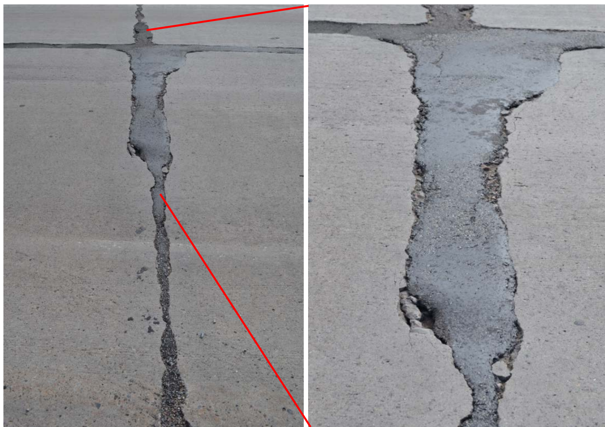
Figure F-12. PDR to address transverse joint deterioration (left) and surrounding concrete pavement deteriorating around PDR (Site #23, W. Kemp St., Rhinelander).
