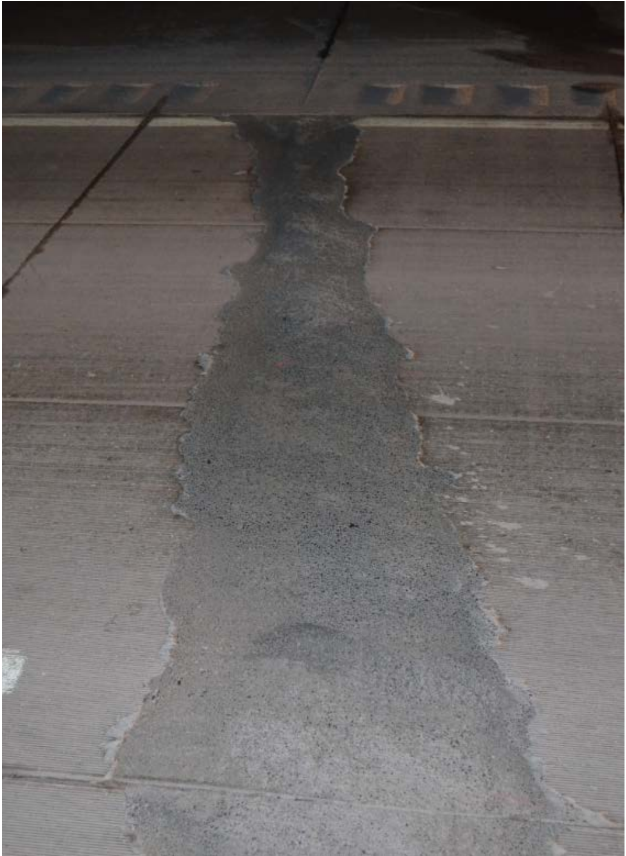
Figure B-9. RM-1 PDR (8)—large, full lane-width patch (Site #1, US 12/18, Madison Beltline).
