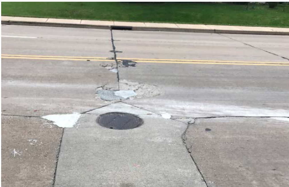
Figure E-23. Existing concrete pavement deteriorating around PDRs (Site #15, Calumet St., Appleton).
