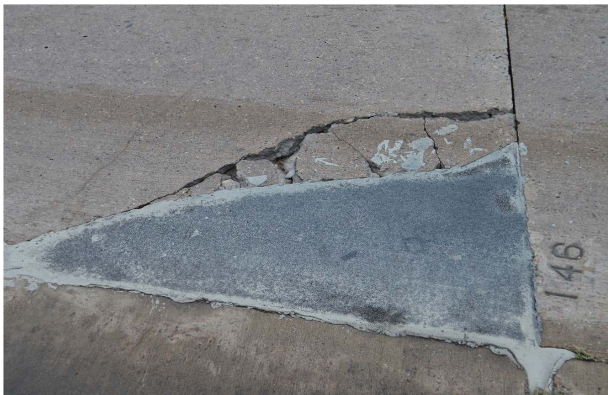
Figure E-8. Concrete pavement deterioration around PDR (Site #11, US 10, Stevens Point).
