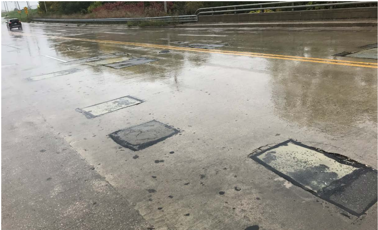
Figure E-24. PDRs on bridge deck (Site #16, W. Main Ave., Ashwaubenon).
