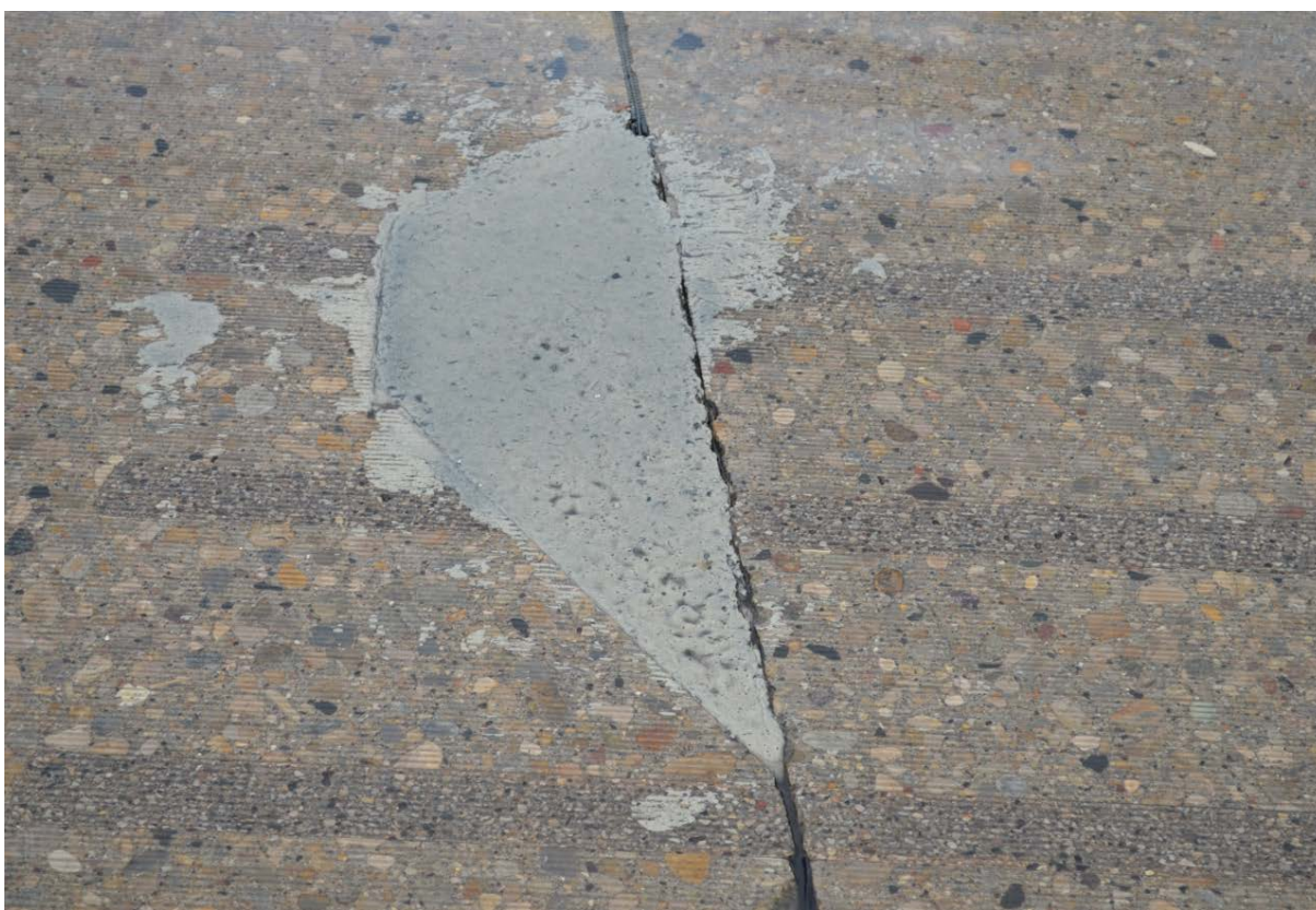
Figure E-15. PDR to address spalling at a transverse joint (Site #12, US 41, Marinette).
