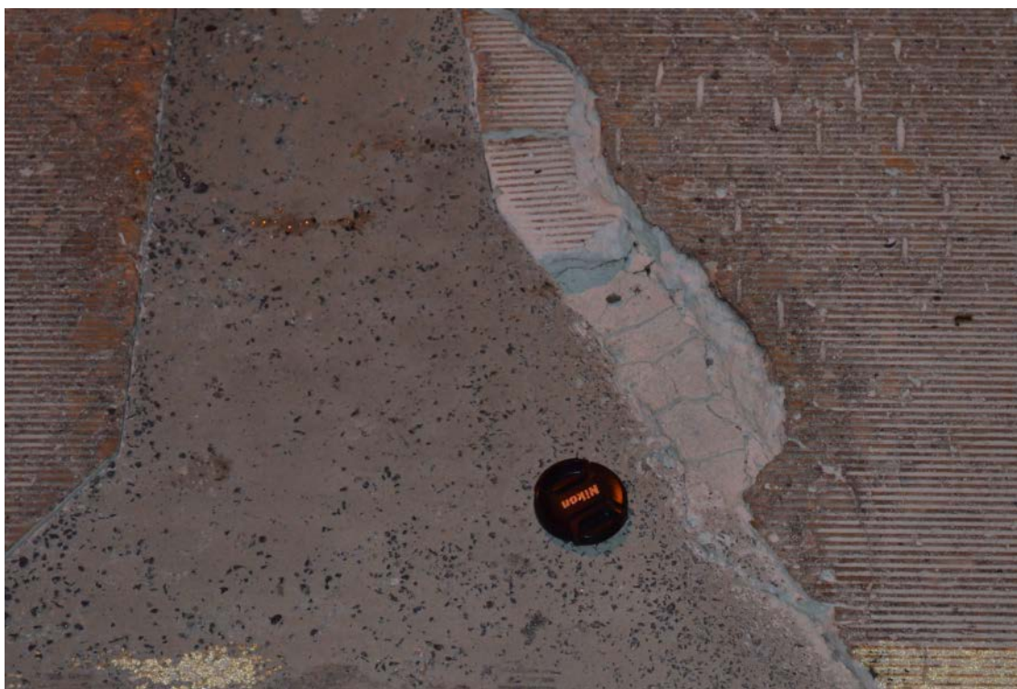
Figure B-7. RM-1 PDR (6)—close-up of deterioration along patch edge (Site #1, US 12/18, Madison Beltline).
