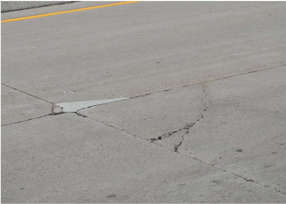
Figure E-12. Corner break in existing concrete pavement (Site #11, US 10, Stevens Point).
