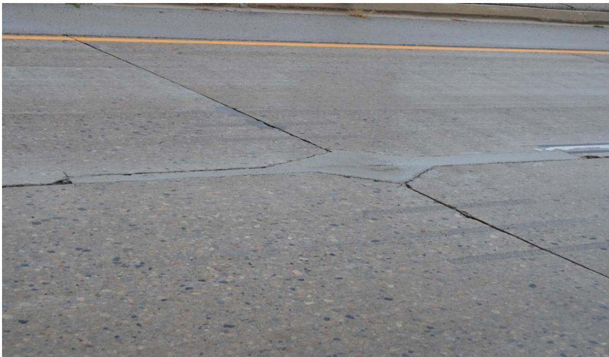
Figure E-17. PDR used to address deteriorated longitudinal joint (Site #12, US 41, Marinette).
