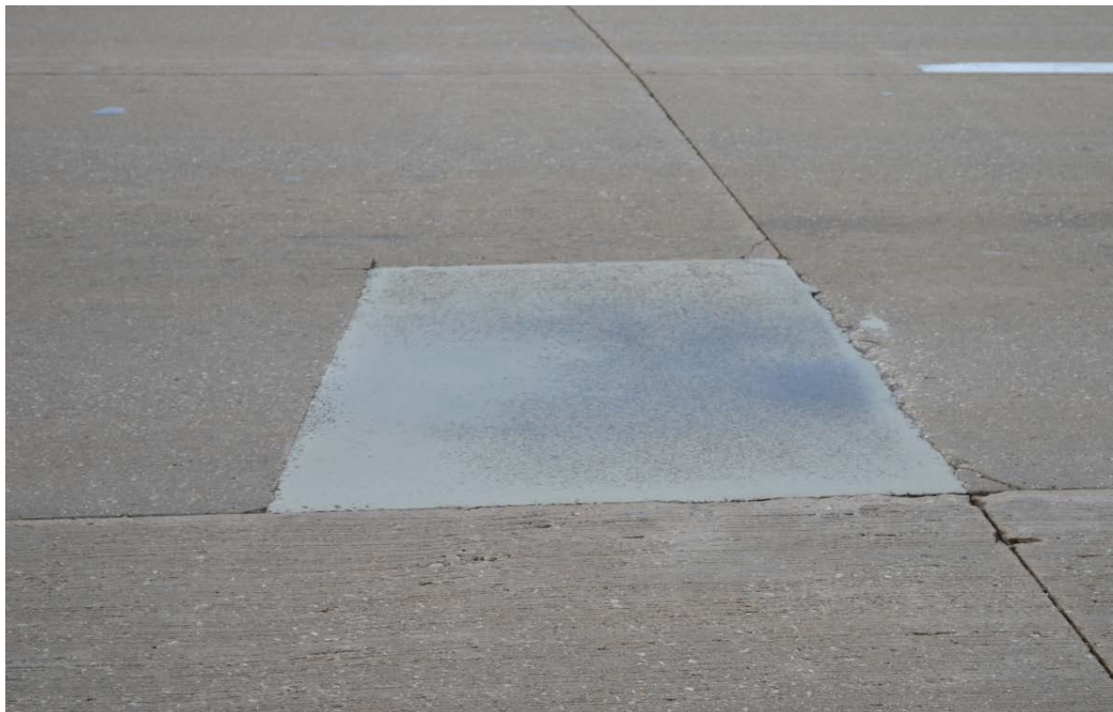
Figure E-27. PDR to address an isolated area of distress in an otherwise distress free pavement (Site #17, W. Johnson St., Fond du Lac).
