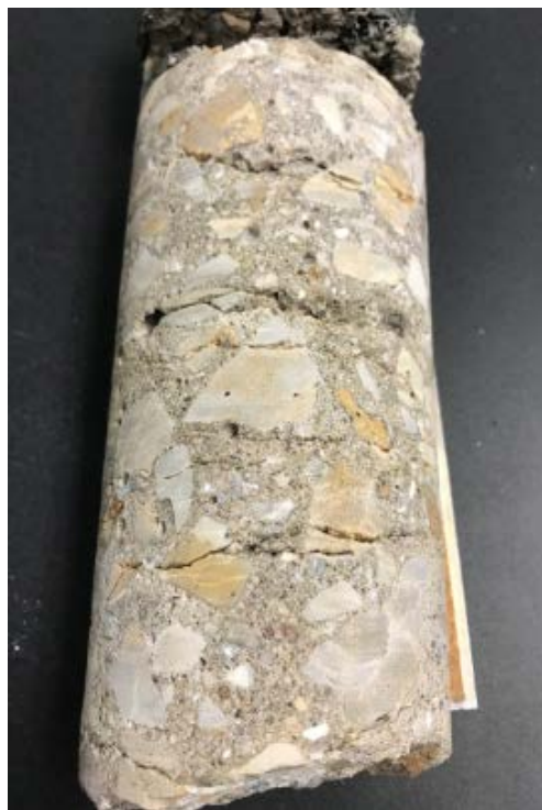
Figure 3-7. Multiple parallel horizontal cracks extending through the entire depth of core #2.
