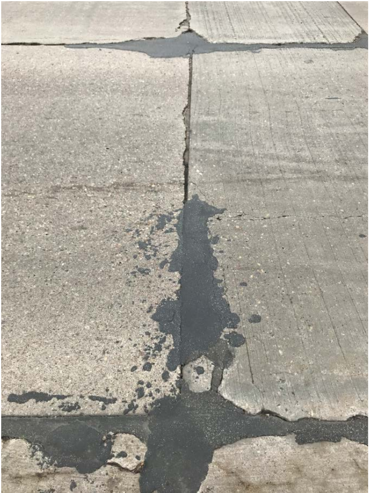
Figure D-2. PDRs to address spalling and deteriorated joints (P Site #6, lower Rd., Plover).
