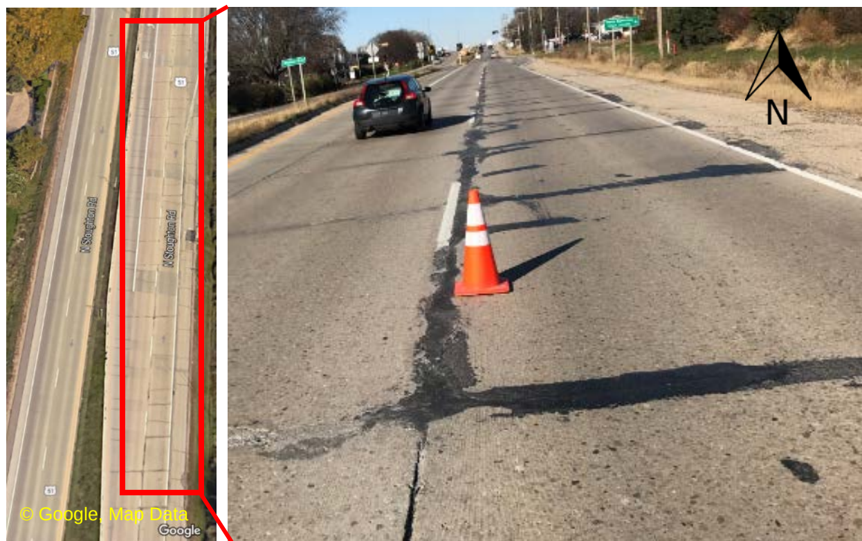
Figure 3-23. Overview of US 51/N. Stoughton Rd northbound lanes(top) and satellite imagery showing severely distressed condition of the north bound lanes.
