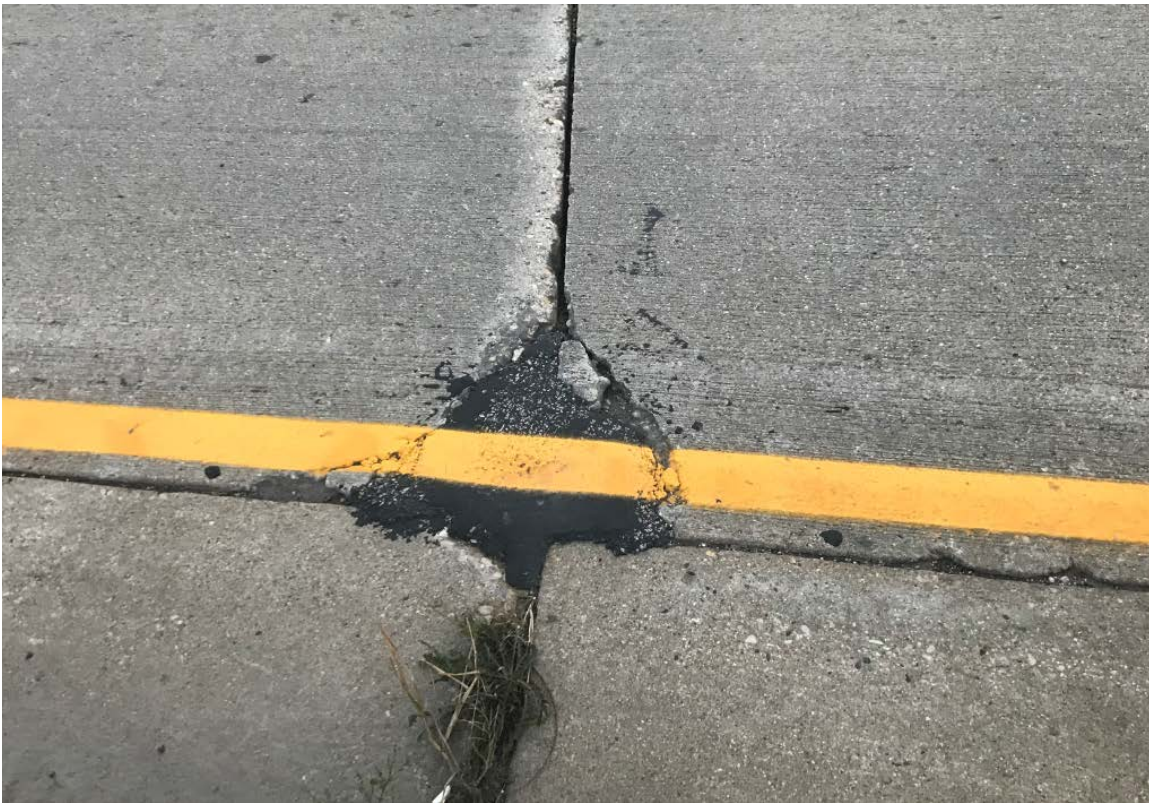
Figure F-7. Existing pavement deteriorating around PDR (Site #21, State Road 59, Waukesha).
