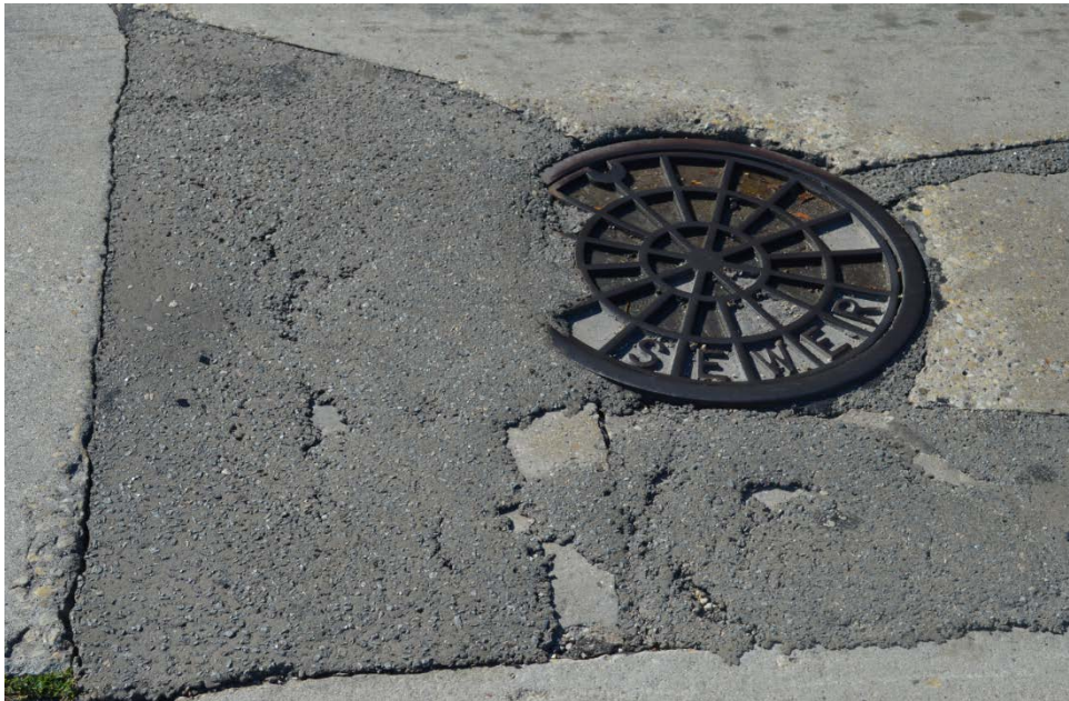
Figure E-2. PDRs to address deteriorated areas around utility hole (Site #9, State Road 66, Stevens Point).
