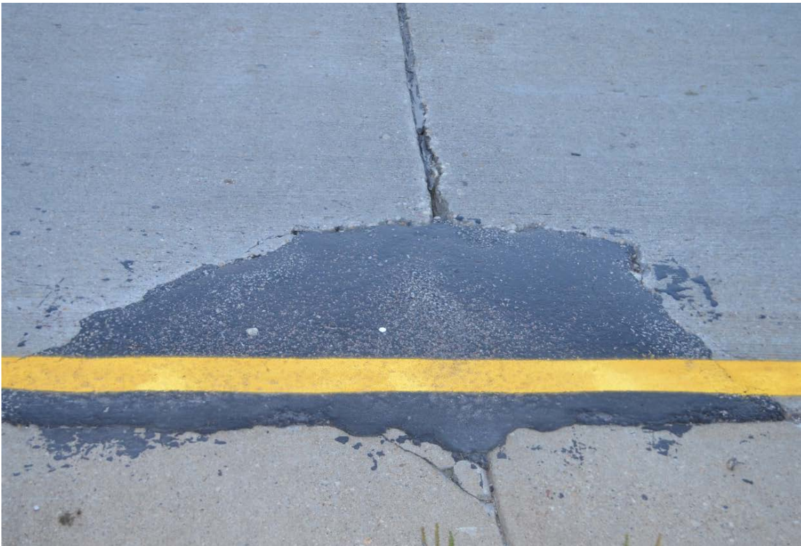
Figure F-6. PDR to address corner spalling (Site #21, State Road 59, Waukesha).
