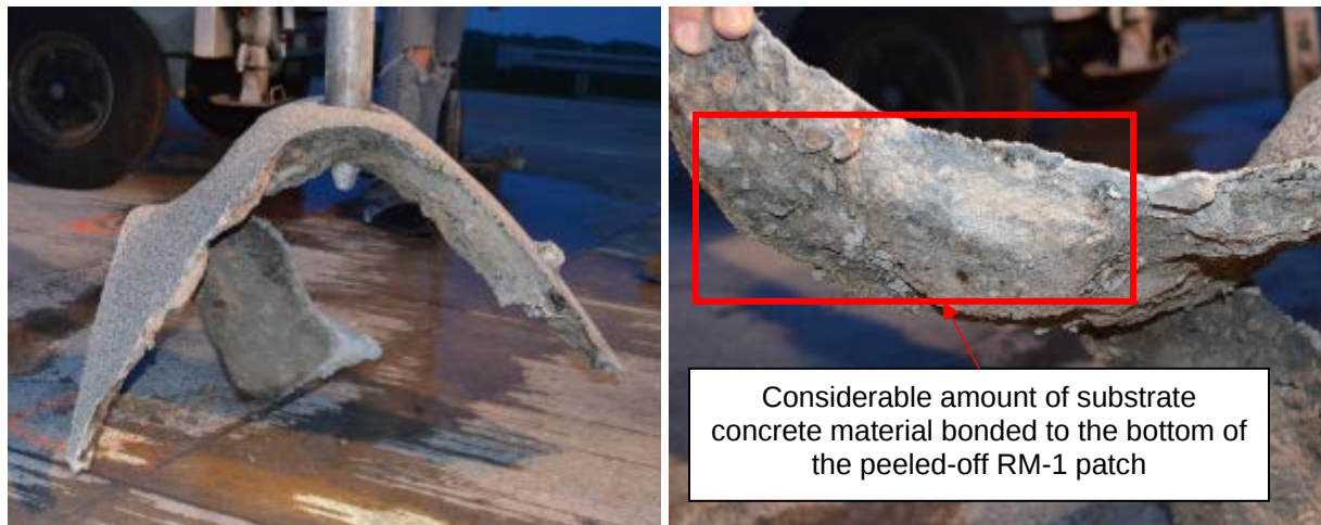
Figure 3-10. RM-1 PDRs peeling off from the concrete pavement.
