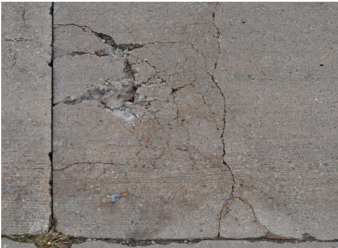
Figure E-10. Severely deteriorated areas in existing concrete pavement (Site #11, US 10, Stevens Point).
