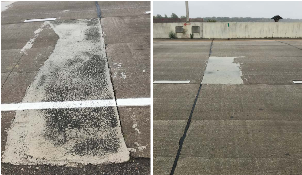
Figure E-28. PDR to address deterioration along transverse joints (Site #18, I 41, Oshkosh).
