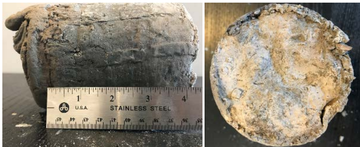
Figure 3-18. RM-4 core from Site #11 (left) and bottom of the core showing substrate concrete material bonded to the repair material (right).
