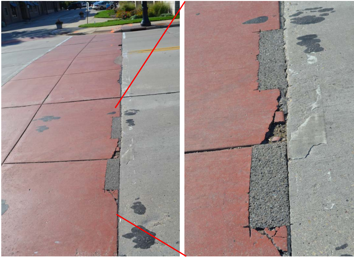
Figure E-1. PDRs along transverse joint (Site #9, Washington St., Grafton).
