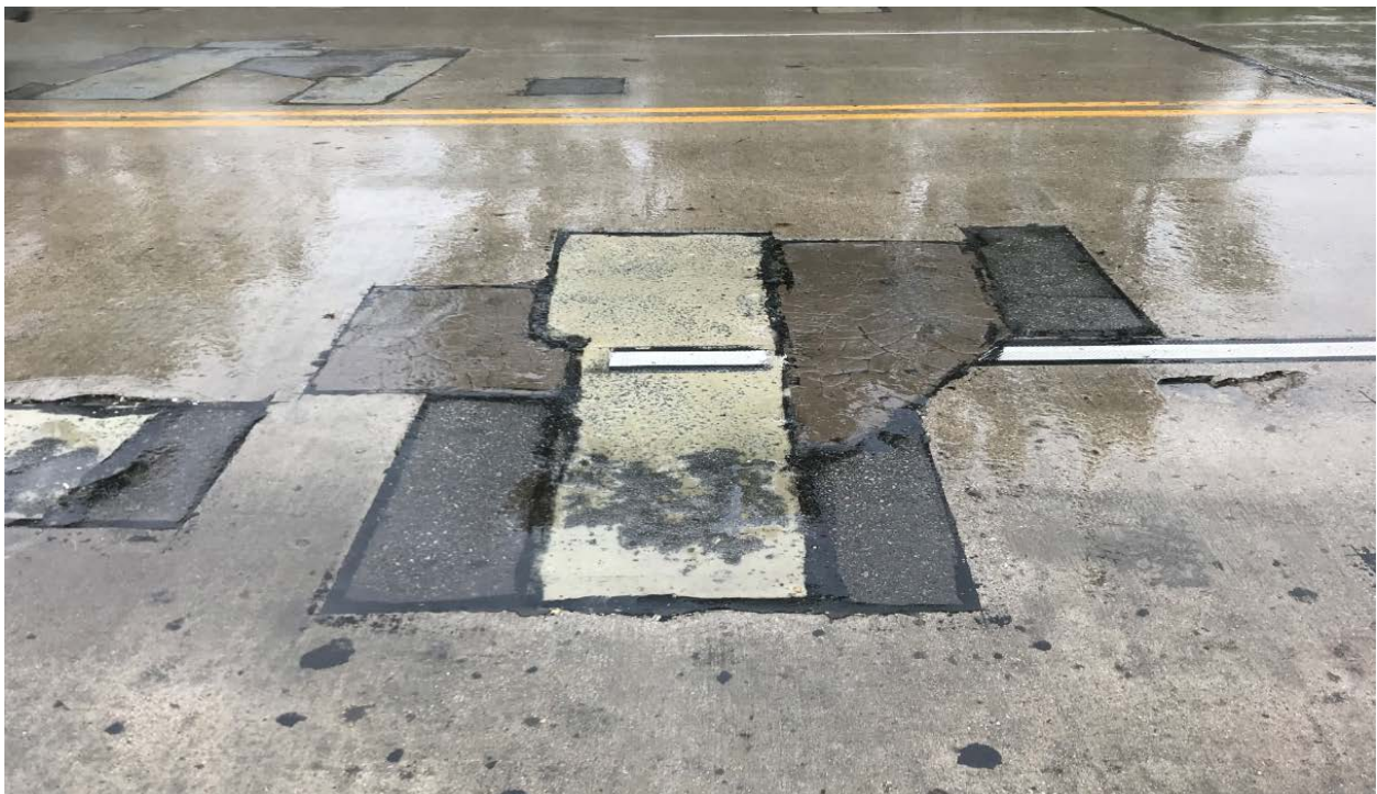
Figure E-25. RM-4 PDRs on bridge deck with starkly different colors (Site #16, W. Main Ave., Ashwaubenon).
