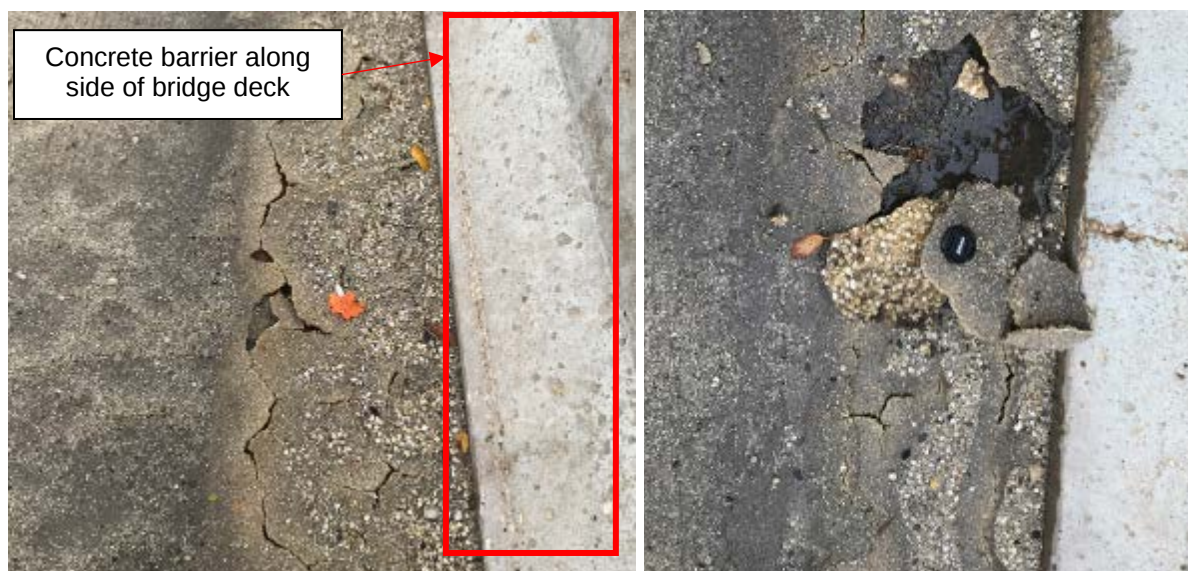
Figure 3-12. Top one-third of the RM-2 overlay peeling off along the deck edge (Site #3).
