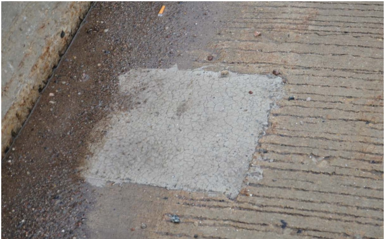
Figure E-19. Map cracking pattern on PDR surface (Site #13, State Road 32, Mountain).
