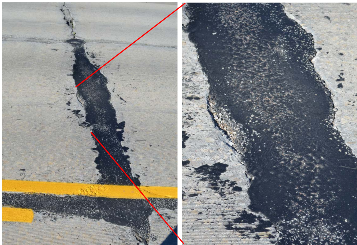
Figure F-9. PDR to address deteriorated joint (left) and existing pavement deteriorating around PDR (right) (Site #22, N. Ballard Rd., Appleton).
