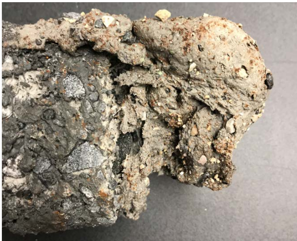
Figure A-10. Site #1, RM-1 Core #3—Closeup of melted material (US 12/18, Madison Beltline).
