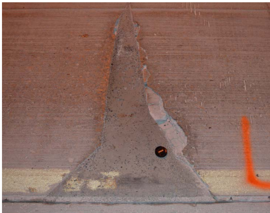
Figure B-6. RM-1 PDR (6)—deterioration along patch edges (Site #1, US 12/18, Madison Beltline).
