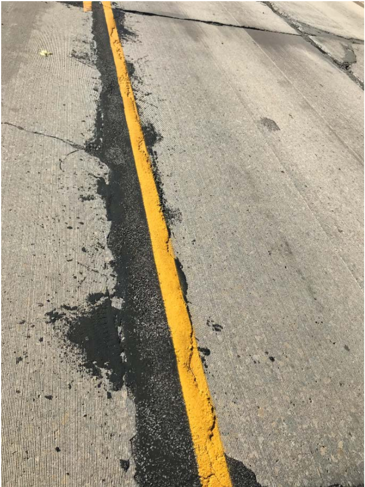
Figure F-10. PDR to address longitudinal joint deterioration (Site #22, N. Ballard Rd., Appleton).
