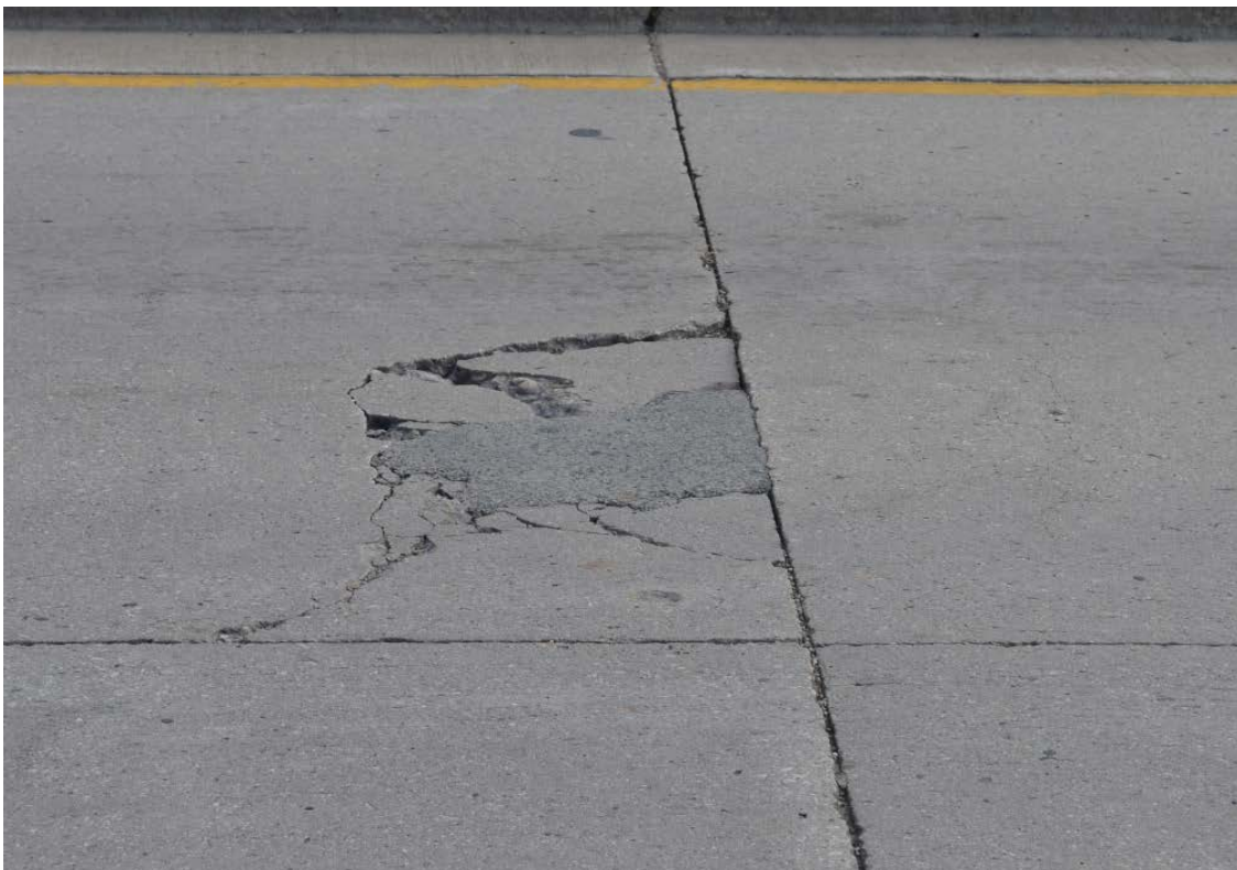
Figure E-6. Concrete pavement deterioration around PDR (Site #10, State Road 145, Menomonee Falls).
