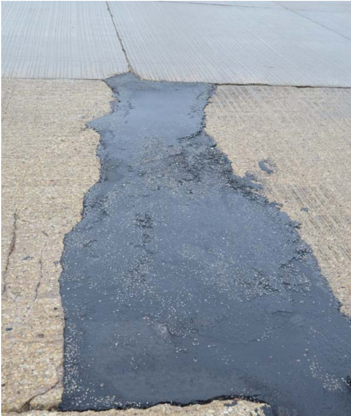
Figure F-1. PDR to address deterioration along transverse joint (Site #19, State Road 93, Eau Claire).
