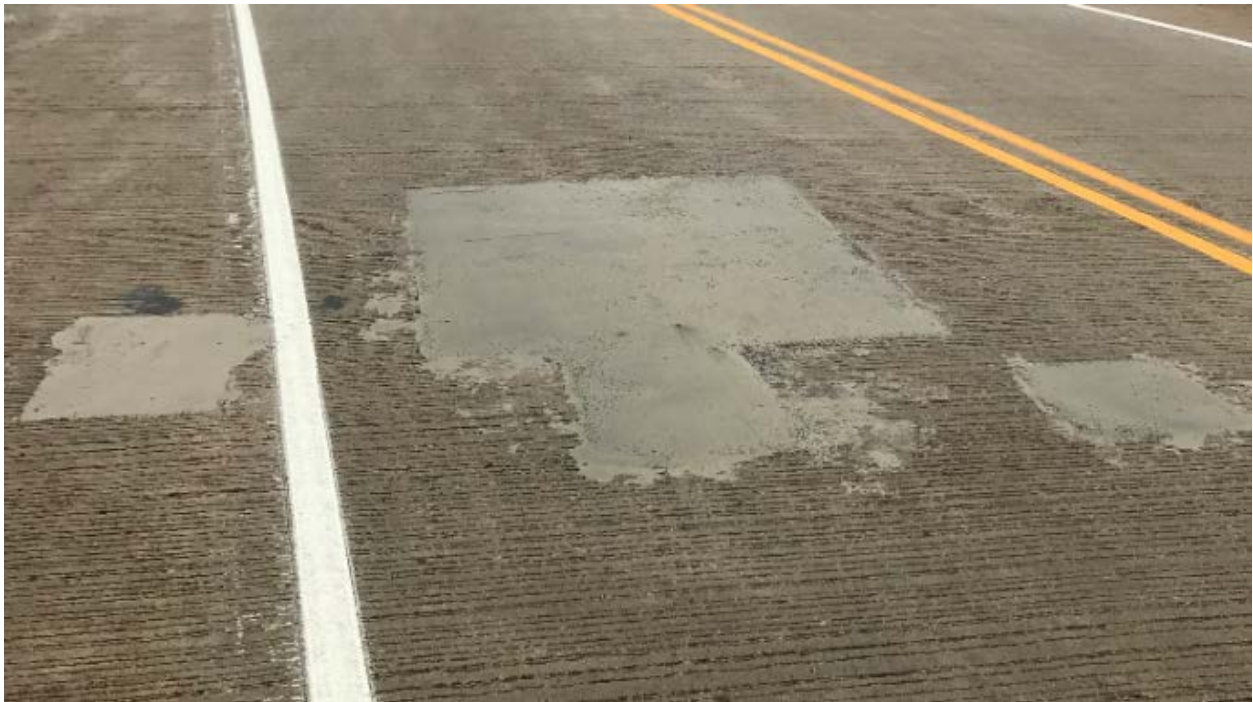
Figure E-18. PDRs on bridge deck (1) (Site #13, State Road 32, Mountain).
