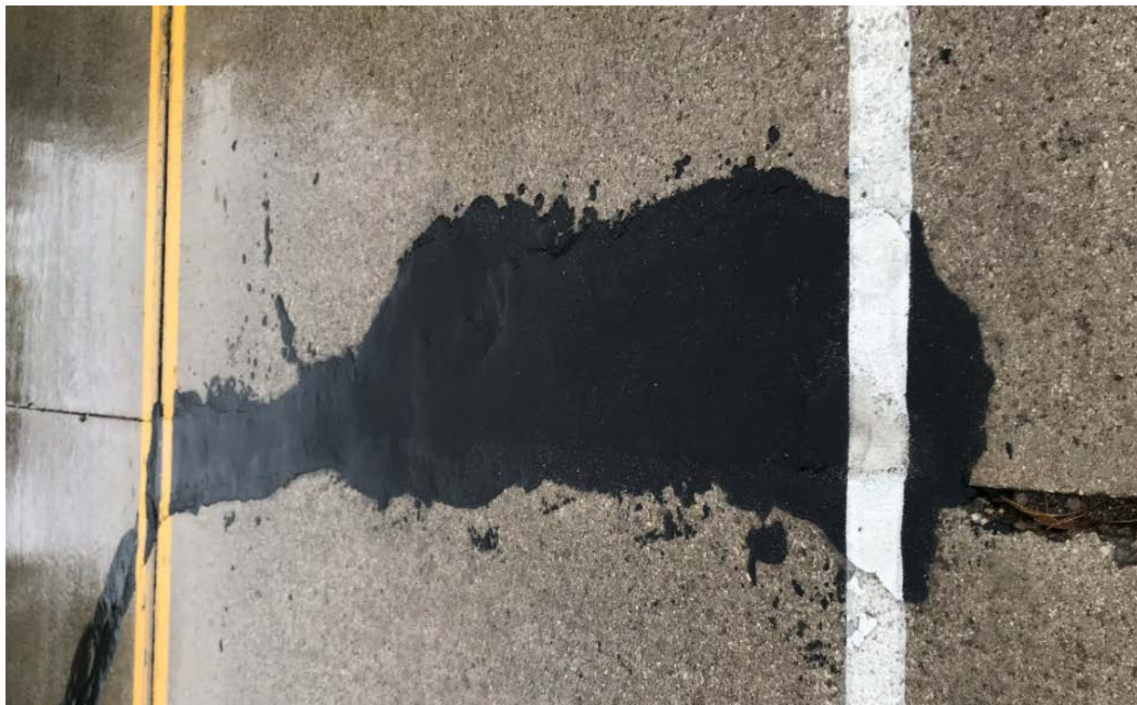
Figure D-6. PDRs along transverse joint (Site #7 S. Taylor St., Green Bay).
