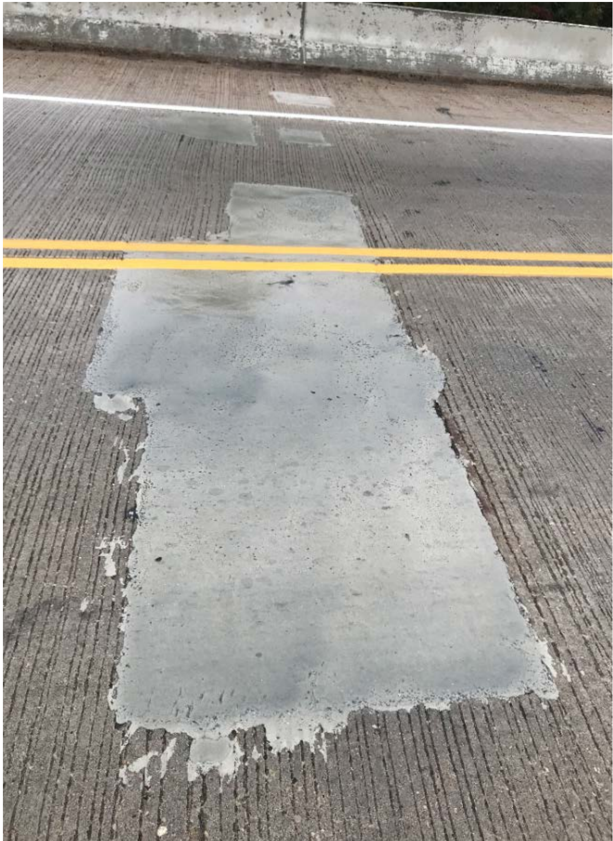
Figure E-20. PDRs on bridge deck (2) (Site #13, State Road 32, Mountain).
