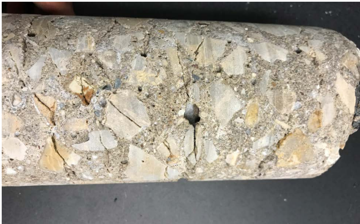
Figure A-6. Site #1, RM-1 Core #2—Closeup of PCC core (US 12/18, Madison Beltline).
