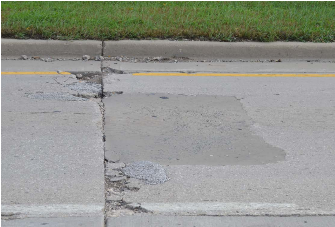
Figure E-5. Concrete pavement deterioration adjacent to PDR (Site #10, State Road 145, Menomonee Falls).
