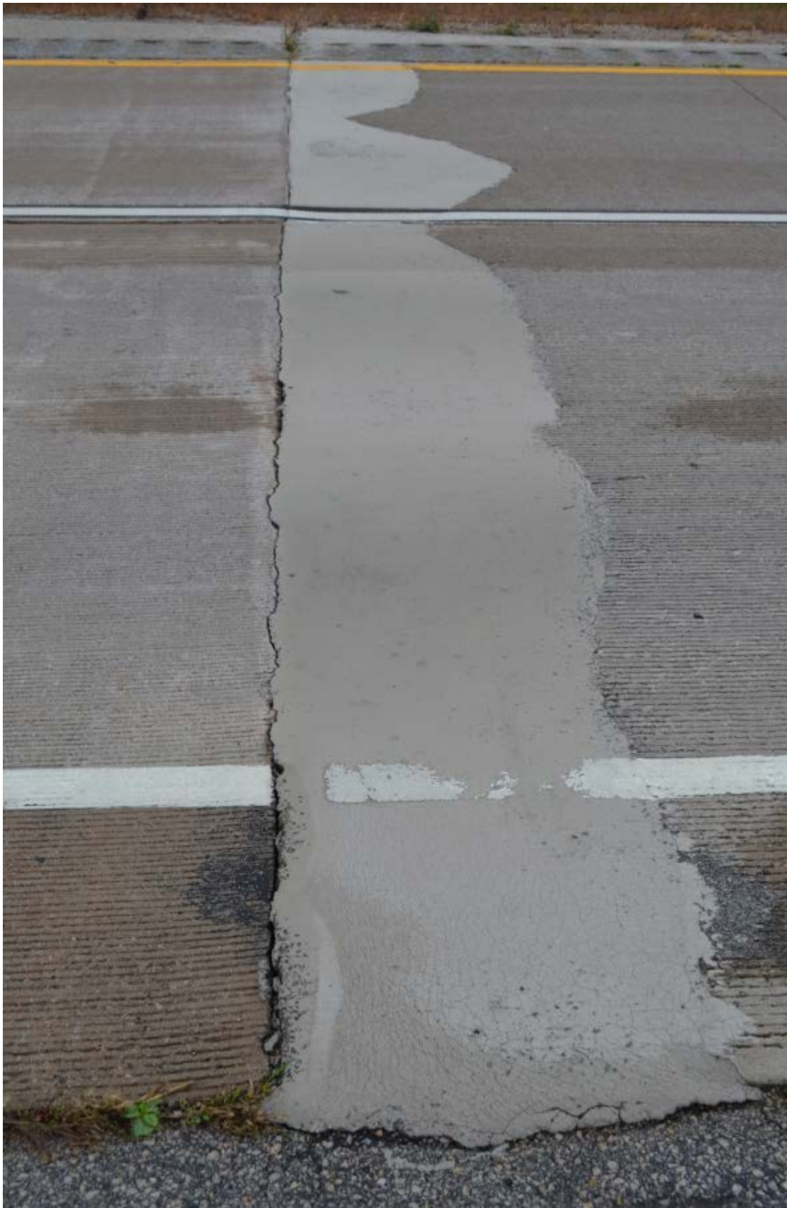
Figure E-21. PDR on bridge deck approach slabs, surface map cracking in shoulder area (Site #14, US 141, Pound).
