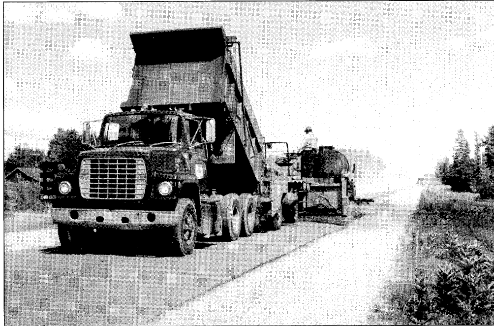
Michigan DOT relies on a wide variety of preventive maintenance treatments to extend the life of its pavements. Here, a chip seal is applied.
