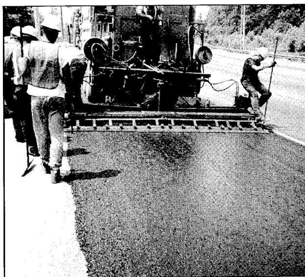
Georgia DOT has recently added microsurfacing to its arsenal of preventive maintenance treatments.
