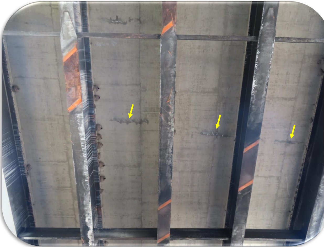
Figure 17. Garrison Bridge - 2020 inspection - Typical deck underside condition (suspended span). Transverse cracks at arrows.
