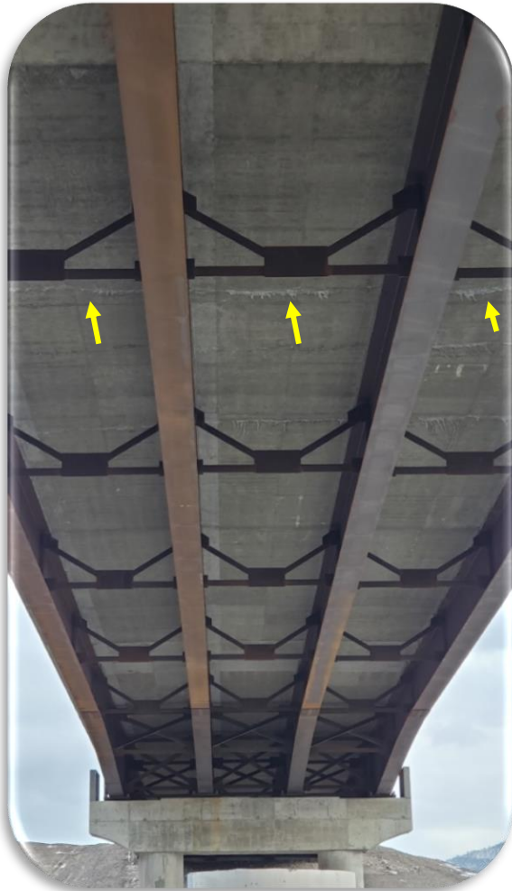
Figure 31. Bonner Bridge Phase I (EB) - 2019 Inspection - Typical deck underside condition, placement 3. Transverse crack at arrows.
