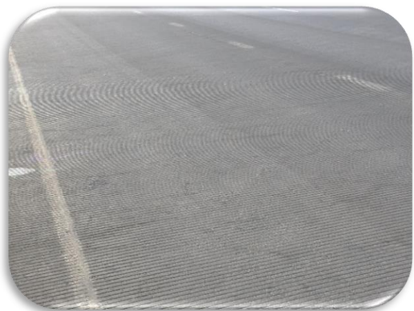
Figure 24. Map cracking at the end of placement 5.
