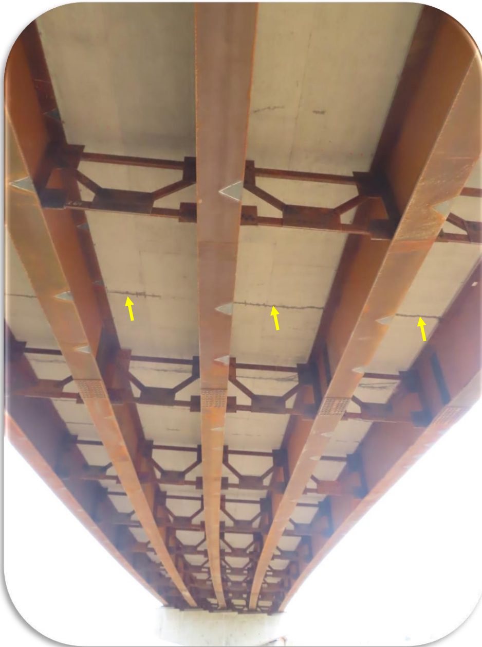
Figure 46. Underside of Rarus/Silver Bow Creek Bridge D - 2020 inspection - Span 2, Typical transverse crack at arrows.
