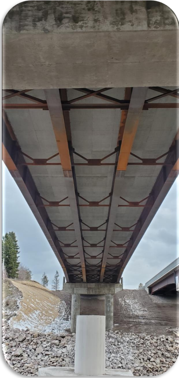
Figure 36. Bonner Bridge Phase II (WB) - 2019 Inspection - Typical deck underside condition, Span 2 - Looking east.
