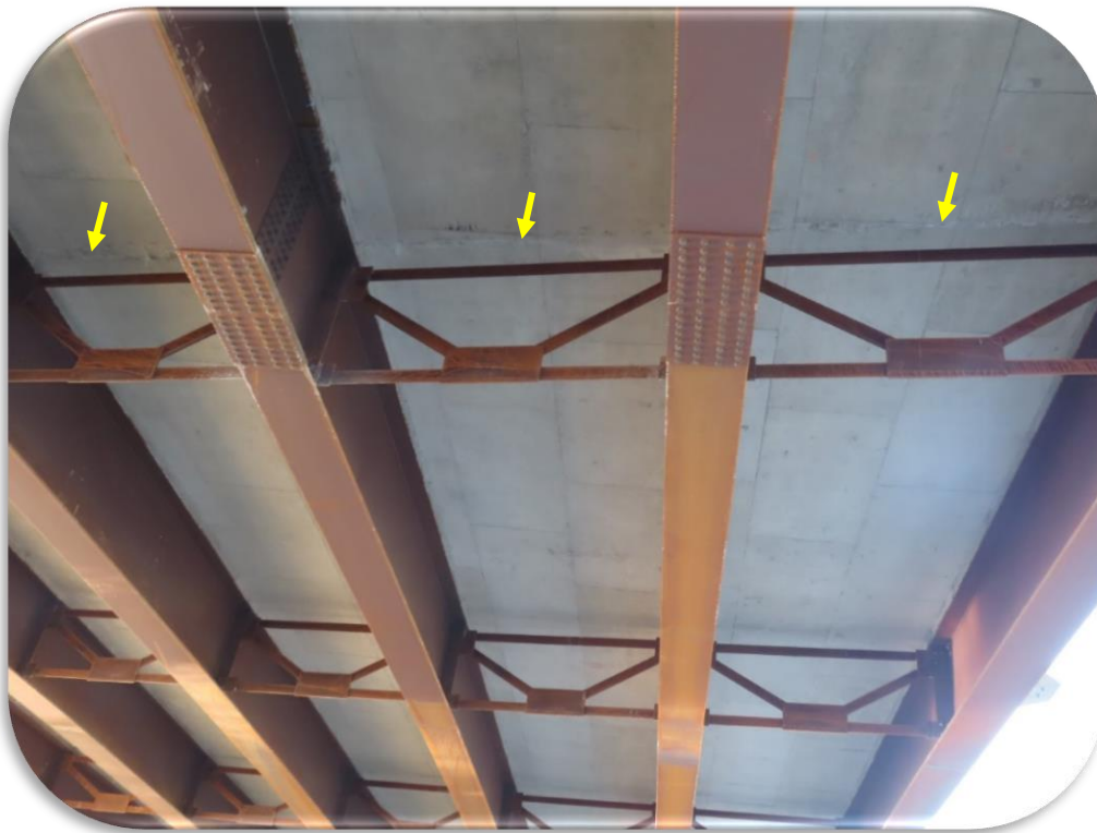
Figure 11. Russell Street Bridge - Phase II, 2020 Inspection - Typical transverse cracks (arrows) in placement 1, underside.
