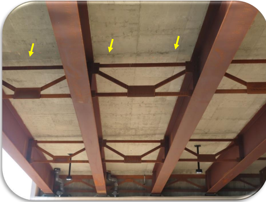
Figure 9. Russell Street Bridge - Phase I, 2020 Inspection - Placement 1, underside. A typical transverse crack at arrows.
