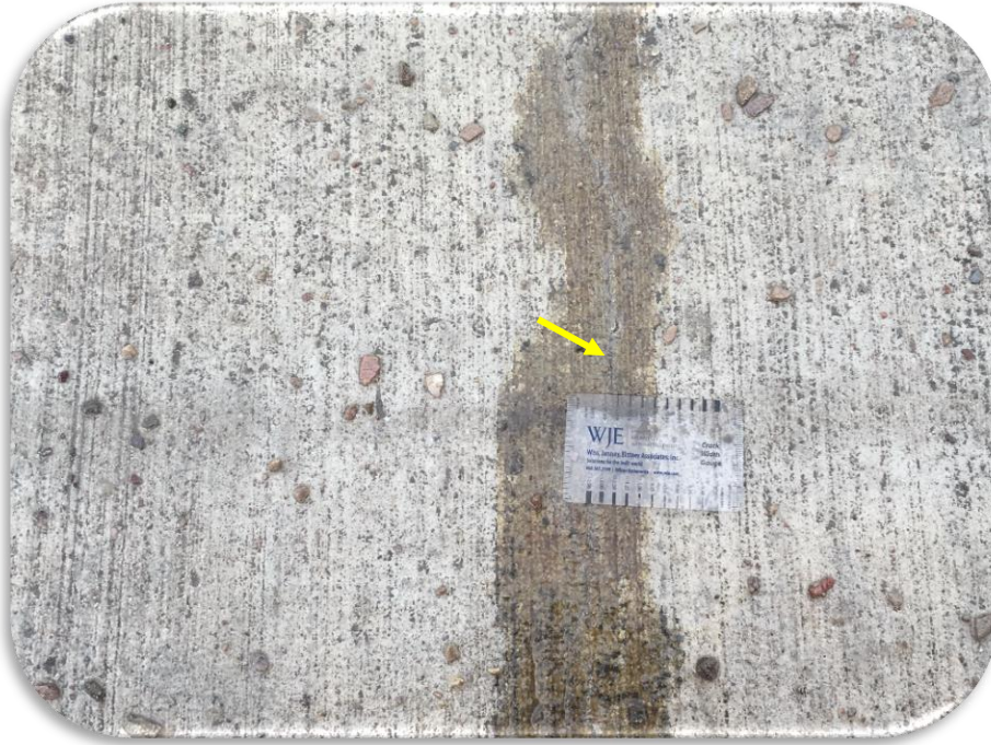
Figure 6. Russell Street Bridge - Phase I, 2019 Inspection - Placement 1, topside. A 15-mil transverse crack at arrow.
