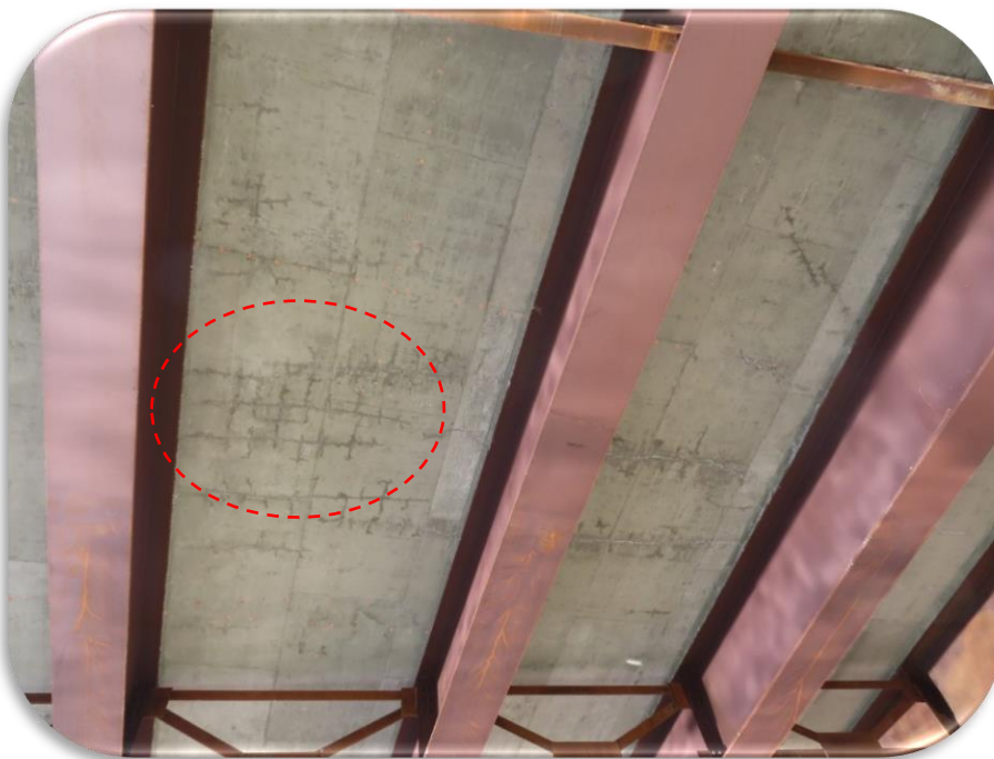
Figure 10. Russell Street Bridge - Phase I, 2020 Inspection - Placement 1, underside. Intersecting cracks in red oval.
