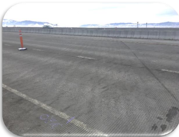
Figure 23. Map cracking at beginning of placement 3.
