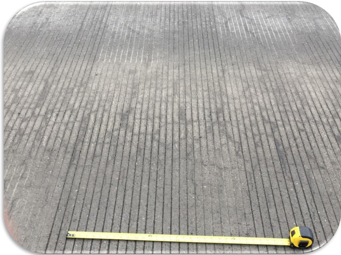
Figure 32. Bonner Bridge Phase I (EB) - 2019 Inspection - Typical map cracking, placement 5.
