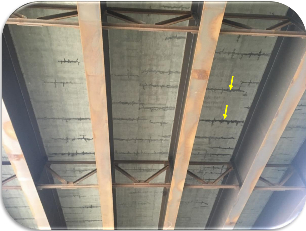
Figure 22. Capitol-Cedar Bridge Phase I (NB) - Typical deck underside transverse cracks at arrows (Placement 3).
