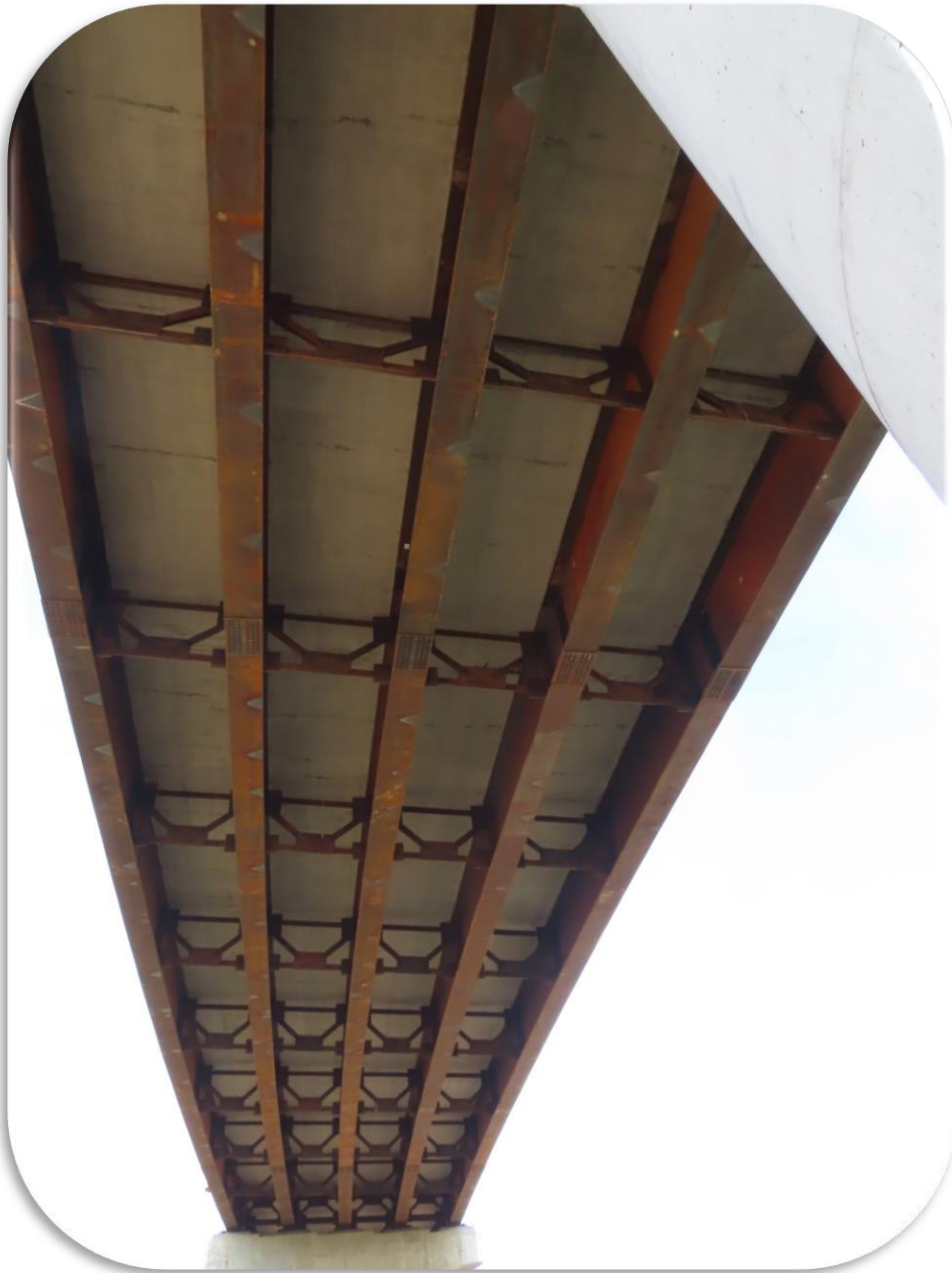
Figure 45. Underside of Rarus Structures - Silver Bow Creek - Bridge C - 2020 inspection, Span 2 overall view.
