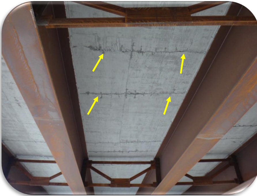
Figure 7. Russell Street Bridge - Phase I, 2019 Inspection - Placement 3, underside. Typical transverse cracks at arrows.
