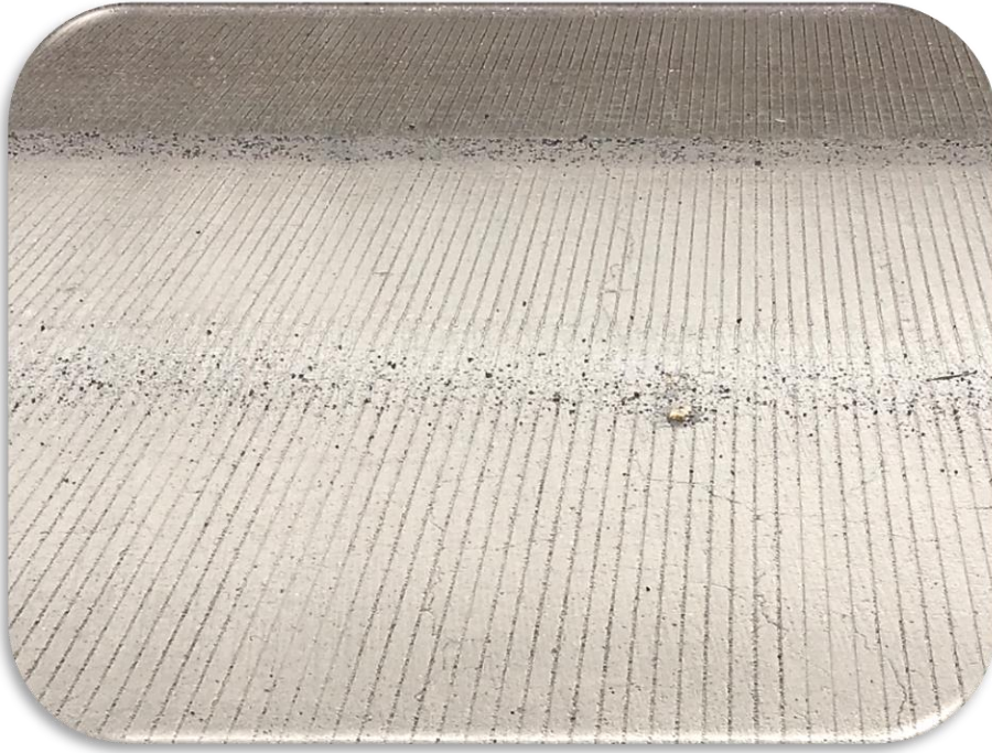
Figure 8. Russell Street Bridge - Phase I, 2019 Inspection - Map cracking in placement 5.
