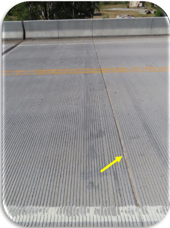
Figure 12. Garrison Bridge - Sealed control joint (at arrow) in concrete deck. Photo taken in 2020.
