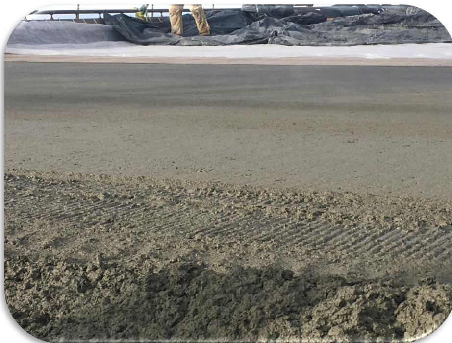
Figure 77. The finished surface of the concrete showing some surface voids, and difficulty closing of the surface.
