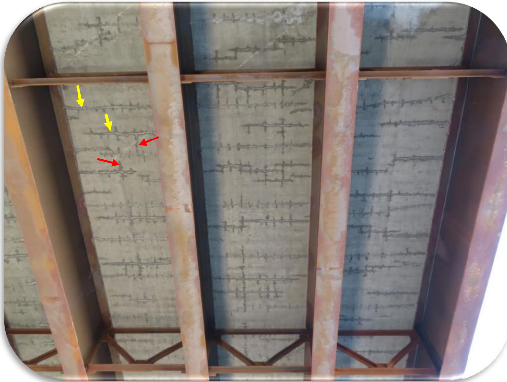
Figure 29. Capitol-Cedar Bridge Phase II (SB) - 2020 inspection. Typical deck underside transverse cracks at yellow arrows); short, hairline longitudinal cracks at red arrows.
