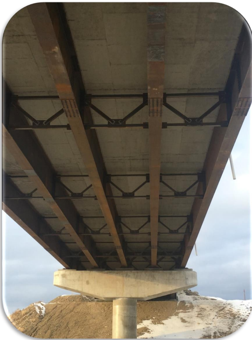
Figure 38. Underside of Rarus/Silver Bow Creek Bridge A - 2019 inspection, condition is very good (Span 2 shown).
