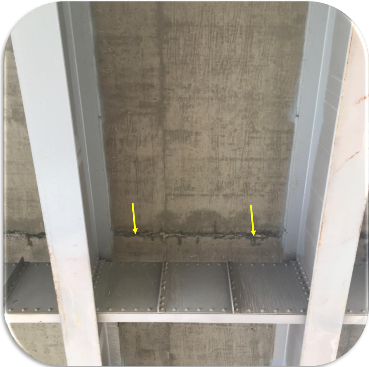
Figure 15. Garrison Bridge - 2019 inspection - Efflorescence on the deck underside at a construction joint (at arrows).
