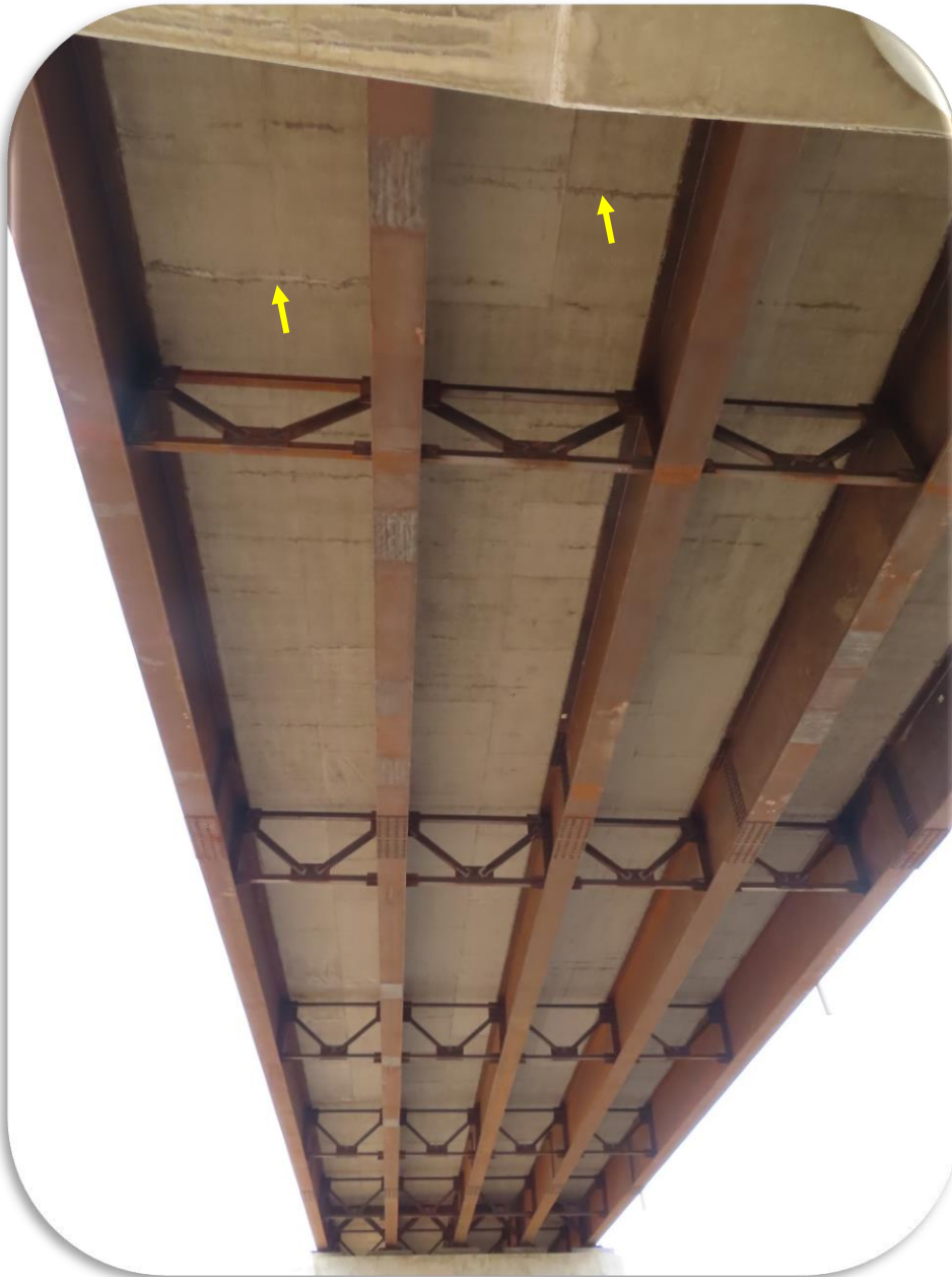
Figure 39. Underside of Rarus/Silver Bow Creek Bridge A - 2020 inspection - Span 2, Typical transverse cracks at arrows.
