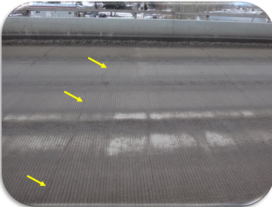
Figure 5. Russell Street Bridge - Phase I, 2019 Inspection - Placement 1, topside. Typical transverse crack at arrows.
