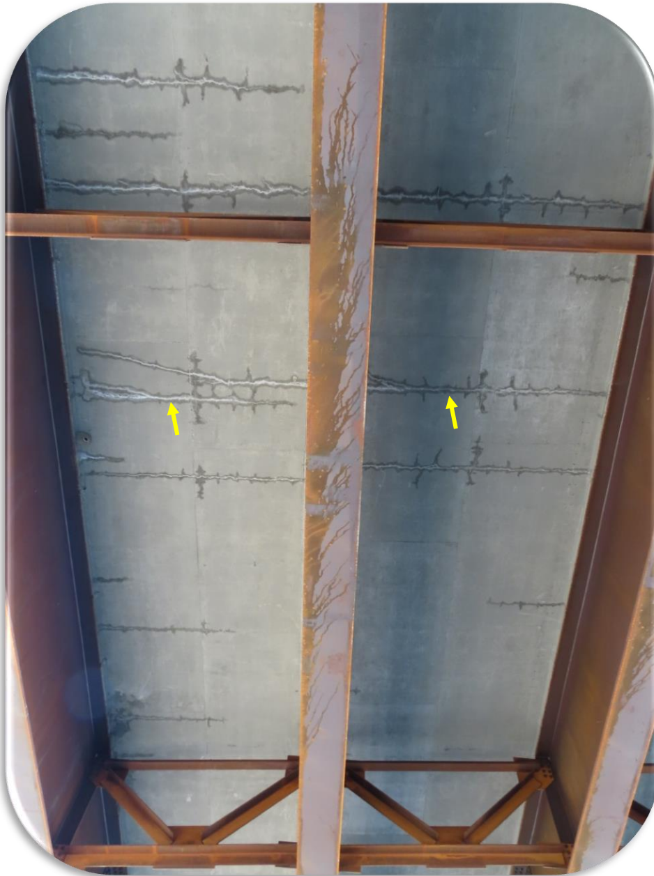
Figure 50. West Laurel Interchange - Phase II - 2020 inspection - Placement 1. Typical transverse crack at arrows.
