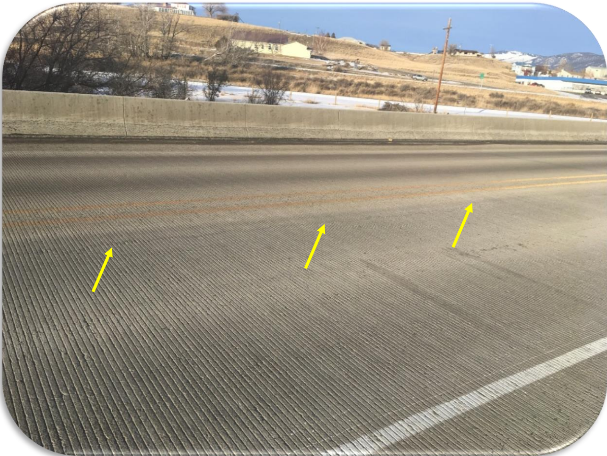
Figure 18. Whitehall Bridge - 2019 inspection - Typical deck topside condition. Arrows point to a longitudinal crack.
