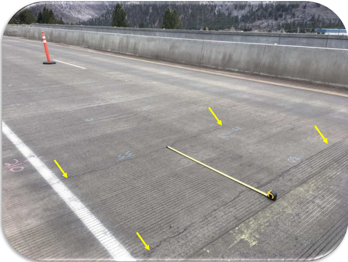
Figure 30. Bonner Bridge Phase I (EB) - 2019 inspection - Typical deck topside transverse cracks, placement 5.
