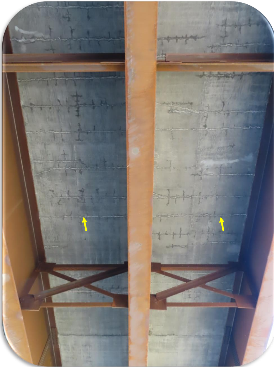
Figure 49. West Laurel Interchange - Phase I - 2020 inspection - Placement 1. Typical transverse crack at arrows.
