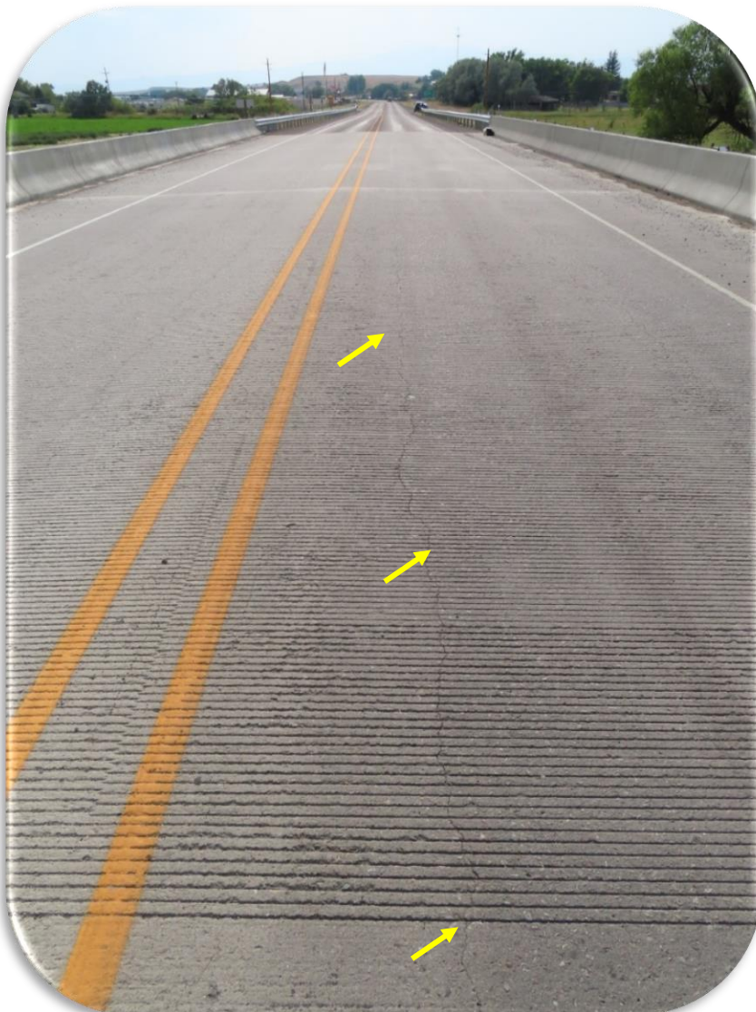
Figure 20. Whitehall Bridge - 2020 inspection - Typical deck topside condition. Arrows point to longitudinal cracking.
