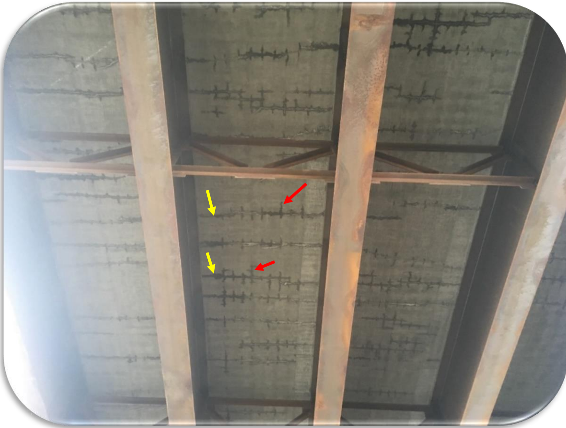
Figure 28. Capitol-Cedar Bridge Phase II (SB) - 2019 inspection. Placement 3. Typical deck underside transverse cracks at yellow arrows; short, hairline longitudinal cracks at red arrows.
