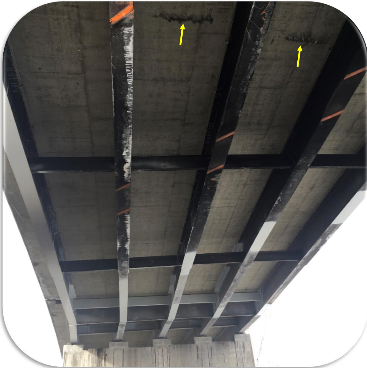
Figure 14. Garrison Bridge - 2019 inspection - Typical deck underside condition. Transverse cracks at arrows.
