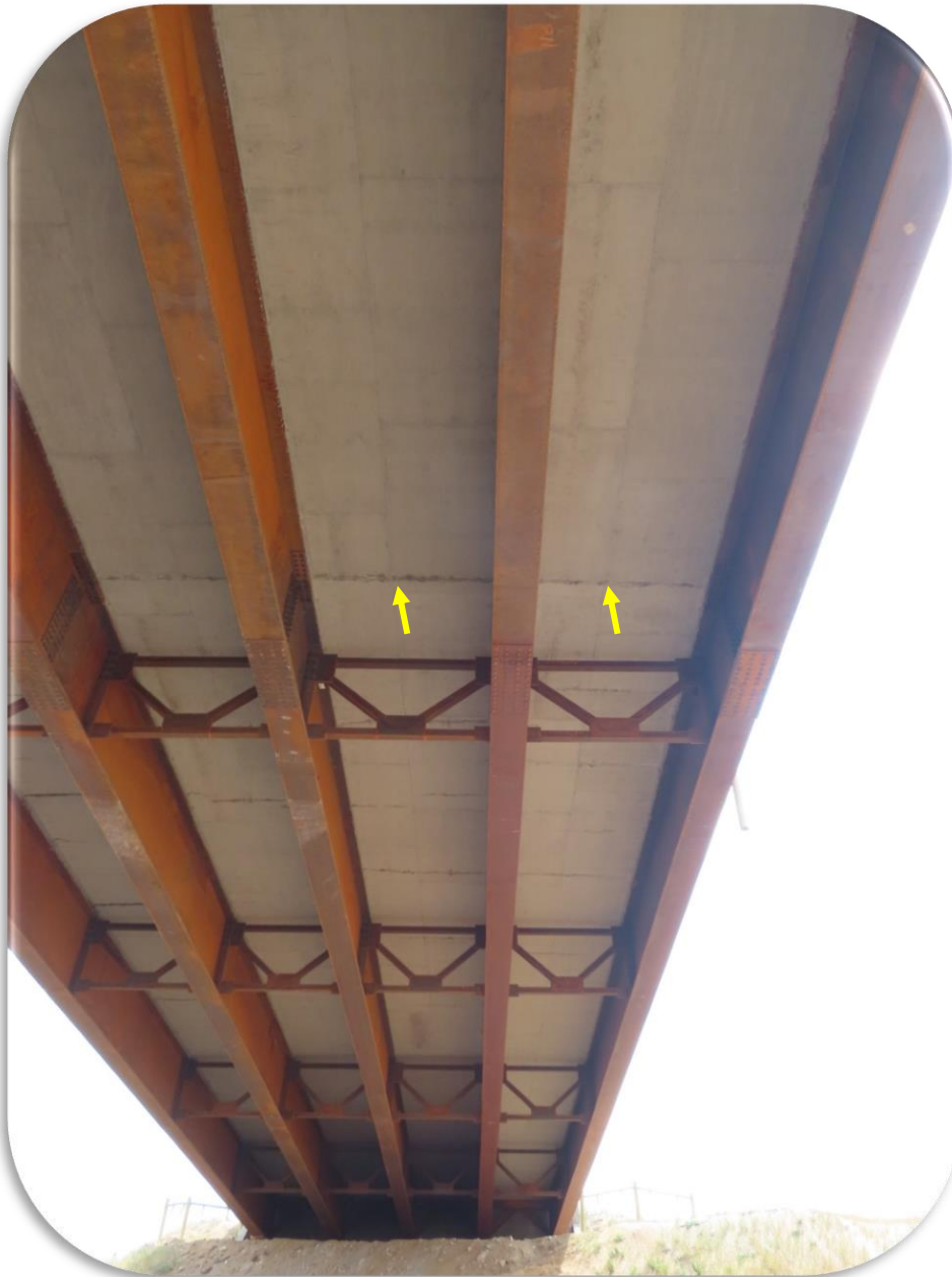
Figure 40. Underside of Rarus/Silver Bow Creek Bridge B - 2020 inspection - Span 1, Typical transverse crack at arrows.
