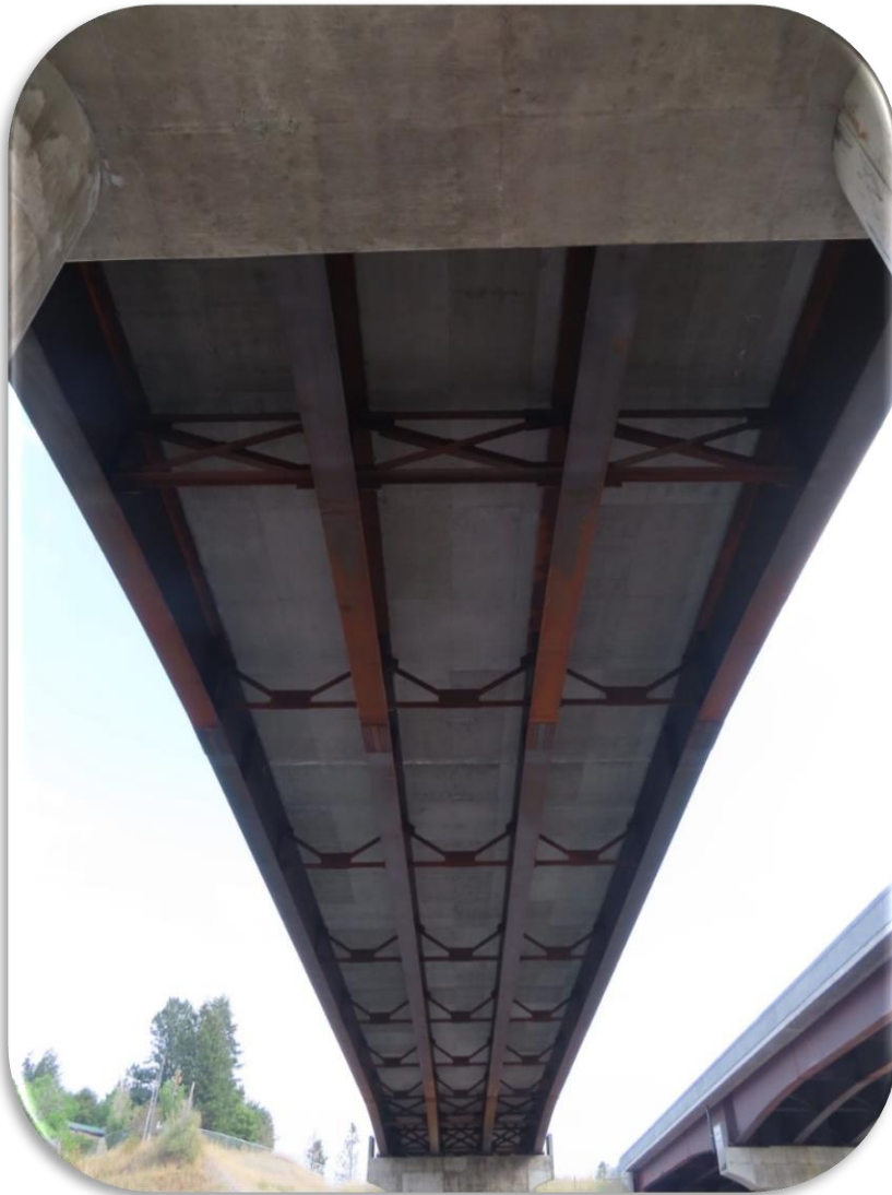
Figure 37. Bonner Bridge Phase II (WB) - 2020 inspection - Typical deck underside condition, Span 2 - Looking east.
