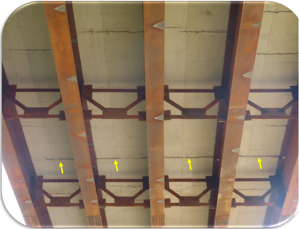
Figure 47. Underside of Rarus/Silver Bow Creek Bridge D - 2020 inspection - Span 3, Typical transverse crack at arrows.
