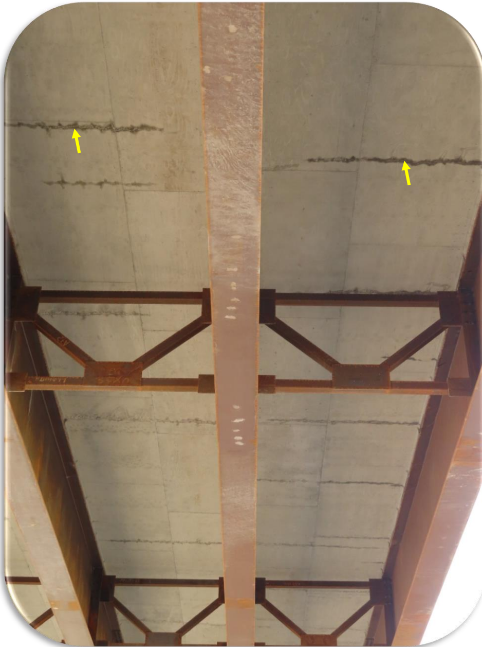
Figure 41. Underside of Rarus/Silver Bow Creek Bridge B - 2020 inspection - Span 2, Typical transverse cracks at arrows.
