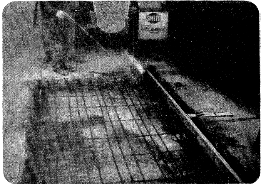
Figure 23. Spraying with water before placing concrete (note the side form being used).
