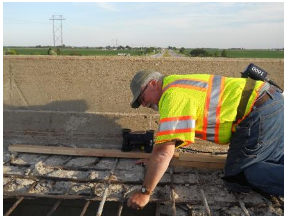
Figure 34. Gap shown in the bridge deck near an inspection site
