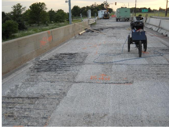
Figure 35. Amount of concrete removed during initial repair efforts
