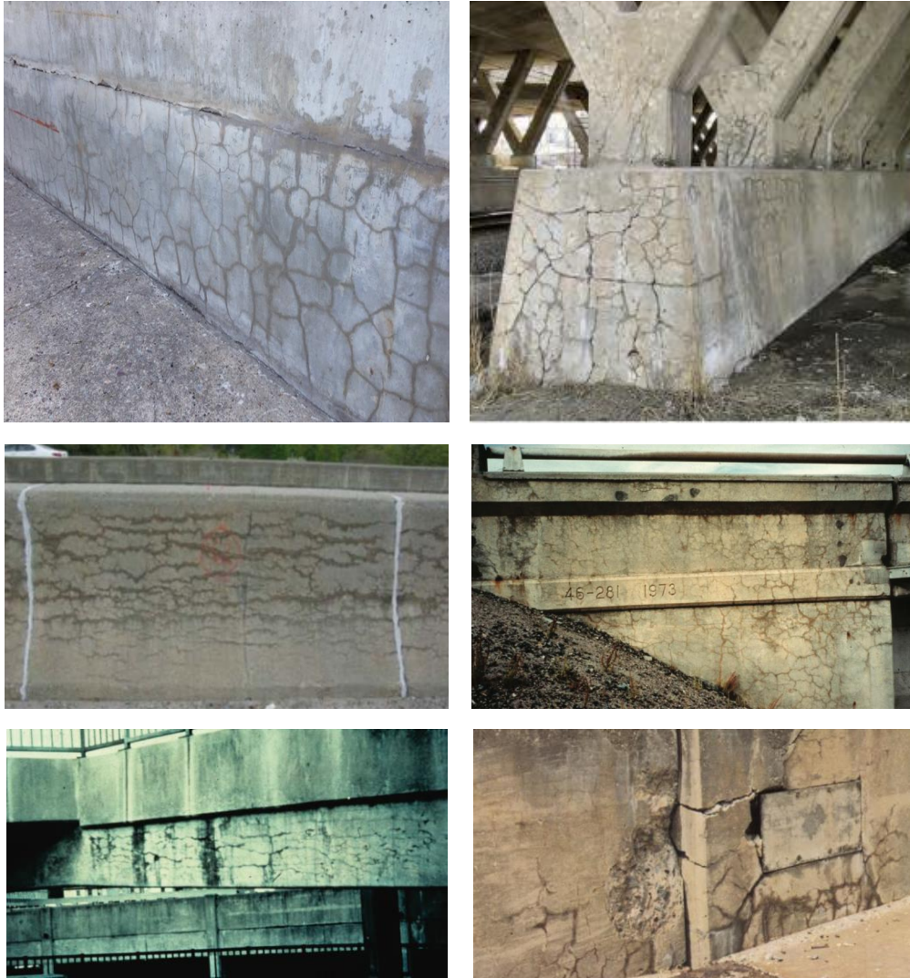
Examples of ASR Damage
