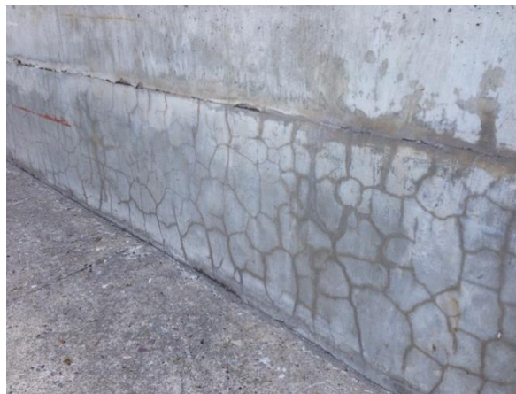
Figure 1: Typical ASR Crack Pattern
