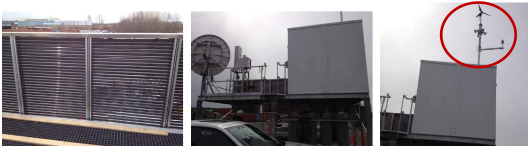
Figure 7. FAA remote WIS module, from left to right: thin-film solar PV tube array, control cabinet and satellite dish, and wind turbine and weather sensors
