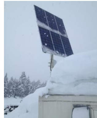
Figure 1. Power supplies at a remote RWIS site in Alaska, from left to right: overall site, 8340K-WG972 propane DC generator, and six Kyocera 120 solar PV modules
