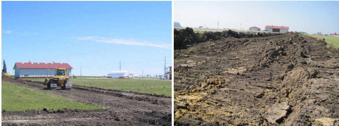
Figure 104. Removal of existing granular subbase and excavating to subgrade elevation on 5th St.
