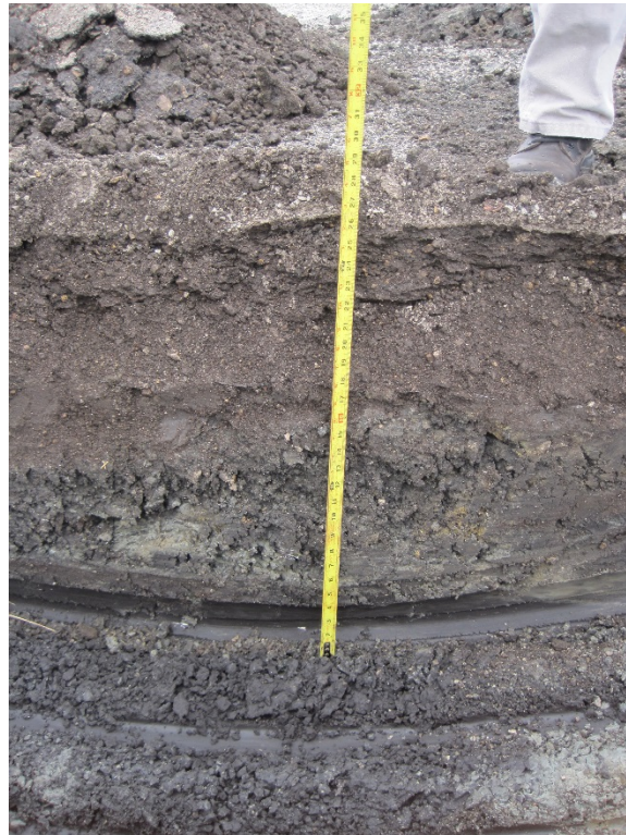
Figure 38. Pavement foundation layer profile from test pit observations on South Ave. (April 2012)
