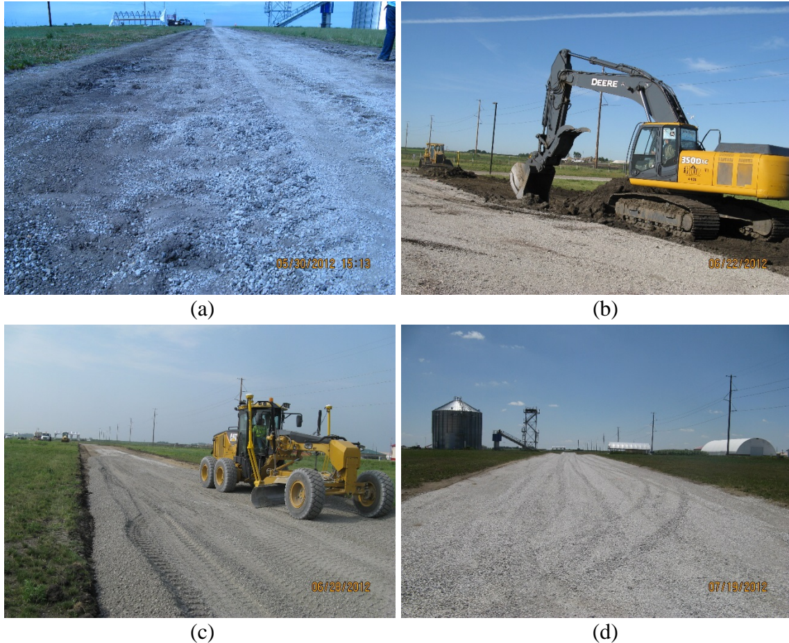
Figure 146. Construction operations on 8th St.: (a) existing subbase layer surface after IR passes, (b) excavating down to 6 in. below final grade to allow placement of MSB, (c) placement of crushed limestone MSB, and (d) 8th St. after placement and compaction of MSB
