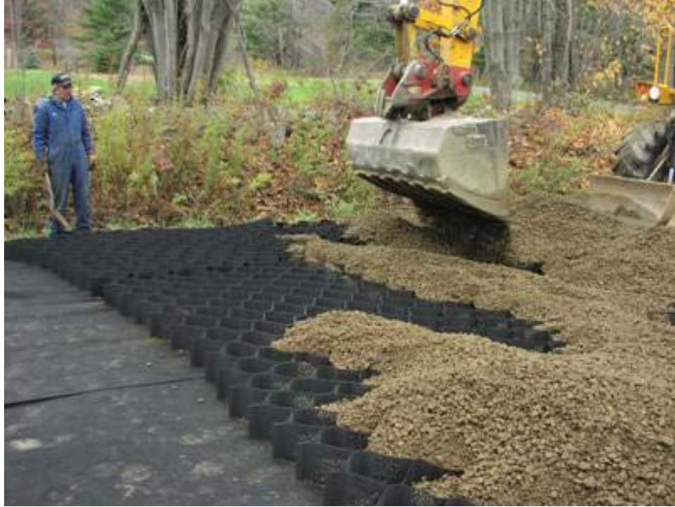
Figure 6. Geocells placed over non-woven geotextile on a test section in Vermont (Henry et al. 2005)
