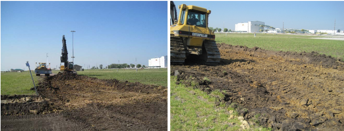
Figure 92. Removal of existing granular subbase and excavating to subgrade elevation on 4th St.
