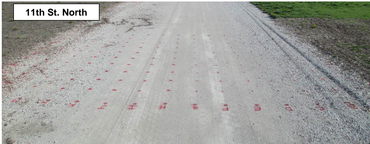
Figure 238. Photographs showing surface conditions during APT testing on the three test sections (May 2013)
