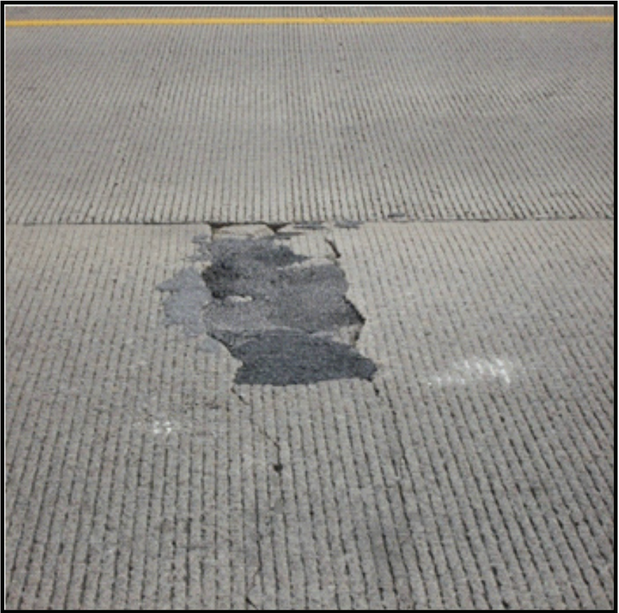
Figure 1. Partial depth distress near longitudinal construction joint
