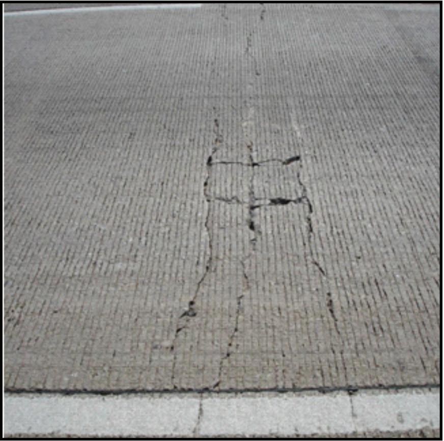
Figure 2. Partial depth distress under wheel path
