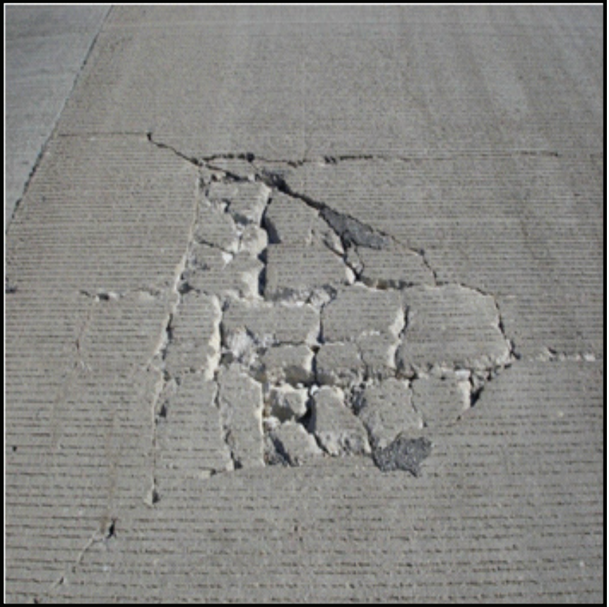
Figure 3. Partial depth distress under wheel path with fractured concrete
