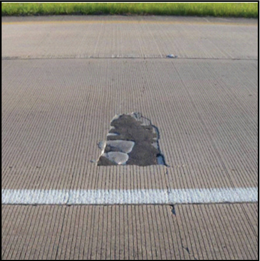
Figure 4. Partial depth distress under wheel path
