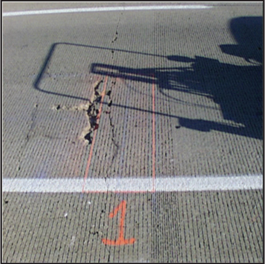
Figure 6. Partial depth distress under wheel path
