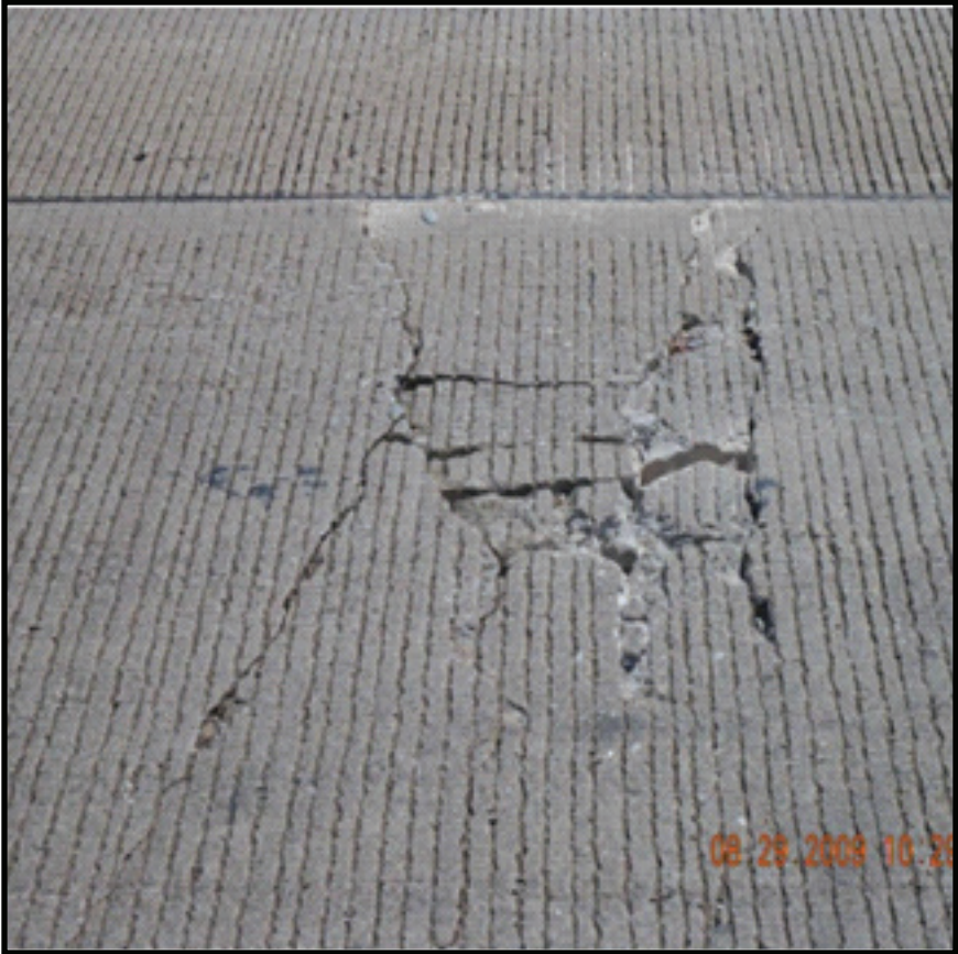
Figure 5. Partial depth distress under wheel path
