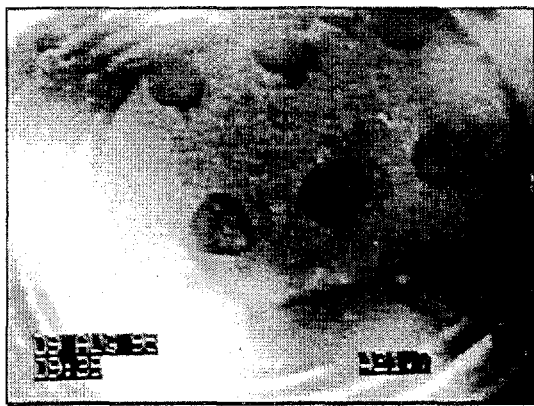
Here is a case where only the first 20 ft of the edgedrain was pipe. After this the edgedrain was an aggregate trench (French Drain). This individual wanted to keep the aggregate material out of the pipe so he used a brick as a stopper. Yet he wanted the aggregate trench to drain into the pipe so he used a brick with holes in it.
