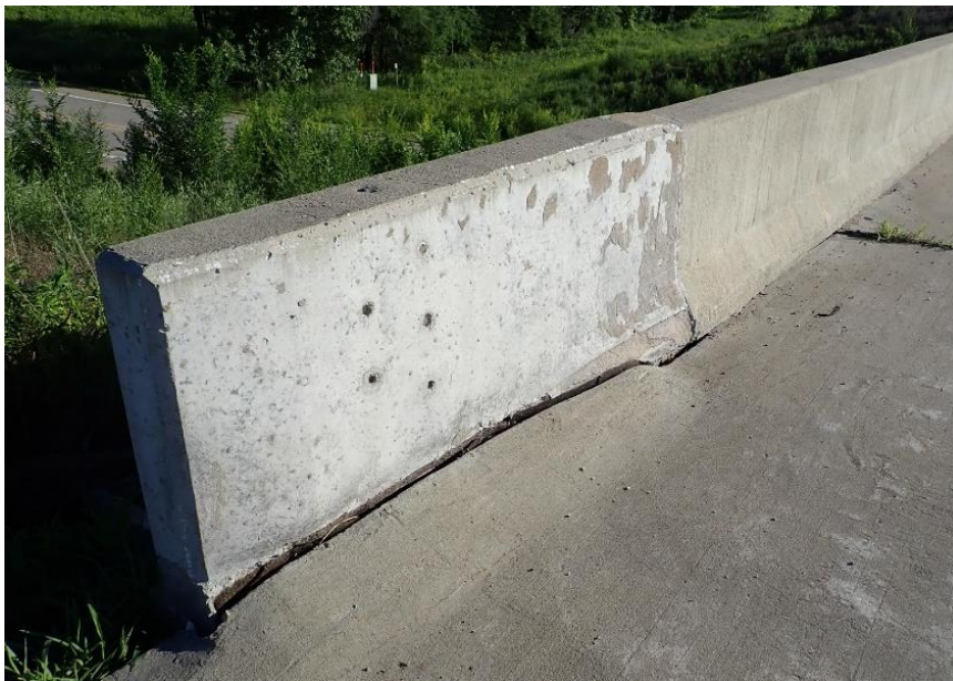
Figure 3.48. Gap between west barrier and shoulder at south approach of Bridge 5617.7L061, note effort to construct a curb along this joint.
