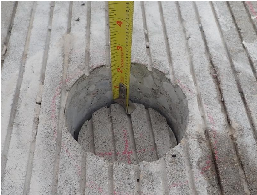
Figure 3.30. Measurement of void (2.0inch) underneath Core 4 of Bridge 5622.50061.
