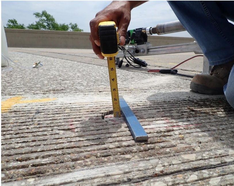
Figure 3.12. View of core drop (1/4 inch) indicating presence of minor void under the slab.
