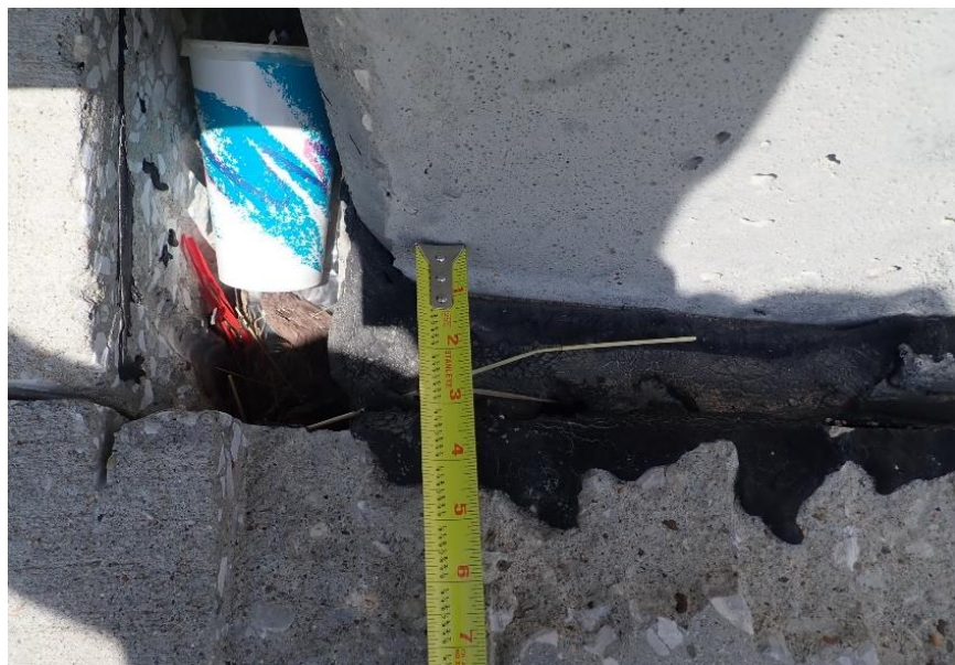
Figure 3.49. Debris in gap between shoulder and north barrier at west approach of Bridge 5622.50061.
