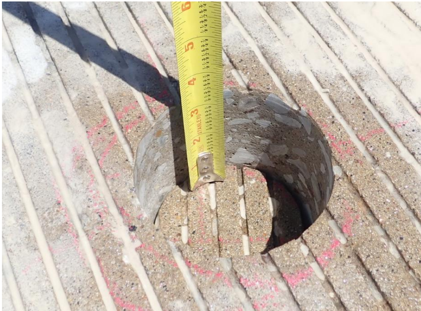
Figure 3.39. Measurement of void underneath Core 3 of Bridge 5624.20061.
