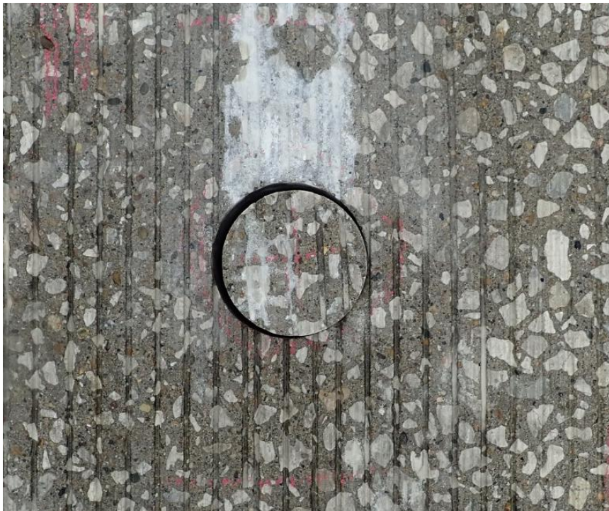
Figure 3.28. View of Core 2 of Bridge 5622.5O061 (no void).
