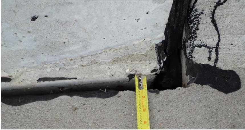
Figure 3.47. Gap between south barrier and shoulder of west approach of Bridge 5627.1O061.
