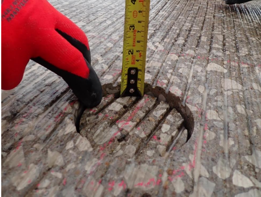
Figure 3.27. Measured drop (0.5inch) of Core 1 of Bridge 5622.5O061.
