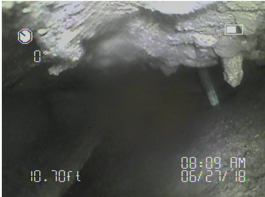
Figure 3.44. Void under north approach from Bridge 5617.7L061.
