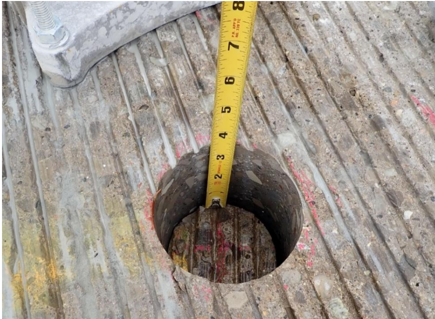
Figure 3.18. Measured drop (3.5 inches) of Core 1 of Bridge 5126.5S078.
