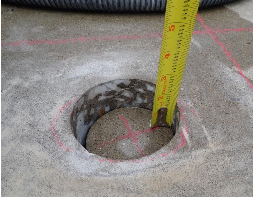
Figure 3.29. Measurement of void (1.5inch) underneath Core 3 of Bridge 5622.50061.
