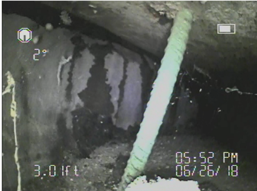
Figure 3.45. Void under east approach from Bridge 5657.40002.
