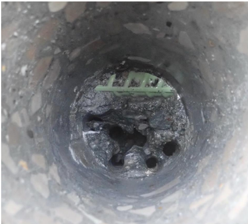
Figure 3.19. Epoxy-coated rebar and voids found under Core 2 of Bridge 5126.5S078.
