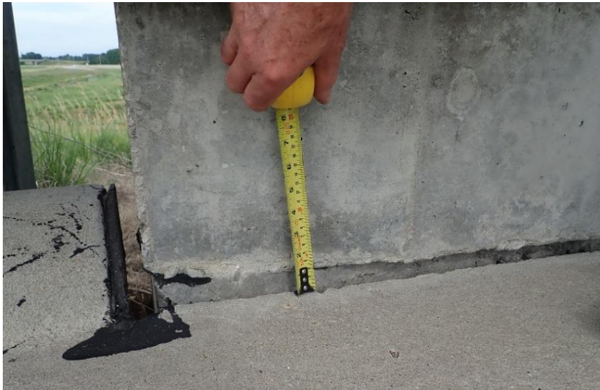
Figure 3.46. Gap between north barrier and shoulder at west approach of Bridge 5627.1O061.
