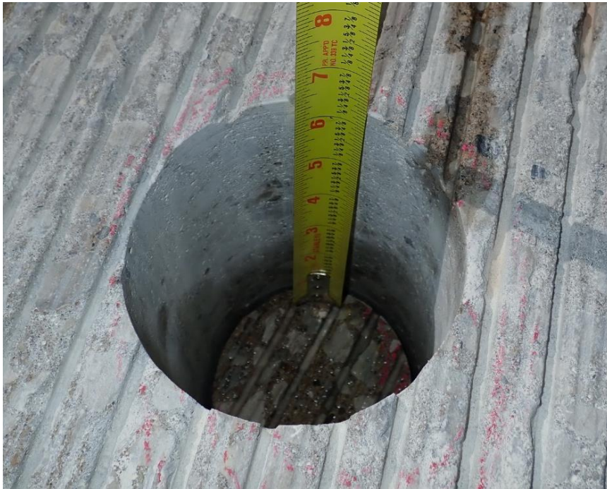
Figure 3.38. Measurement of void underneath Core 2 of Bridge 5624.20061.
