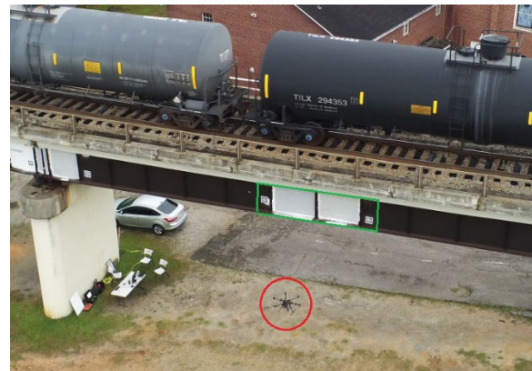
Figure 1. UAS performing DIC measurements on a CSX railroad bridge at Park St., Columbia, SC (the drone is highlighted in the red circle and the speckled area in the green rectangle)
