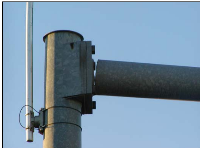
Figure 1.3 Fatigue Failure of Mast Arm in Lubbock, Texas
