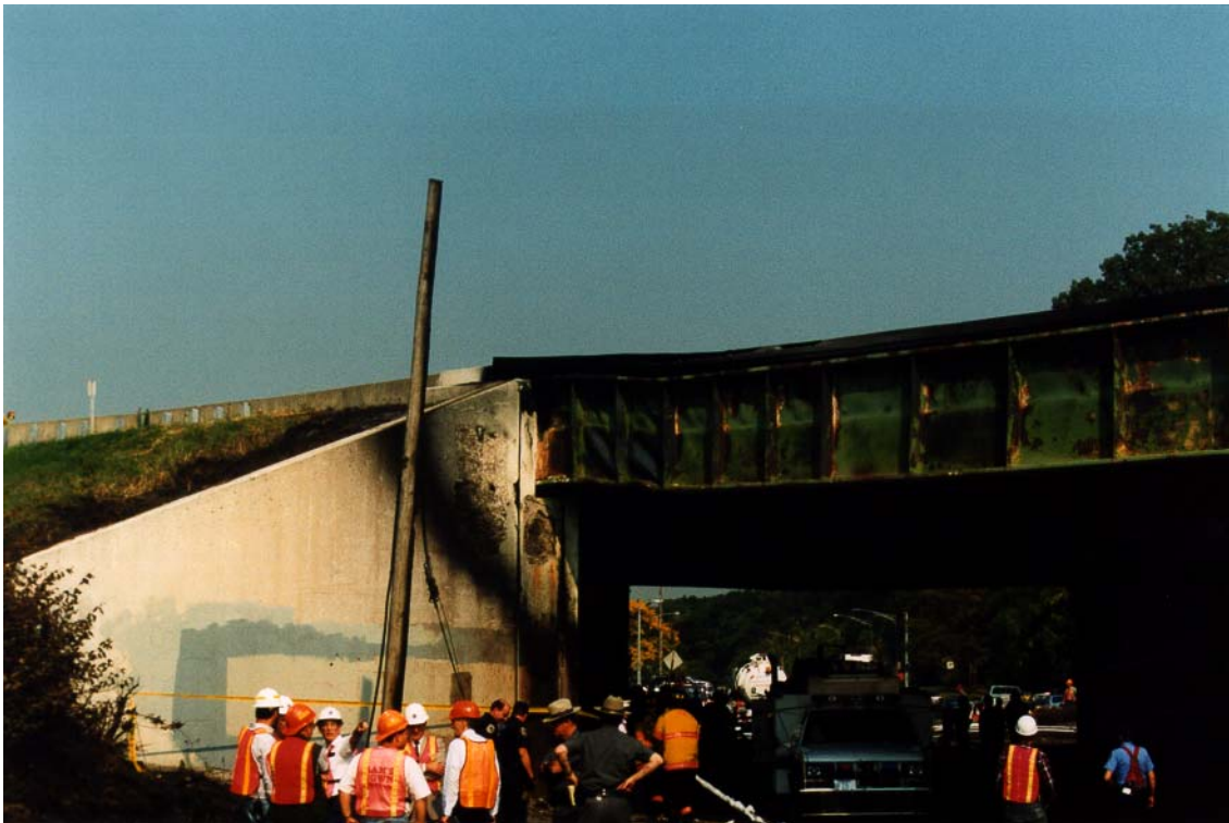
Figure 1 Damaged Bridge in Yonkers (provided by NY State Thruway Authority)
