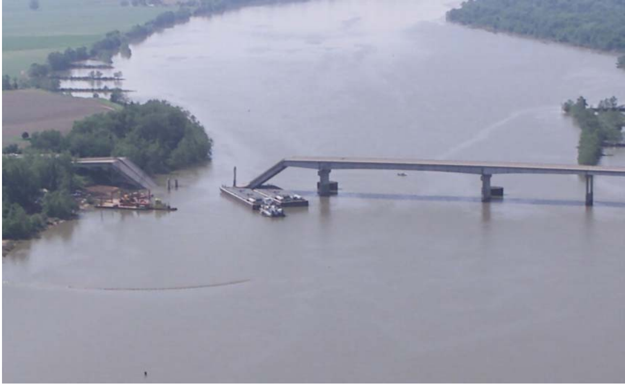
Figure 2 Overview of the Damaged Bridge (Provided by ODOT)
