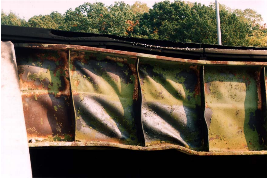
Figure 2 Damaged Bridge in Yonkers (provided by NY State Thruway Authority)
