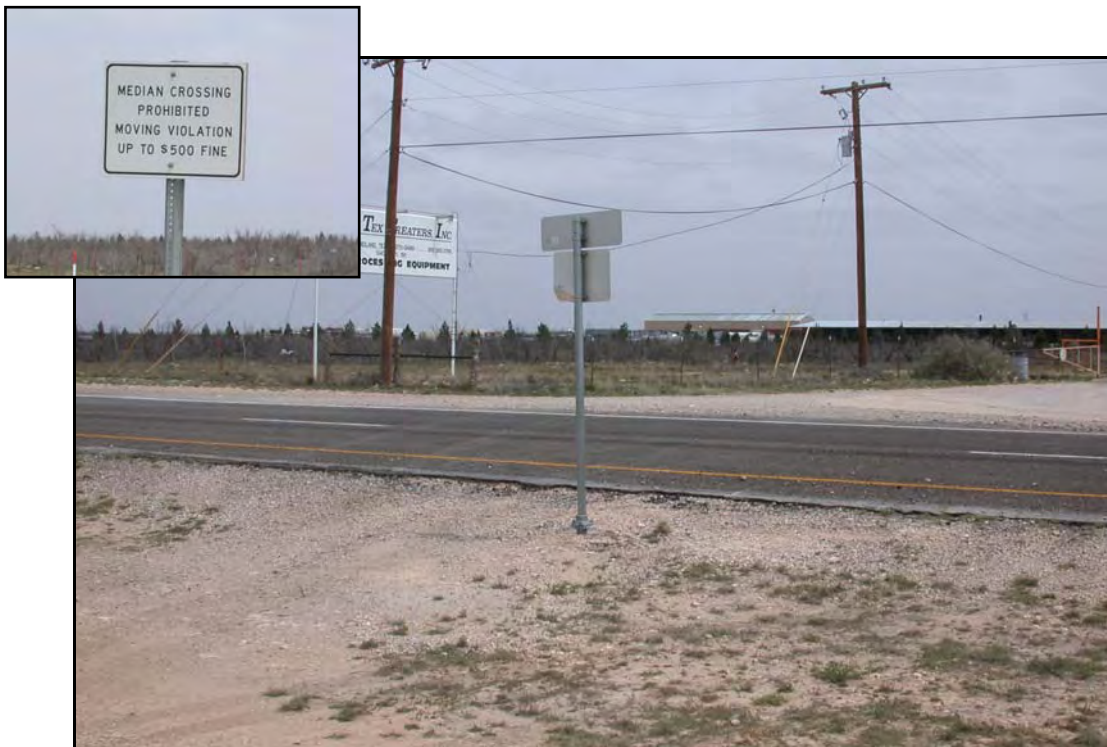
FIG. 4.17. Pavement Edge Damage Associated with Illegal Median Crossing. The Inset Shows the Regulation Sign Posted Where the Crossing Continues to Occur
