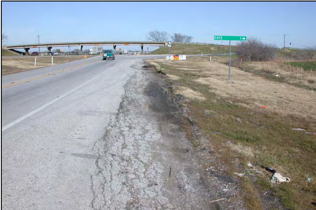
FIG. 4.10. Edge Damage Along Interstate Highway Access Road.
