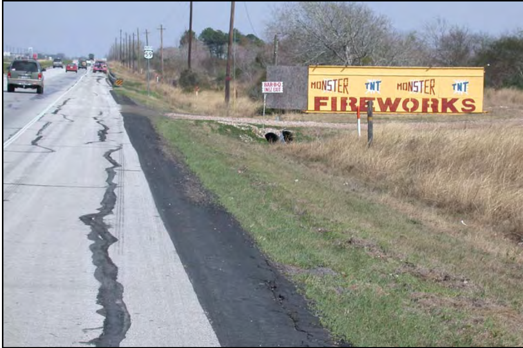
FIG. 4.21. Typical Edge Damage at Location of Roadside Vendor.
