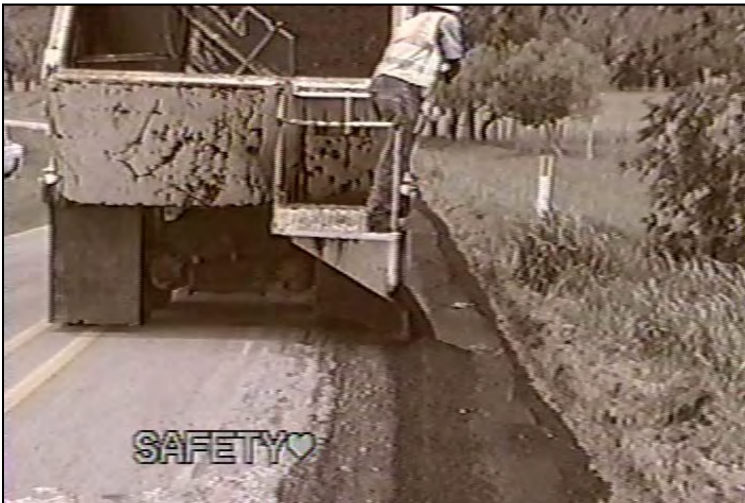
FIG. 7.12 Side-Discharge Tailgate Chute, Waco District (see Waco District Profile, Photo 7)
