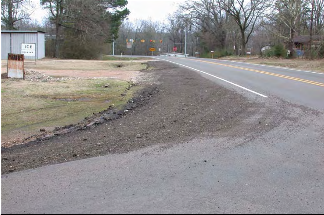
FIG. 4.12. Typical Edge Drop-off at Turning Radius (Maintained by placing RAP).
