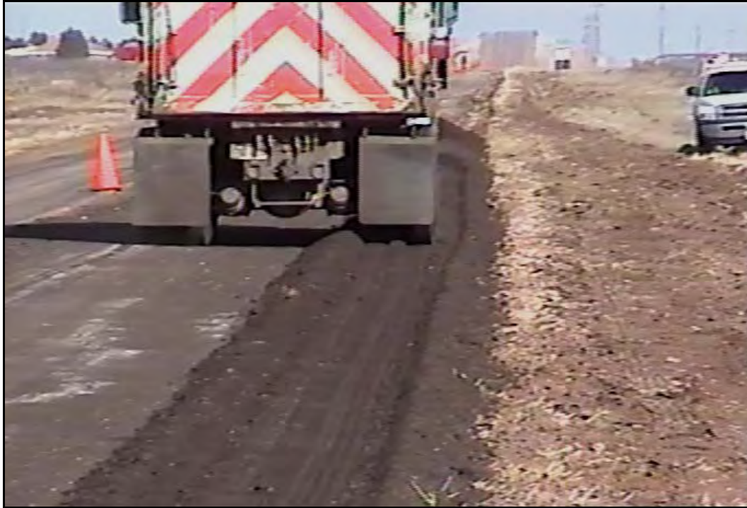
FIG. 5.28 District Forces Use Dump Truck Tires to Achieve Ordinary Compaction for Edge Repair, Amarillo District
