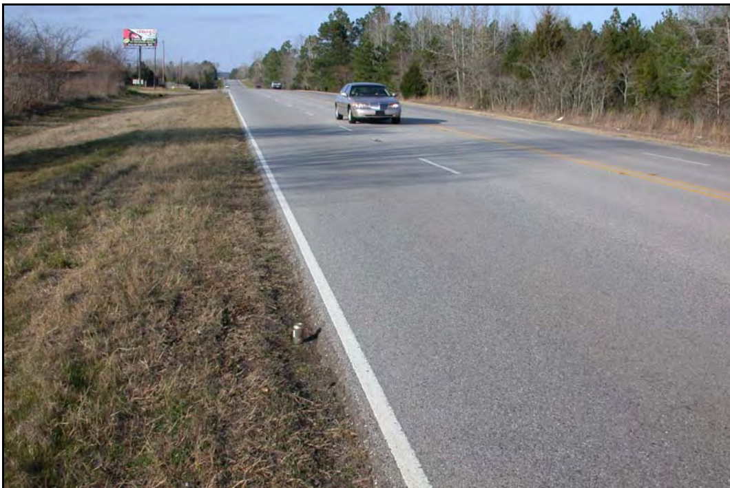
FIG. 4.7. Edge Drop-off Along a Narrow 4-Lane US Highway (“Poor-Boy” 4-Lane).
