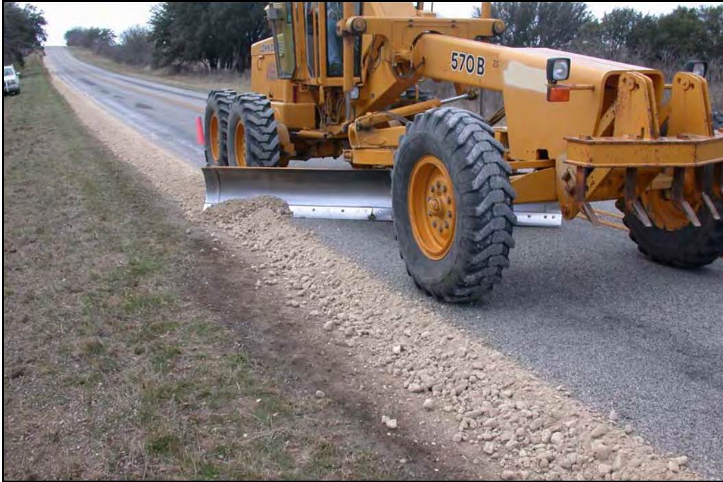
FIG. 5.32 Flex Base for Pavement Edge Repair, Brownwood District, (see Brownwood District Profile, Photograph 15)
