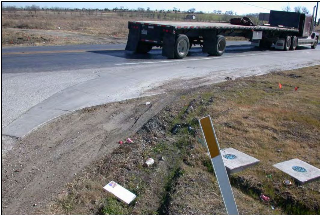
FIG. 4.20. Edge Damage Caused by Cutting Corners at a Convenience Store Access Drive.
