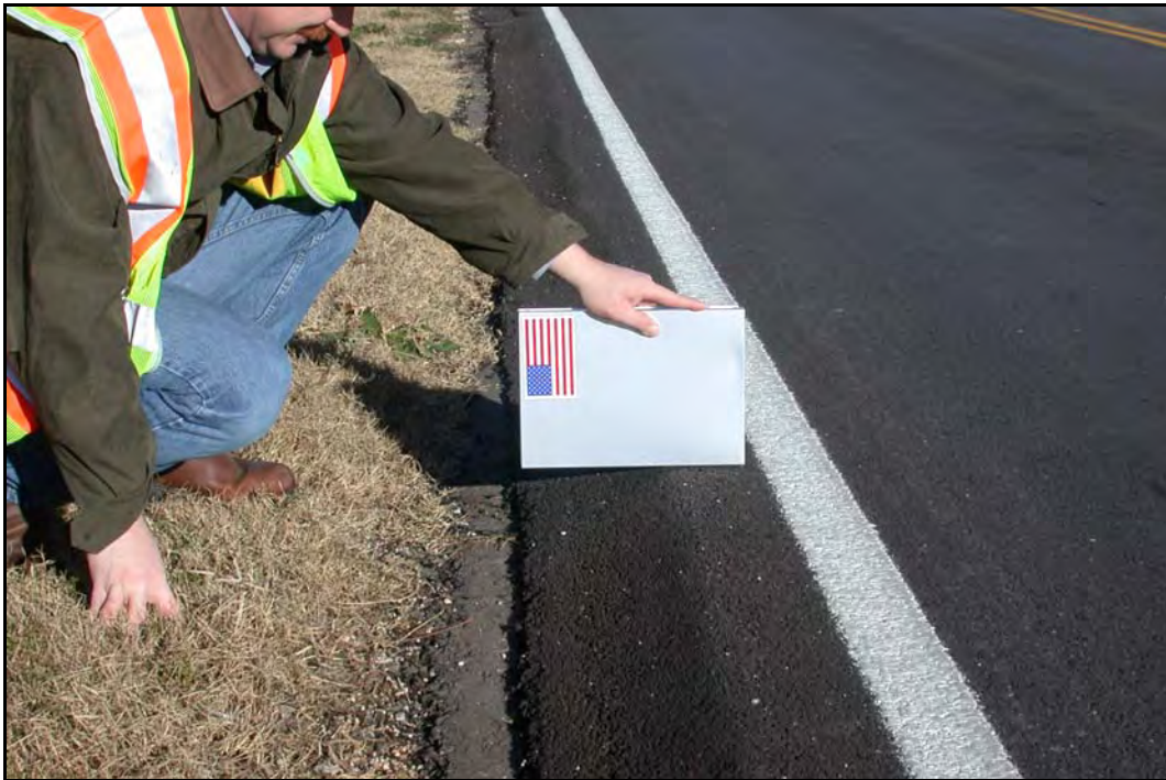
FIG 5.5 Tapered Edge Detail to Reduce Edge Drop-offs Following a Full-Width Overlay, Fort Worth District (see Fort Worth District Profile, Photo 8)
