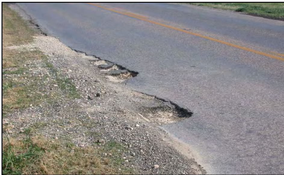
FIG 5.22 Fishmouth-type Edge Failure, San Antonio District (see San Antonio District Profile, Photo 12)
