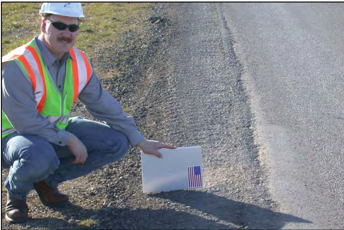
FIG. 7.35 Completed Edge Repair Project Using Midland Machinery Road Widener, Fort Worth District (see Fort Worth District Profile Photo 43)
