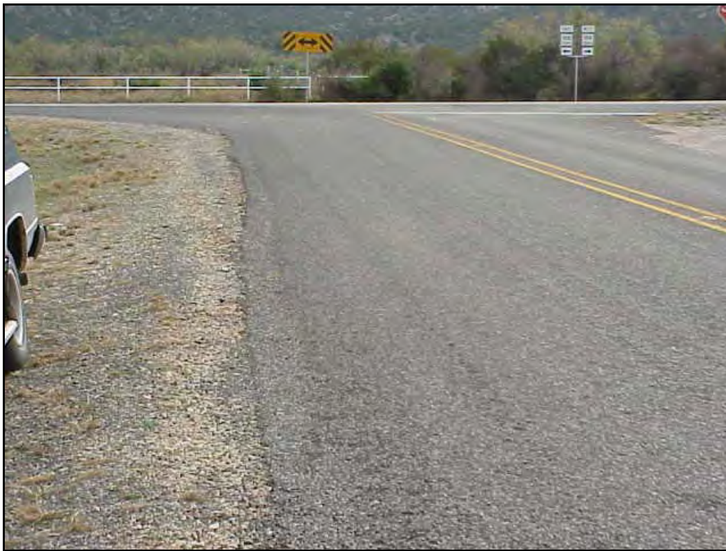
FIG 5.11 Intersection Approach Apron, San Angelo District (see San Angelo District Profile, Photo 5)
