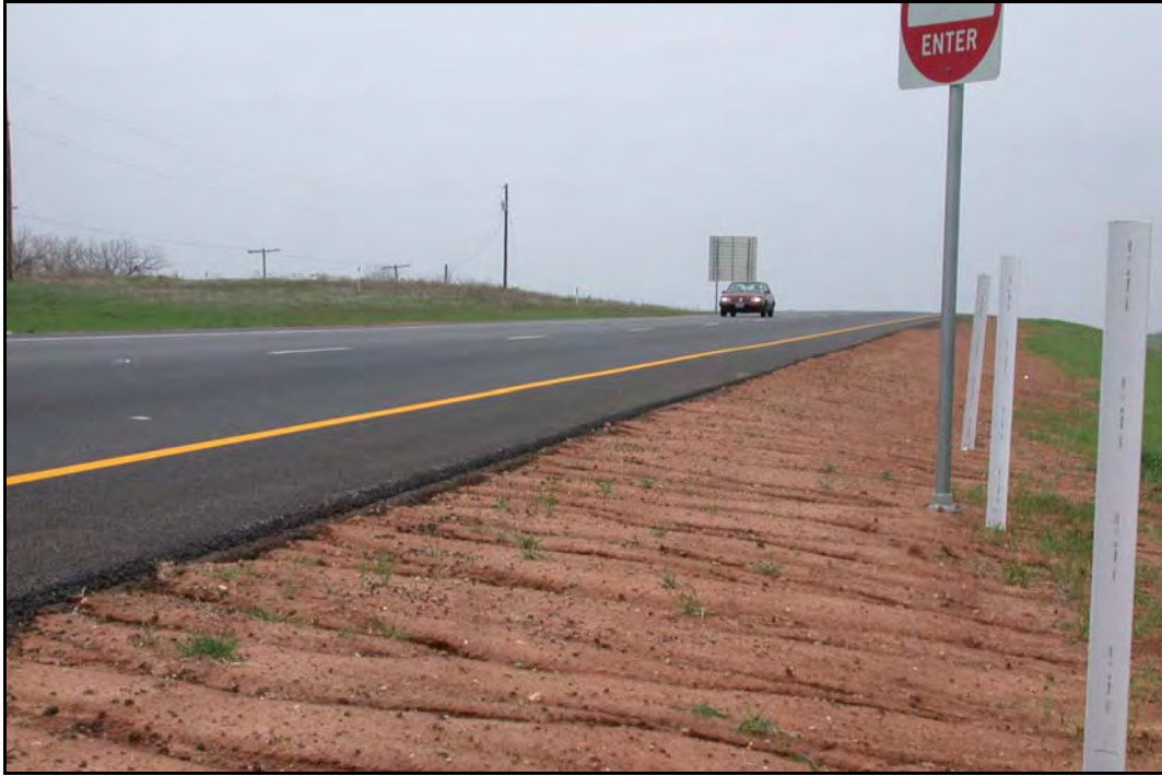
FIG 5.6 Soil Erosion of Pavement Edge Backfill due to Improper Specification, Wichita Falls District (see Wichita Falls District Profile, Photo 7)
