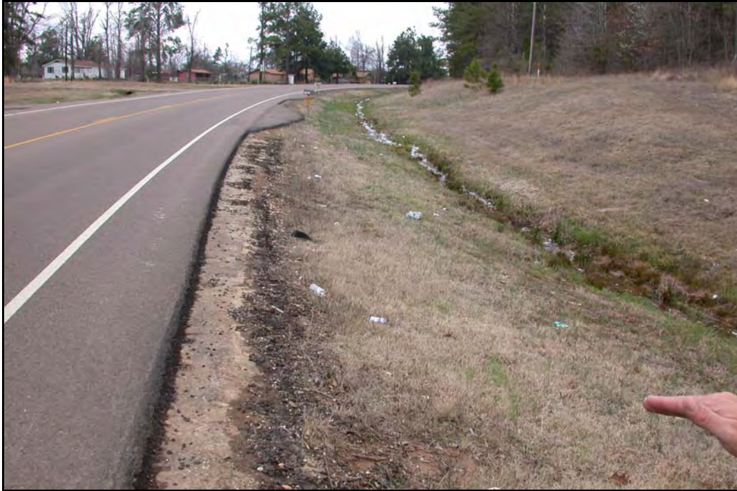
FIG 5.13 Erosion-induced Edge Drop-off Following an Overlay, Atlanta District (see Atlanta District Profile, Photo 11)
