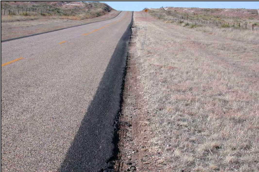
FIG. 4.13. Typical Edge Drop-off at Approach to Uphill Vertical Curve.
