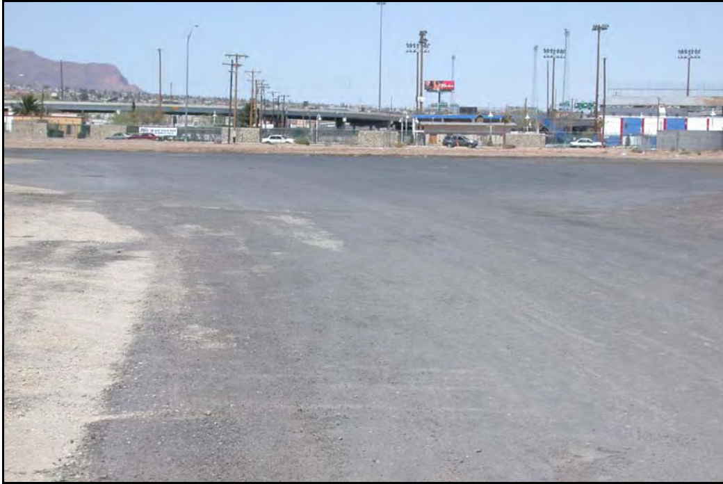
FIG. 5.31 US Customs Truck Parking Lot, RAP Treated with Magnesium Chloride, El Paso District, (see El Paso District Profile, Photograph 23)
