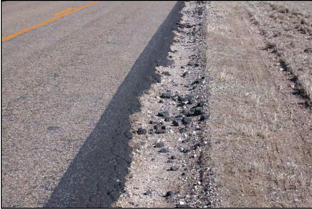
FIG. 4.22. Typical Edge Damage on a Low Volume Road Caused by Snow Plow Operations.
