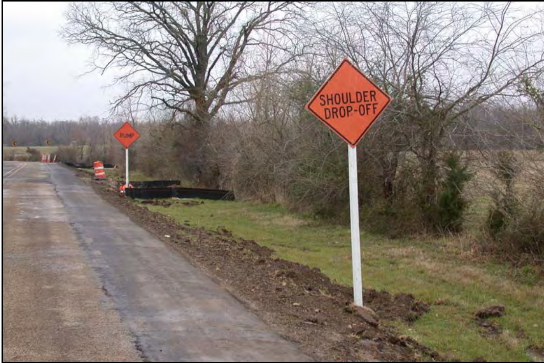
FIG 5.17 Shoulder Drop-off Sign, Construction Project, Paris District (see Paris District Profile, Photo 34)
