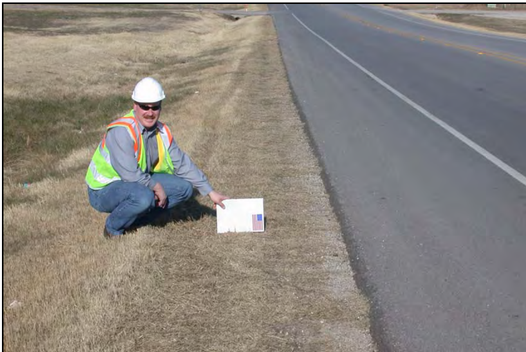
FIG. 4.19. Typical Edge Damage Associated with Illegal Left-Turn Bypass Maneuver.
