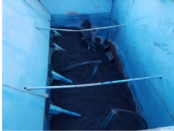
Figure 6-2. View inside ECR feeder Unit showing pugmill-style agitation system
