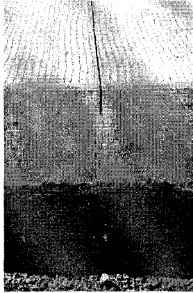
Figure 50 – Traverse crack at form edge
