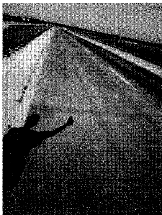
(a) Staining along longitudinal cracks
