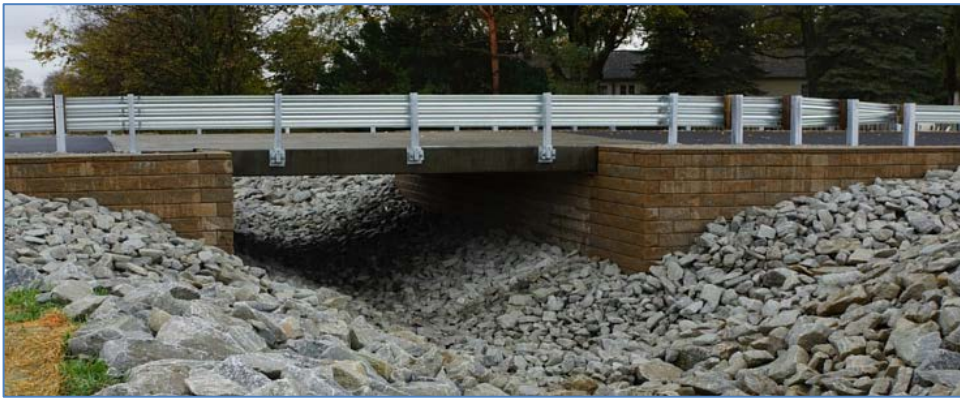
Figure 7 A bridge built using the GRS-IBS methodology
