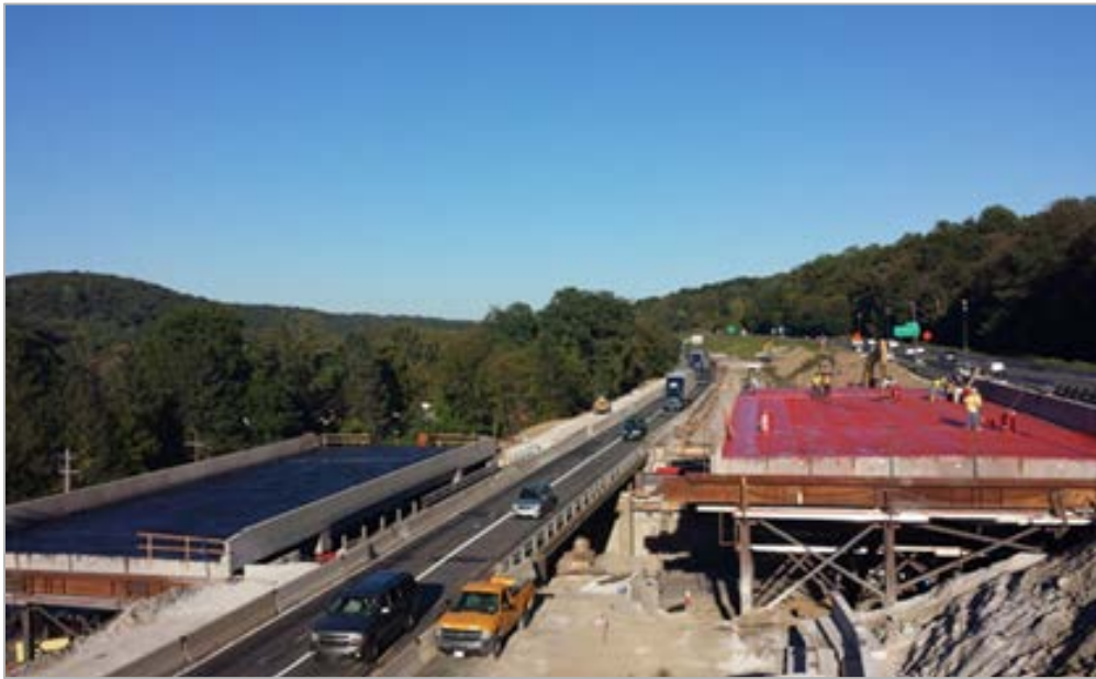
Figure 1 Dingle Ridge Road bridge replacement project using slide-in bridge construction method (New York State), Photo by FHWA
