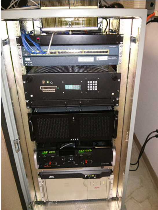
Figure 12 AGHME rack containing a cooling unit, power supplies, network and maintenance components, main computer which houses the 1090MHz message decoding board set, and GPS unit
