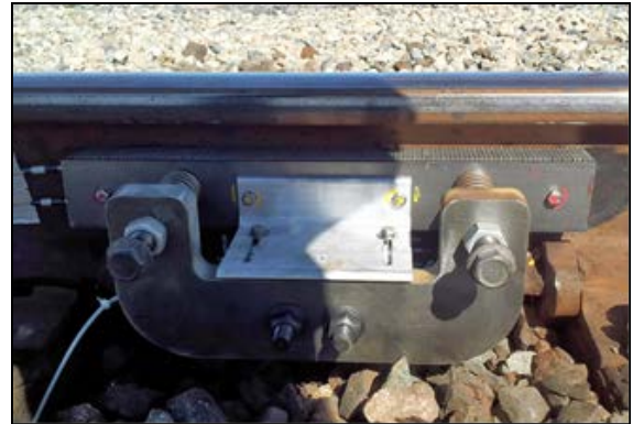
Figure 13 The Rail-NT sensor head installed on a rail.
