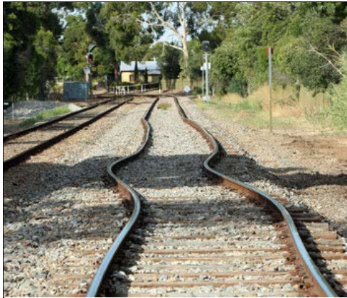
Figure 12 Buckling of a CWR.
