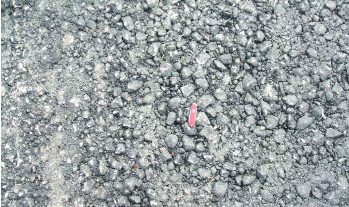
Figure 11-10. Area of excessive coarse aggregate due to end of load segregation.
