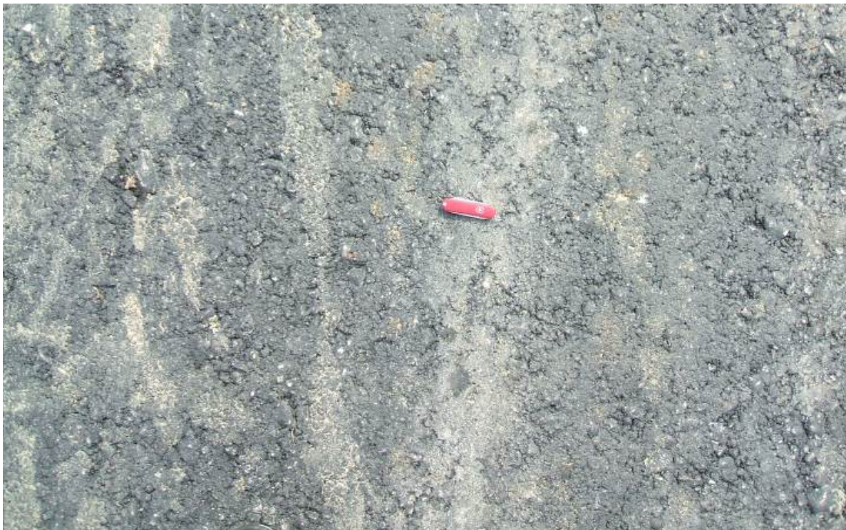
Figure 11-9. Area of excessive fine aggregate due to end of load segregation.
