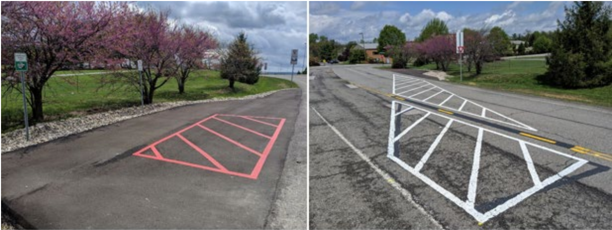
Figure 9. Views of the constructed pulloff and loading area (left) and travel lane crossing zone installed near the Blacksburg Transit bus stop.
