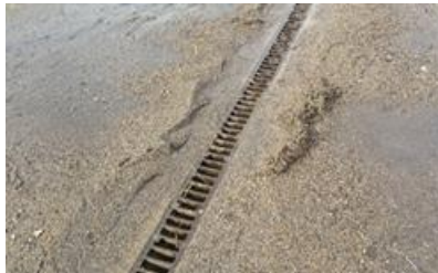
Figure 2.9. Debris cleaned from the drain
