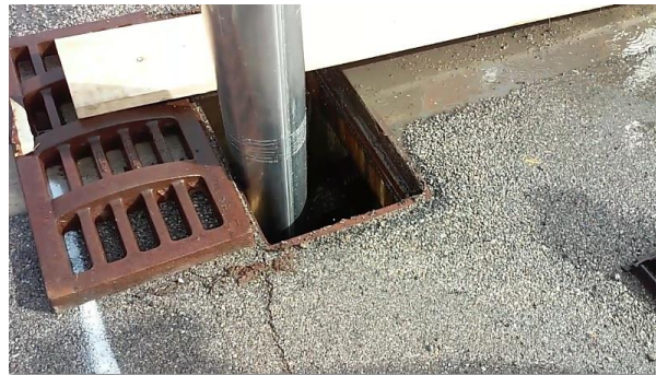
Figure 2.14. Suction tube placed in catch basin
