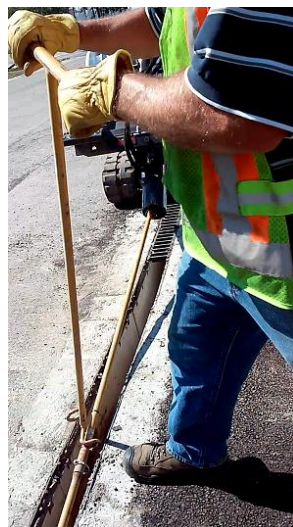
Figure 5.27. Manually applying pressure on drill rods to push augers to the bottom of the drain
