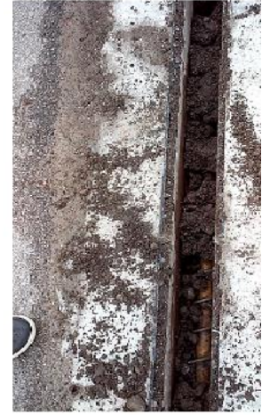
8-Auger flights convey the material back to the cleanout location
