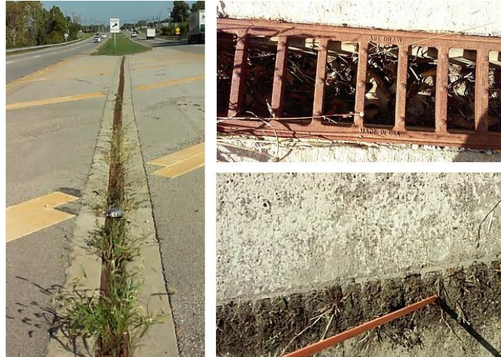
Figure 2.2. Debris and vegetation in trench drains
