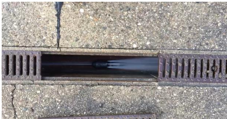
Figure 5.16. Drainage channel nozzle inside trench drain
