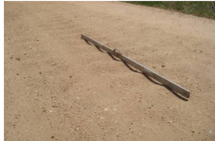
Figure 18. Washboarding, or corrugation, on dirt road (Jones and Paige-Green 2015).
