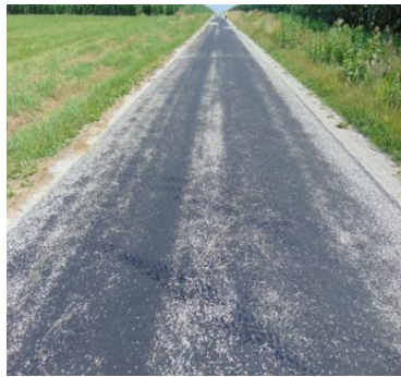
Figure 10. Bleeding of asphalt binder in seal-coated road.
