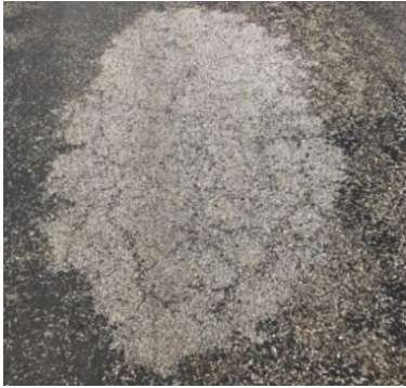
(a) Patch deterioration with cracks
