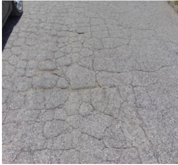
(a) Fatigue, or alligator, cracks
