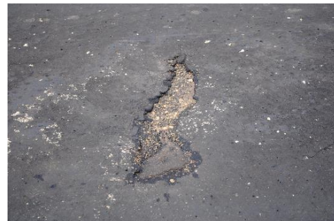
(b) Pothole associated with chip loss
