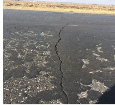
(b) Transverse cracks
