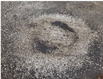
Figure 12. Chip loss in a seal-coated road.
