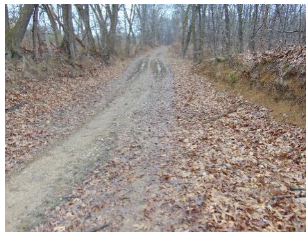
Figure 5. Typical dirt road.
