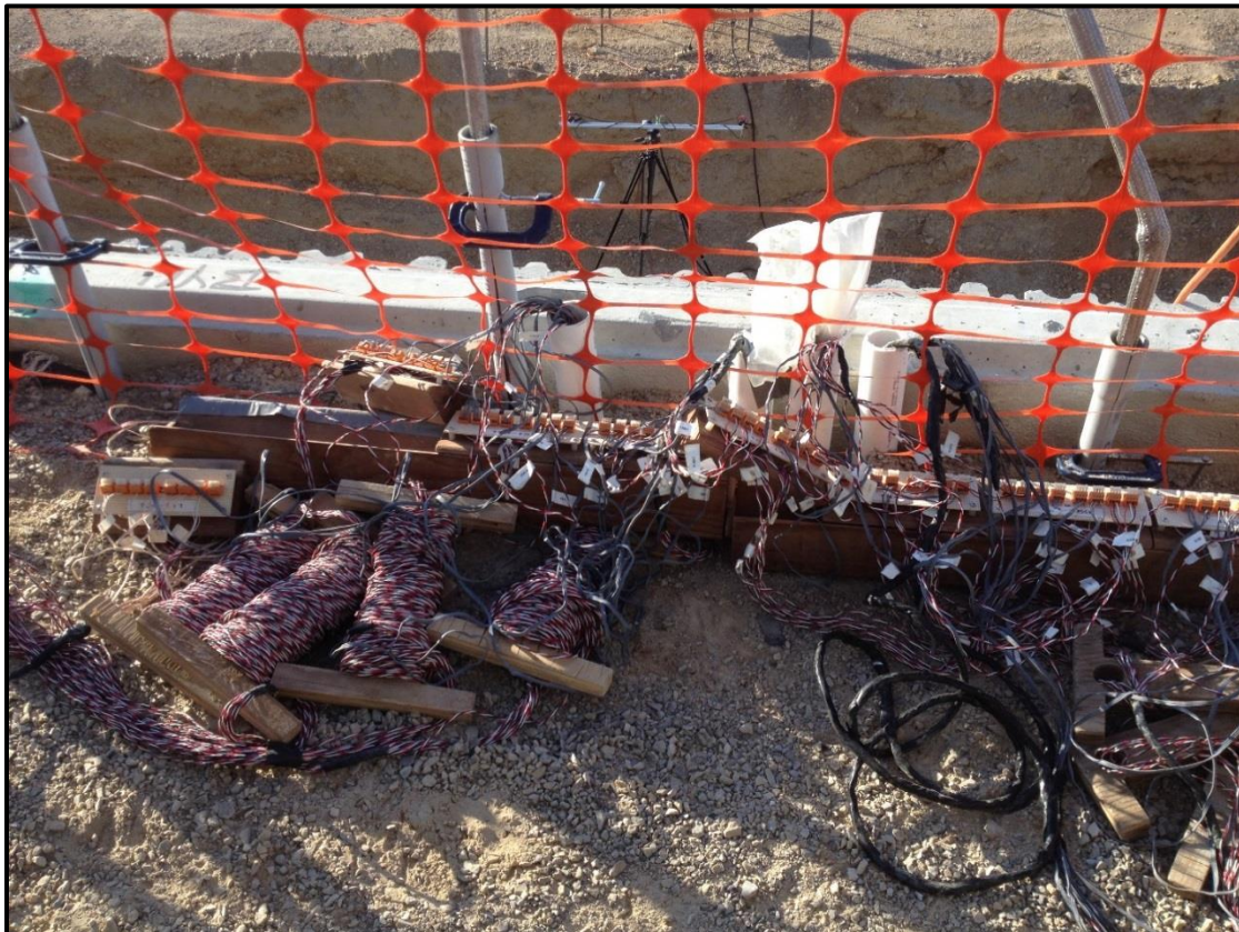
Figure 4-4: Strain gauge connections to terminal strips.
