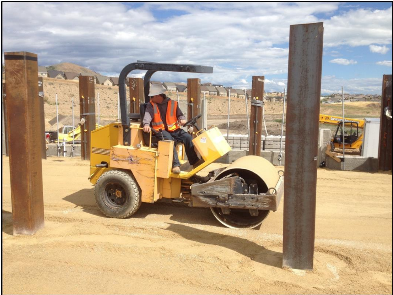
Figure 3-12: Compaction of backfill behind the test piles using a vibratory roller compactor.
