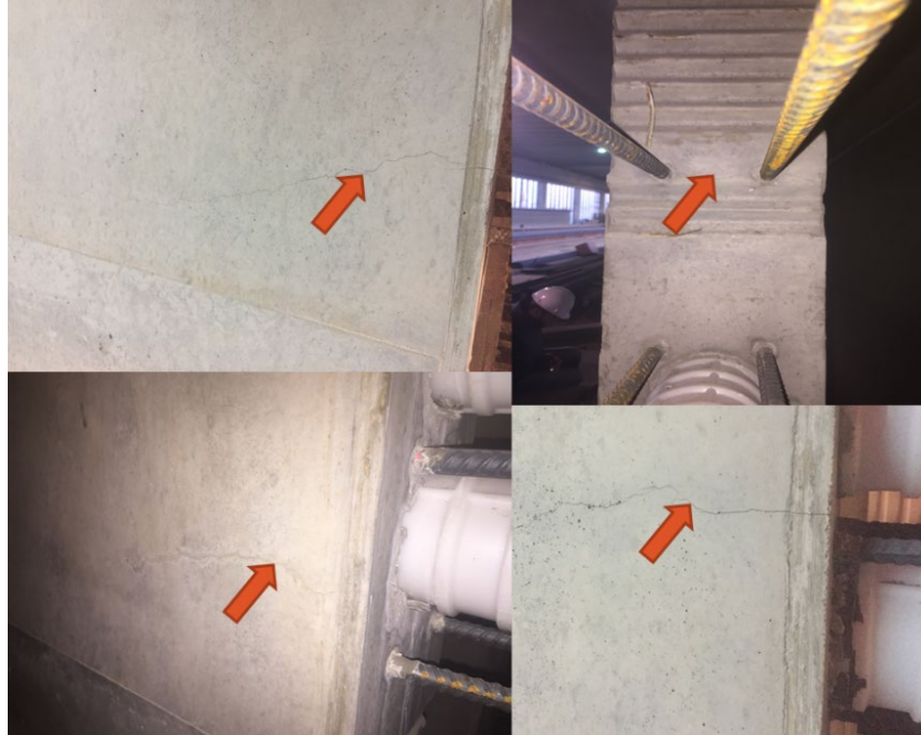
Figure 1.3: Recorded end zone cracking of bulb tee
