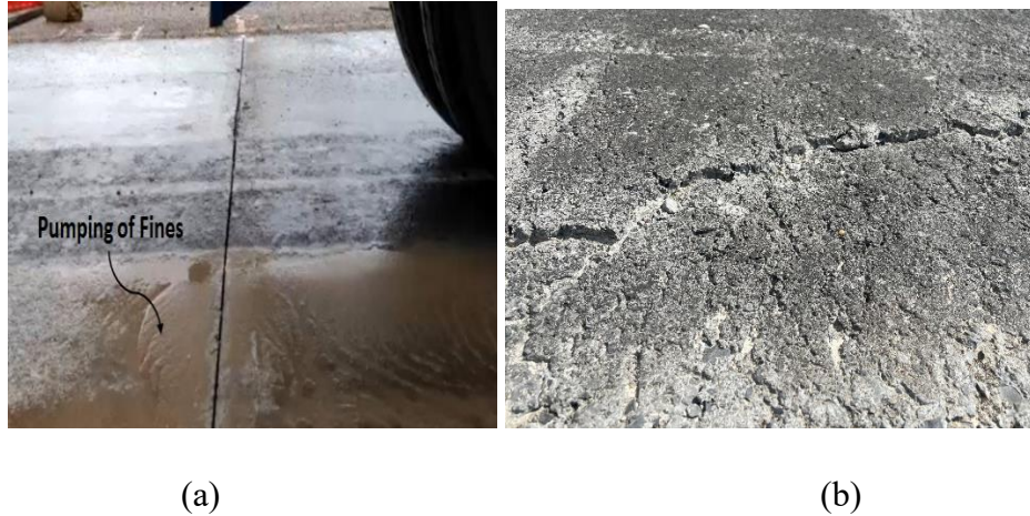
Figure 21. (a) Observed pumping (b) Observed slab settlement
