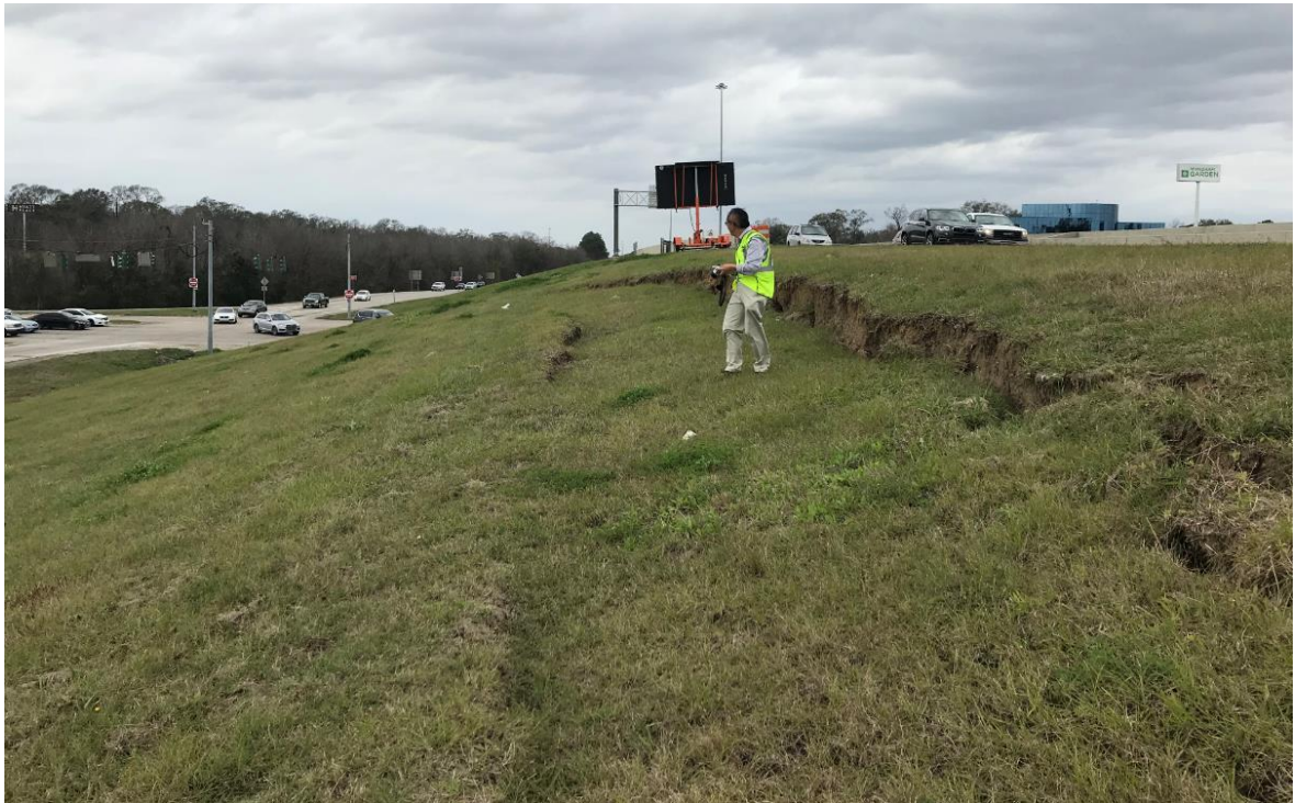
Figure 4. Interstate 10 at Bluebonnet Boulevard slope failure, 2019
