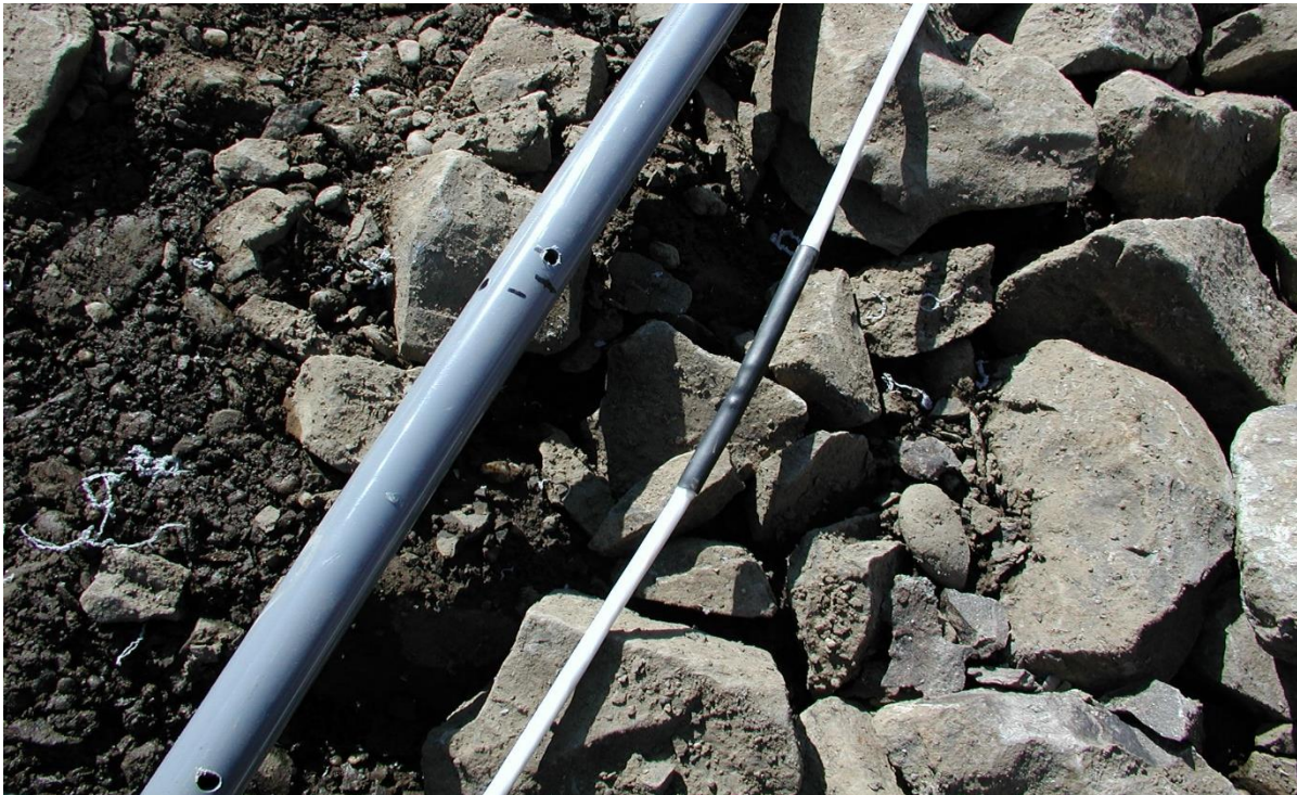
Figure 3-2 Thermistor sensor wire and vented PVC armoring tube as used in ACE areas
