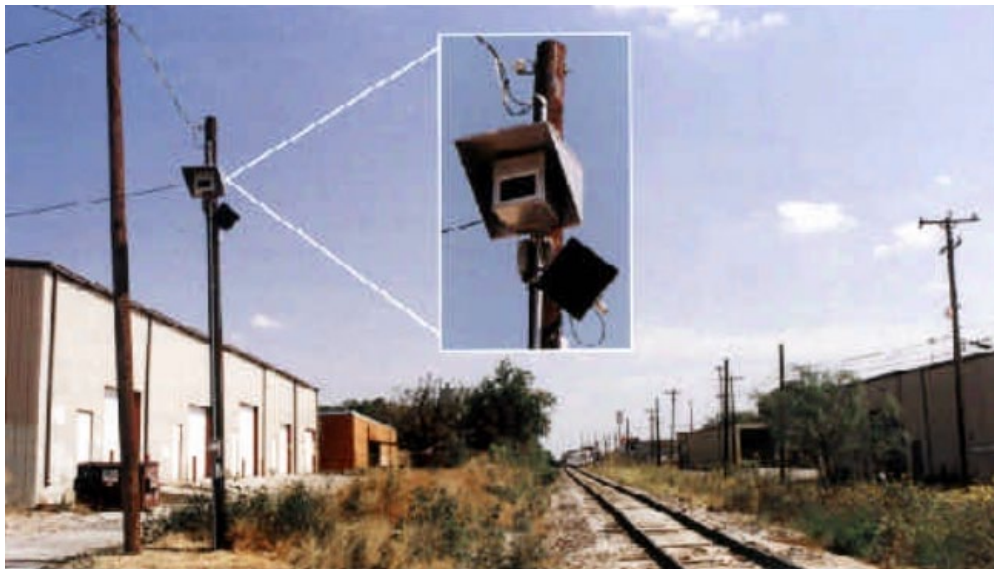
Figure 2.11 AWARD site installation to collect train information (Carter et al. 2000)
