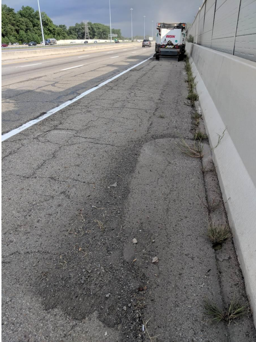
Figure 8.3 Debris left by inadequate down pressure on gutter brush
