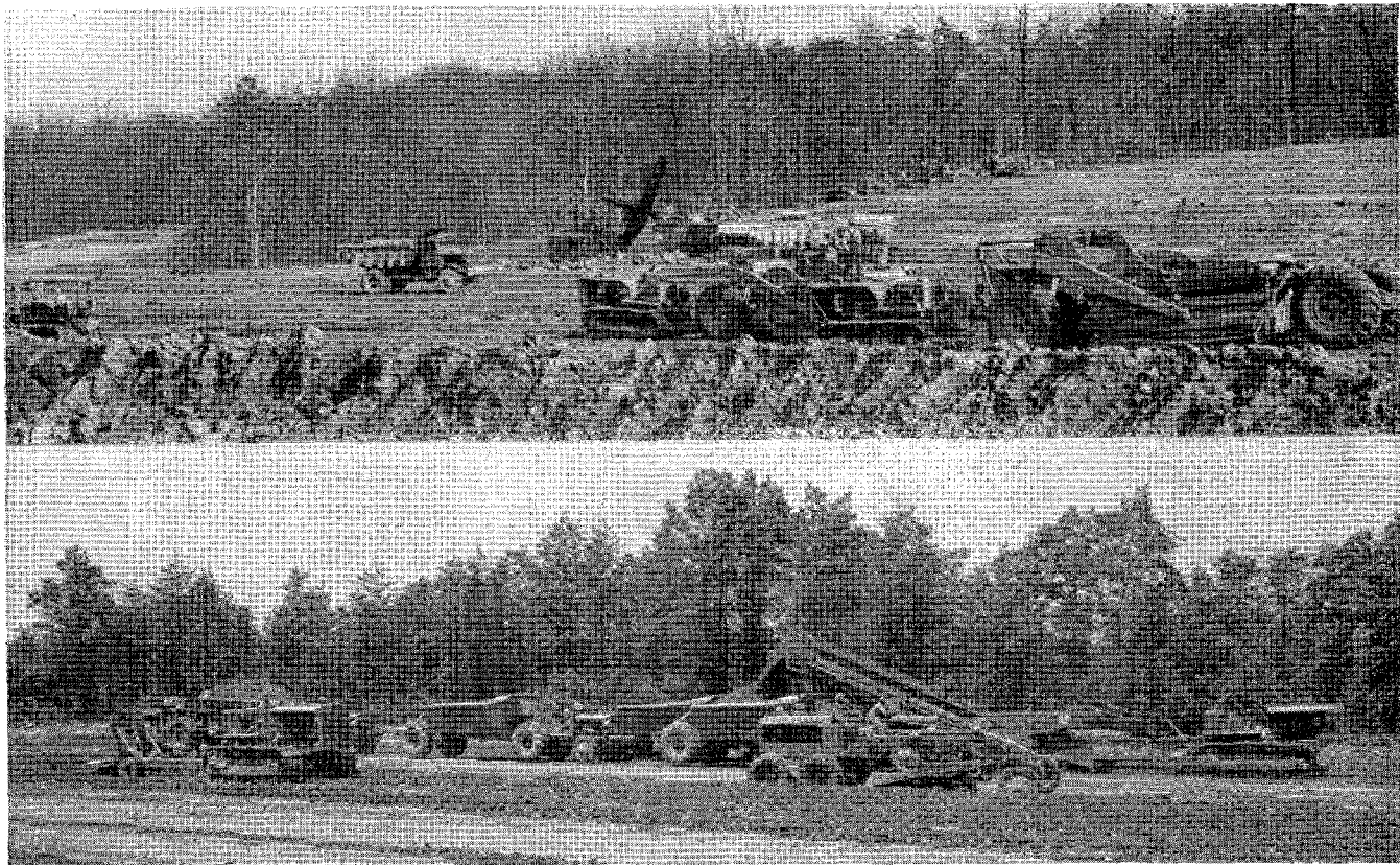
Typical mechanized grading jobs. Above: Tractor-drawn scrapers operate in the foreground while a power shovel loads trucks in the rear. Below: A tractor-towed elevating grader fills wheeled tractor-wagons. In the foreground, a roter (left) and a motor patrol grader (right) aid in the work.
