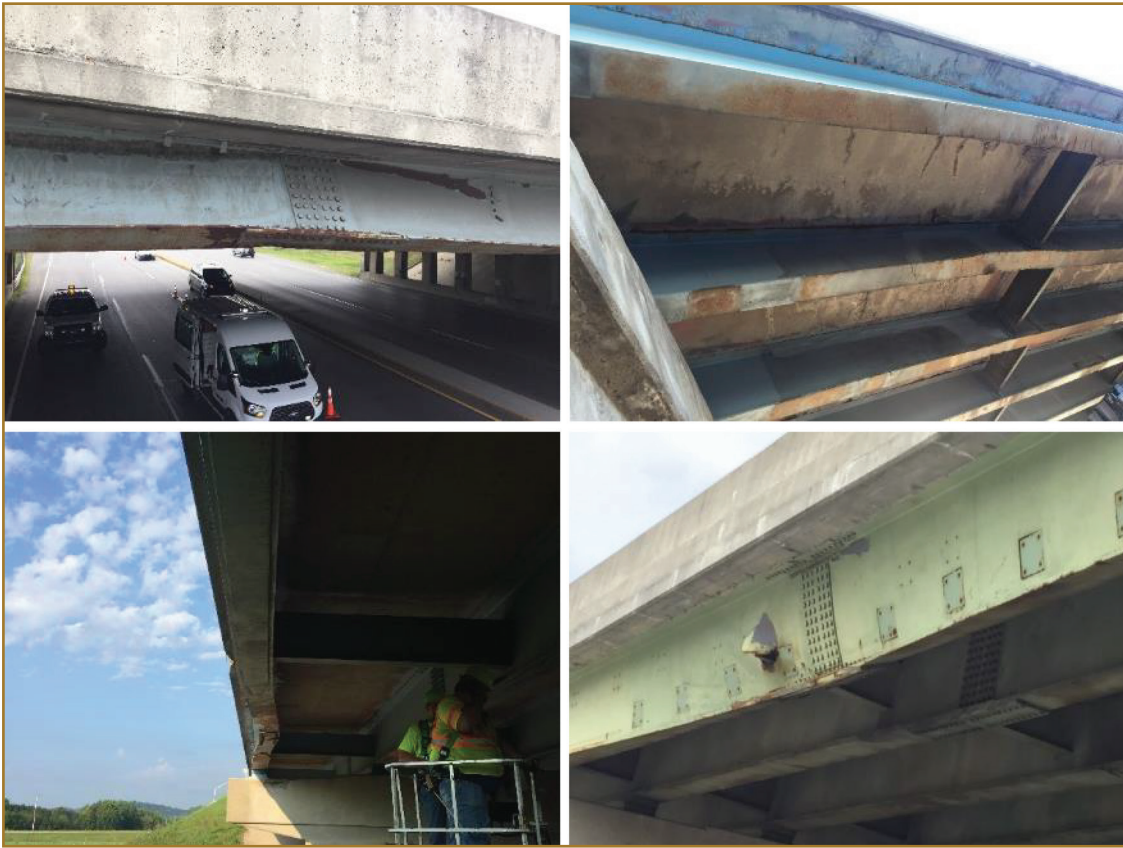
Examples of damage
