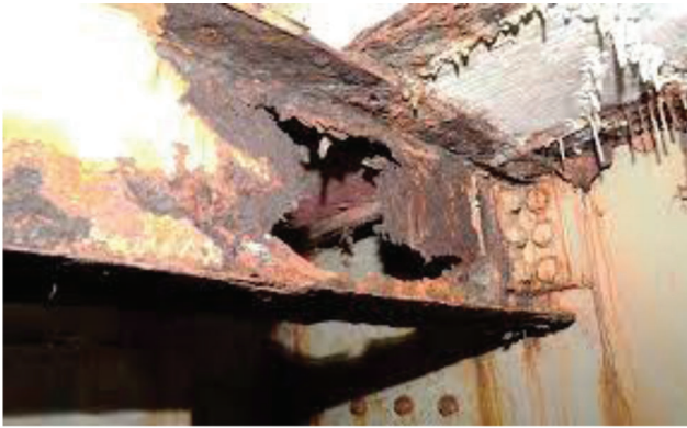
Figure 1.1 Steel bridge coating failure with most of the web thickness lost due to corrosion (NYDOT).
