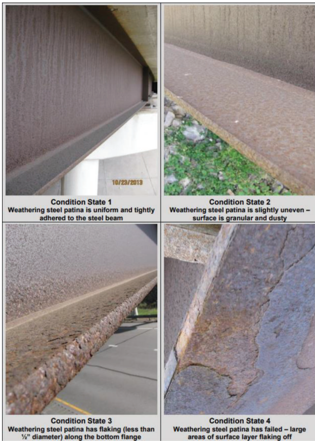
Figure 2.10 Reference images provided by MnDOT for weathering steel condition states (MnDOT, 2021).
