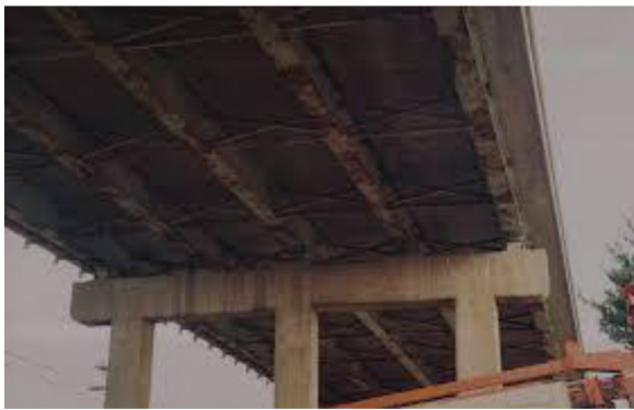
Figure 1.2 Steel bridge coating that is compromised with corrosion visually evident.
