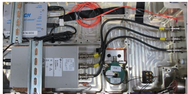
Fig. 13.27. Empty equipment enclosure with oscilloscope, modem, and optical fiber link to a display outside of the airplane.
