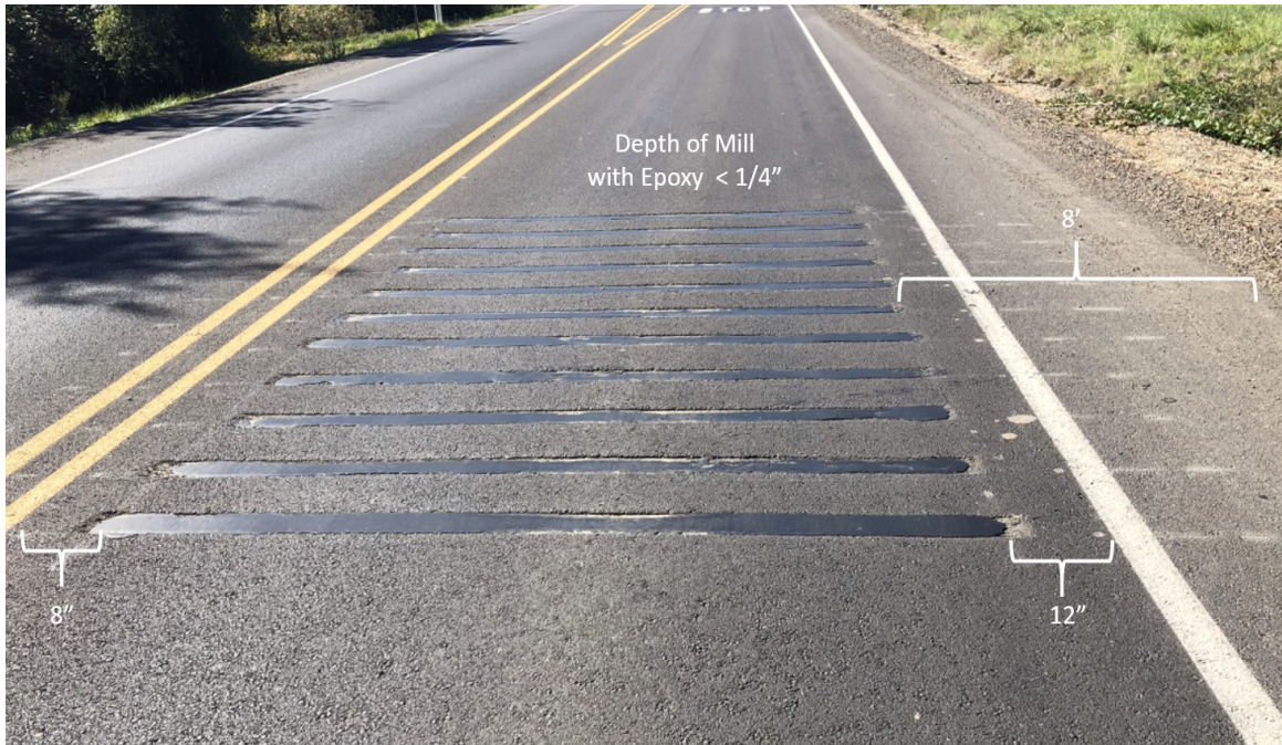
Figure 3.2: After condition: Epoxy filled TRS at near location
