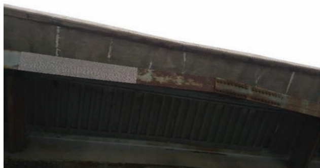
Figure 4.4 Damaged girder of Asset 020-71-04052.
