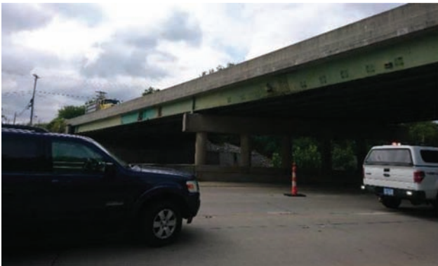
Figure 4.21 Damaged girder of Asset (45)46-53-05993.
