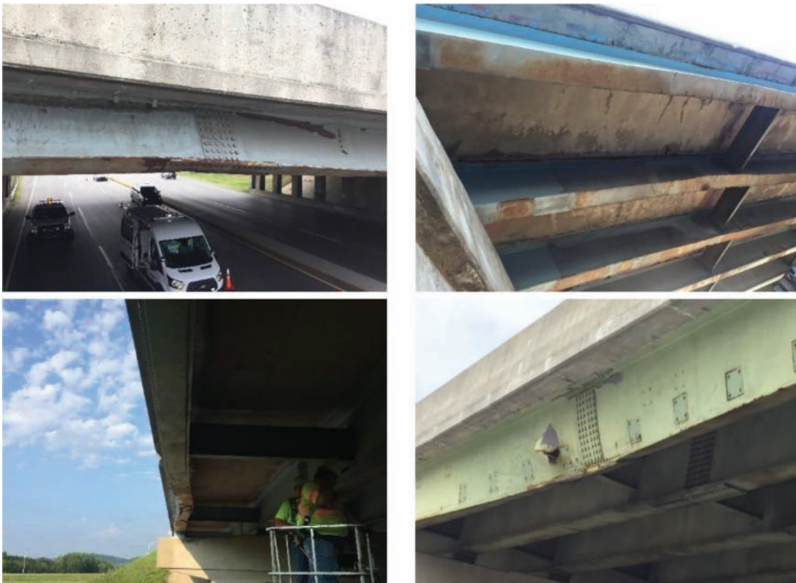
Figure A.1 Examples of damage.
