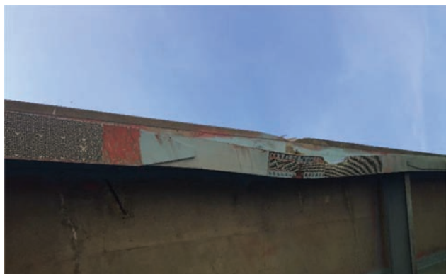
Figure 4.16 Damaged girder of Asset 037-55-05265.
