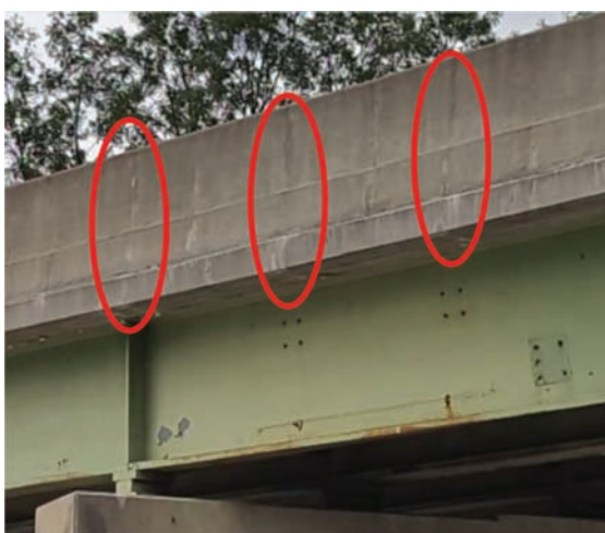
Cracks in Negative Moment Region
