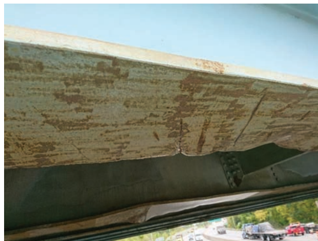
Figure 4.10 1st and 2nd damaged girder from West of Asset 030-02-04803.
