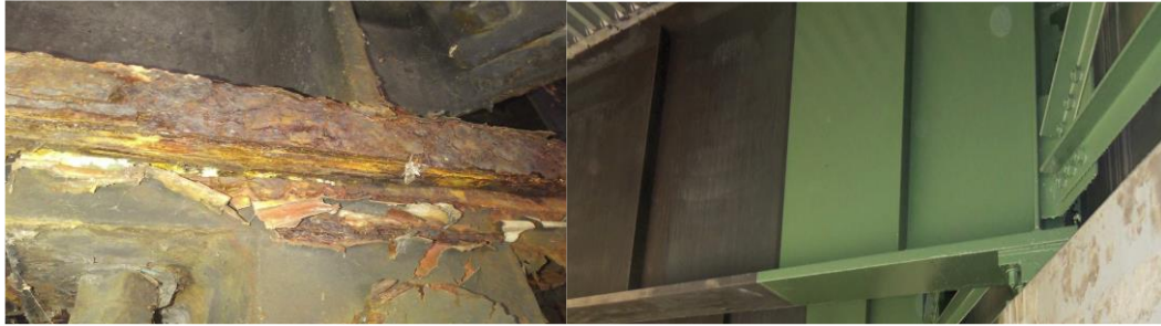
Figure 1. An Over-coated beam: US Route 202 over NJ Route 29 before and after Over-coating
