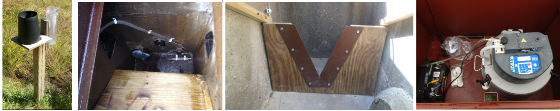
Figure 3. Monitoring equipment utilized at the PSD monitoring sites. Manual and tipping-bucket rain gauge (left), sample intake and bubbler tubing with wooden awning in foreground in catch basin at SR-59 (second from left), weir installed at SR-49 (second from right), and automated sampler at SR-43 (right).
